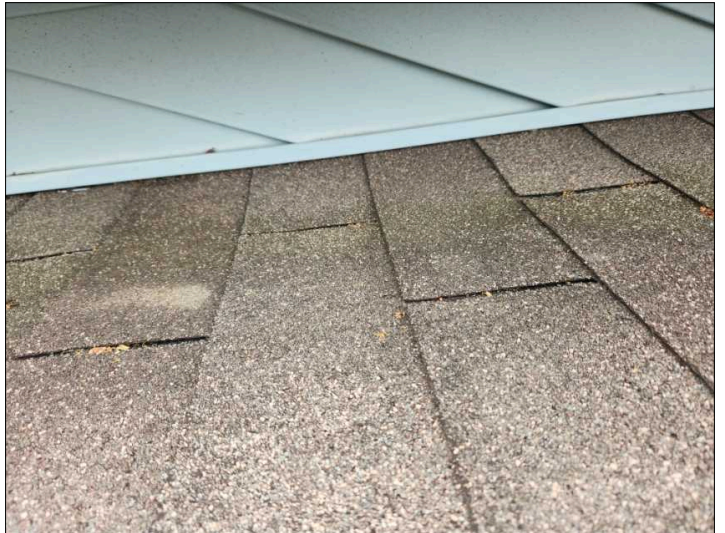
The siding is closer than recommended or in contact with the roof. It is recommended that there be a separation to help prevent water from wicking up into the siding material causing deterioration.
