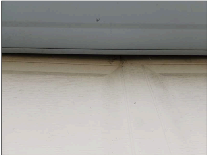
Garage door is dented.
