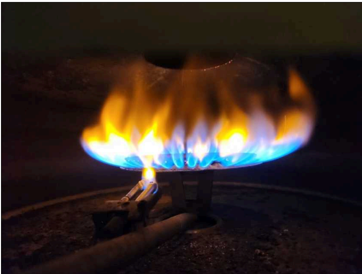
Overview of water heater burner compartment
