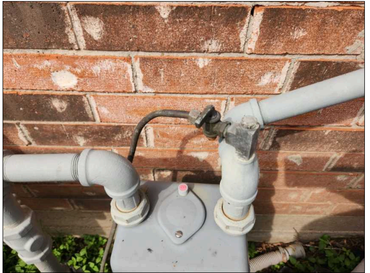
Unapproved gas valves were noted, recommend changing all unapproved gas valves. These valves are designed with a spring at the bottom of the valve which weaken over time causing gas to leak when operated. Although they may not be leaking at the time of inspection they have a high likely hood of leaking when operated. Mainly at - gas meter
