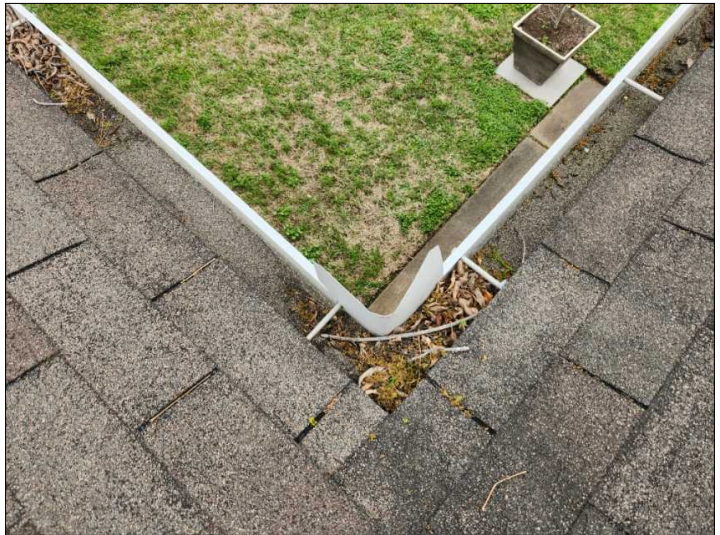
There is debris in the gutters, recommend cleaning gutters to restore to proper operation.
