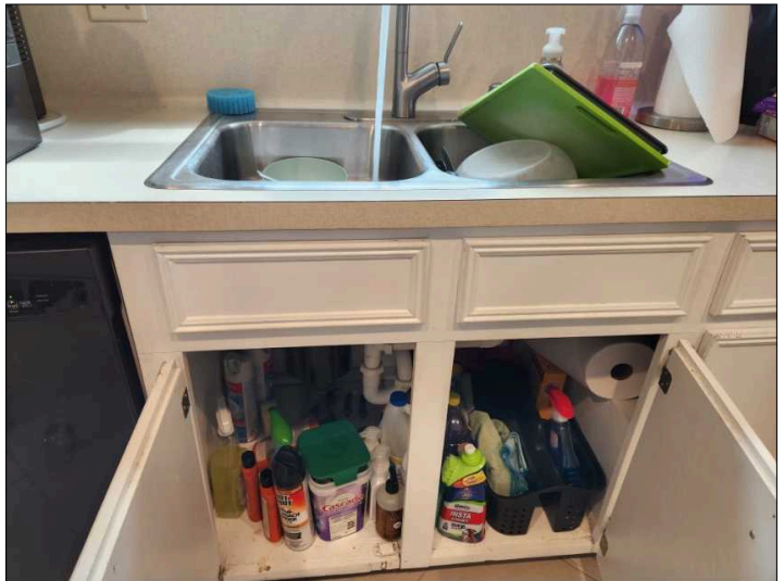
Overview of Plumbing Fixture(s) in Operation.
