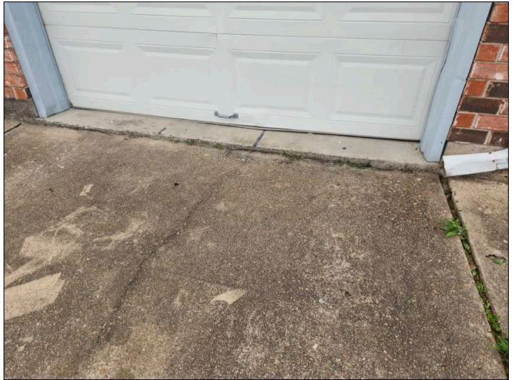
Uneven pavement was noted, recommend repairs to help prevent tripping. Mainly at - driveway
