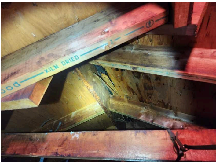
The roof decking was deteriorated, recommend all deteriorated decking be replaced to help prevent further damage and water penetration into home. Mainly at -
