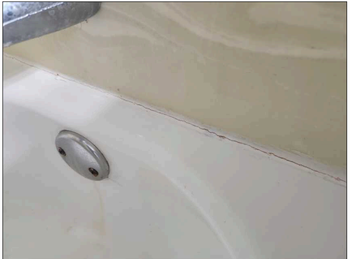
Recommend sealing the tub/shower surround to help prevent water penetration to underlying materials. Mainly at - primary bath
