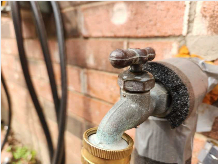
There is a leak at the valve stem on the exterior water faucet, recommend tightening packing nut, adding packing cord or replacing packing if needed. Mainly at - left
