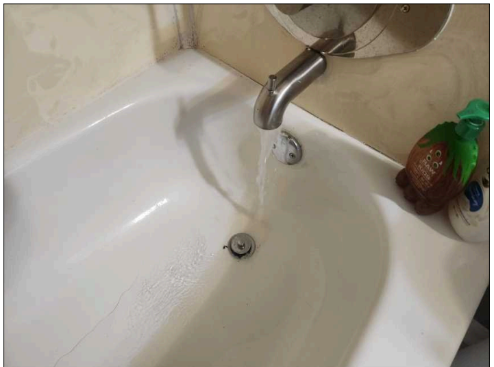
Overview of Plumbing Fixture(s) in Operation.
