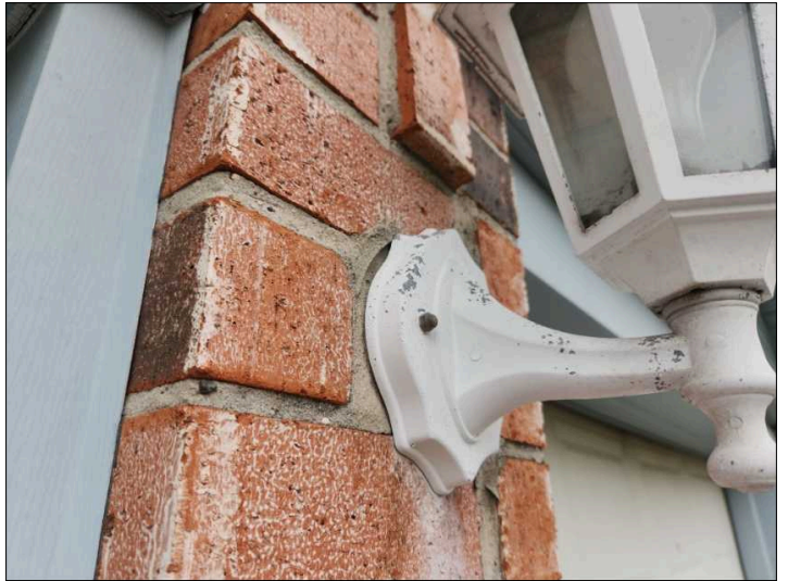
Seal all electrical lighting fixtures at wall connection to help prevent water penetration. It is a good idea to leave a small opening at the bottom to allow any water penetrating to escape.
