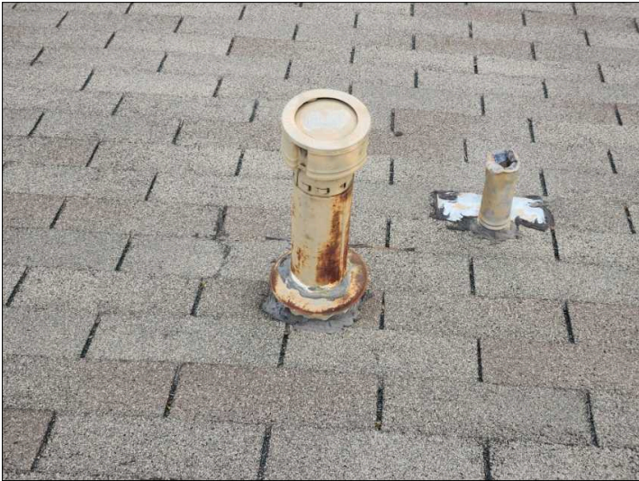
There are signs of rusted vents or flashing on the rooftop. We recommend painting or replacing all rusted or deteriorated vents or flashing as needed.
