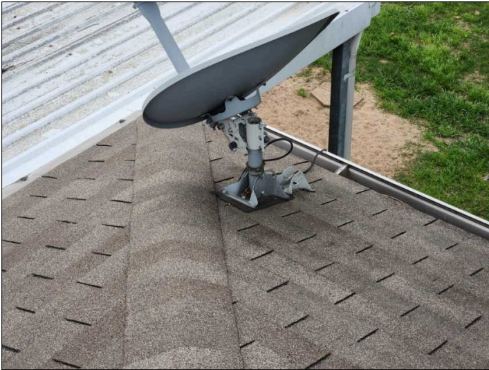
There is/was a satellite dish mounted to the roof structure. It is recommended that the Satellite dish be properly mounted at the siding of the home or on a stand-alone base in the yard. Recommend sealing the mounting hardware to help prevent water penetration.
