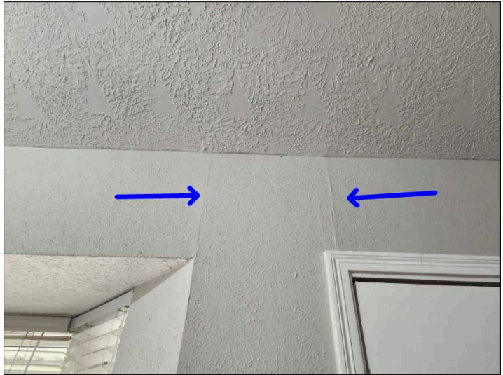
Settlement cracks were noted at the tape joint in the drywall. Mainly at - dining room
