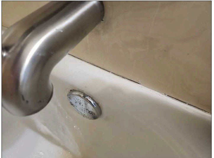
Recommend sealing the tub/shower surround to help prevent water penetration to underlying materials. Mainly at - hall bath
