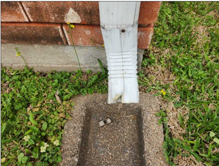
The 90 on the downspout was damaged. Mainly at - front
