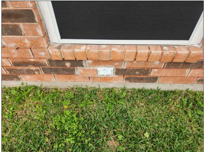
Recommend replacing all wet area exterior receptacle covers with the code approved bubble style cover.
