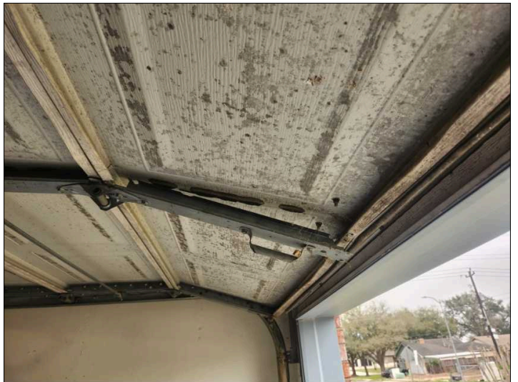
Garage door hardware is loose.
