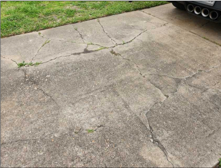
Cracks were noted in the pavement. The pavement is unlevel and can be a tripping hazard if not corrected, recommend repairs. Mainly at - driveway
