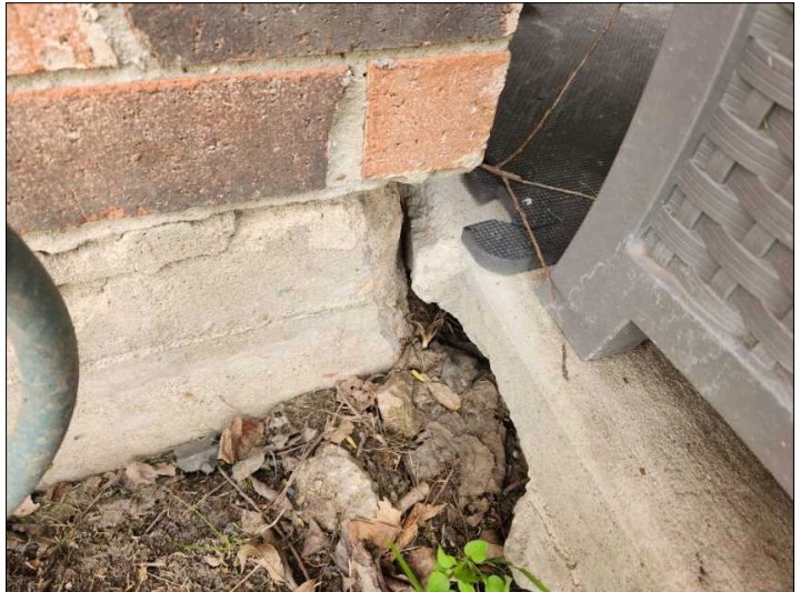
Corner chips or breaks were noted on the corner(s) of the foundation. These are usually considered cosmetic in nature unless other movement is noted. Recommend patching or repairing to help support corner above. Mainly at - rear
