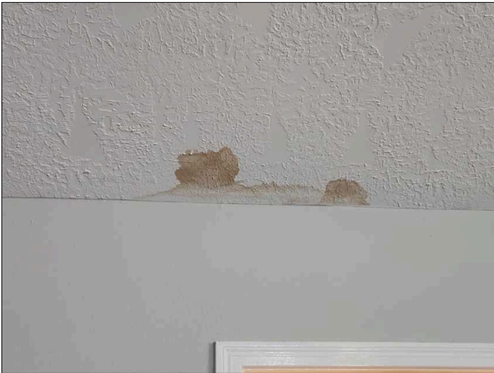
There are indications of water penetration to the ceiling evident mainly by staining. Unable to determine condition of the underlying materials. Mainly at - living room
