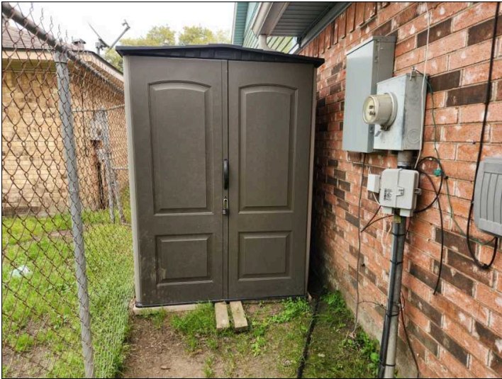
Wood or other debris is stacked against the house. Recommend all wood or other materials be separated from the structure to help prevent conducive conditions for wood destroying insects.
