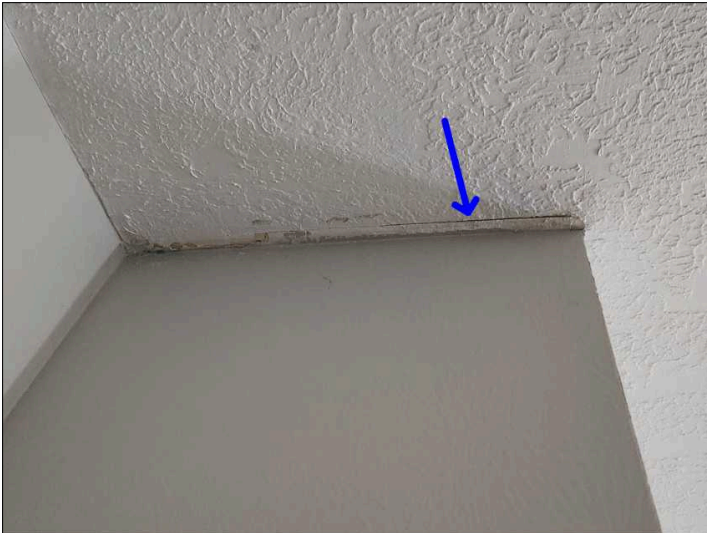
Settlement cracks were noted at the corner bead/tape joint in the drywall. Mainly at - living room
