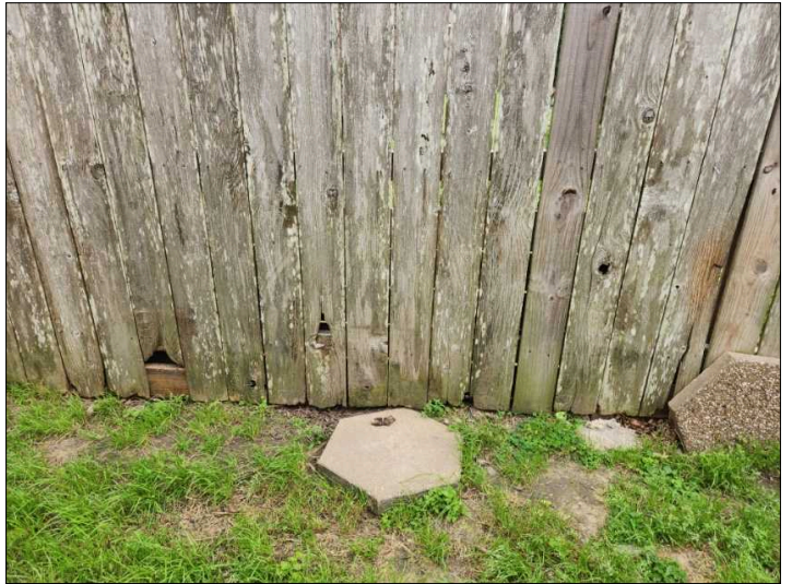
Although fences are not inspected it was noted that the fence is showing some signs of damage or deterioration.
