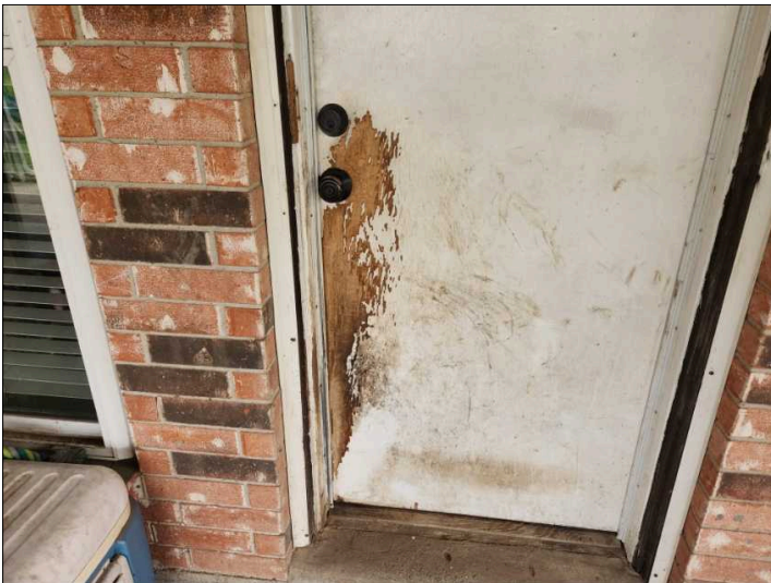
There is pet damage on the door. Mainly at - back door
