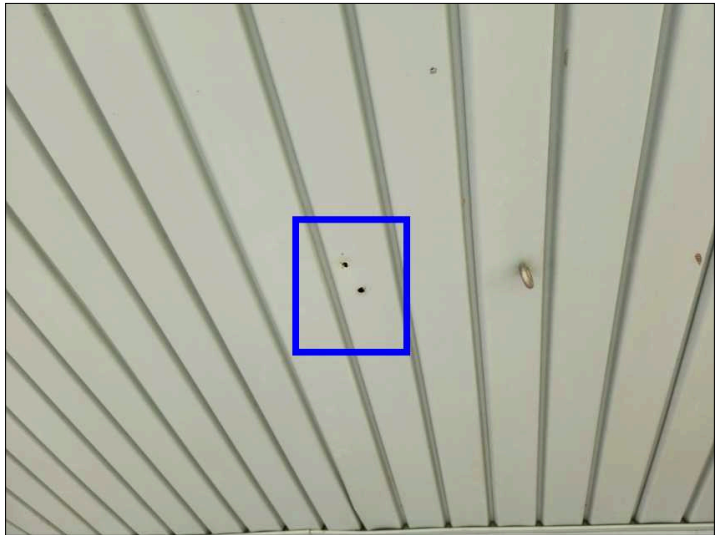
Seal gaps and holes in soffit to help prevent water penetration and rodent intrusion. Mainly at - front patio
