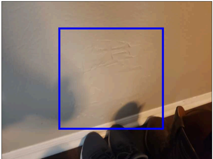
There is evidence of previous patch work and or painting on the interior finishes. Recommend contacting homeowner for more information. Mainly at - primary bedroom
