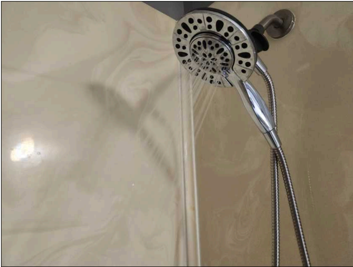
Overview of Plumbing Fixture(s) in Operation.
