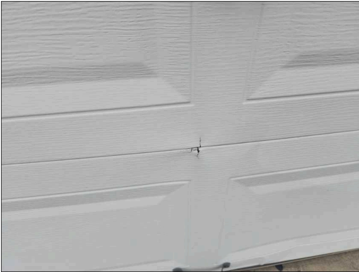
Garage door is cracked or split.
