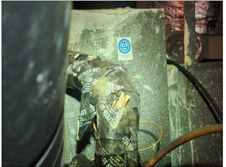
The insulation on the A/C condensation or low pressure refrigerant line is missing at the evaporator unit. Recommend insulating to prevent moisture damage to ceiling surfaces.
