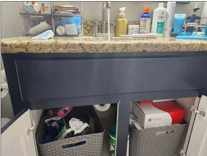
Overview of Plumbing Fixture(s) in Operation.
