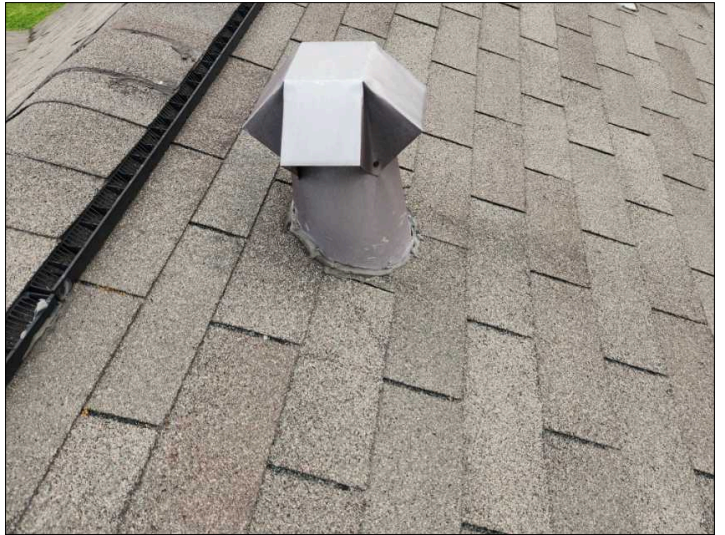
Improperly installed vent flashing
