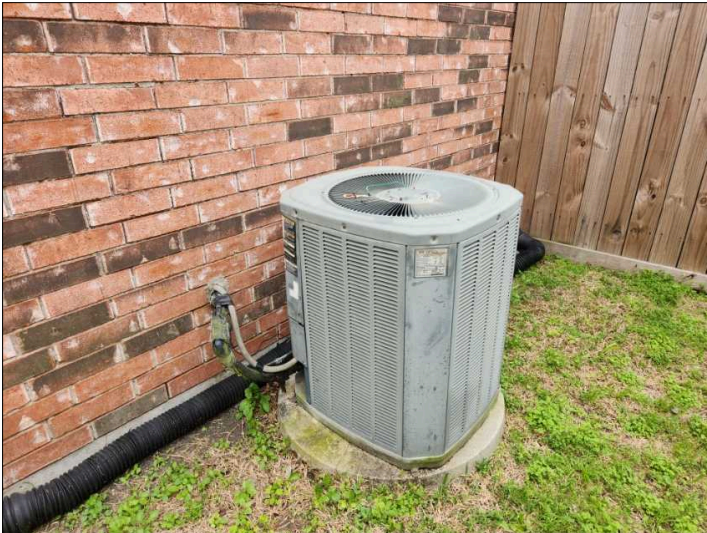
Overview of A/C Condenser
