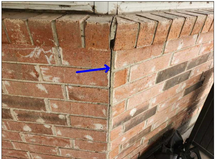
Settlement cracks were noted in the brickwork. Mainly at - rear
