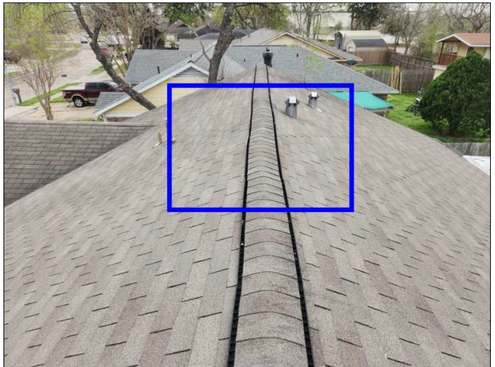
There are indications that there is deteriorated decking under the roof covering due to a soft spot under the shingles, recommend contacting a roof specialist to evaluate and repair as needed and check entire roof for other issues that may be of concern.
