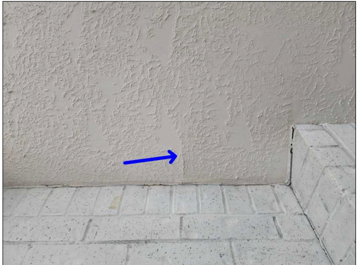
Settlement cracks were noted in the drywall. These are generally considered cosmetic only, unless otherwise noted. Mainly at - living room
