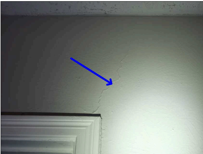
Settlement cracks were noted in the drywall. Mainly at - primary bedroom
