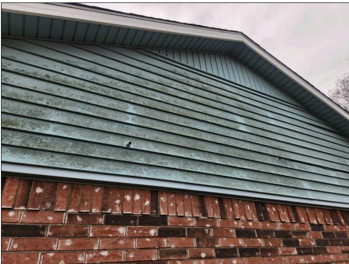
There are signs of growth on exterior brickwork/siding, recommend cleaning to help prevent deterioration.
