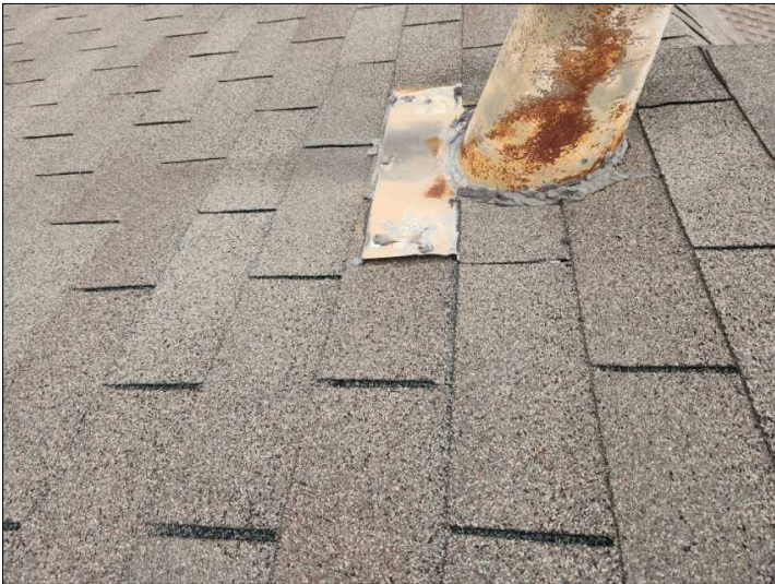
The roof flashing is lifted. Recommend securing all loose or lifted flashing and sealing nails to help prevent water penetration.
