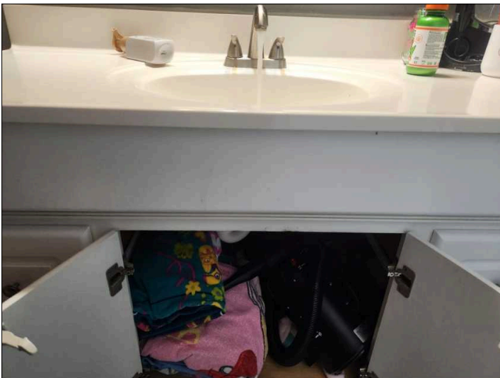
Overview of Plumbing Fixture(s) in Operation.
