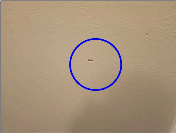
There is damage to the drywall, recommend repairs as needed. Mainly at - front entryway
