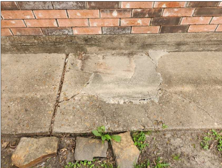
There are indications of previous foundation repair. We recommend you refer to the structural engineer's report if available for further information of repairs, warranty and proper maintenance of the foundation. There is often a transferable warranty after work has been completed, recommend contacting the homeowner for more information.
