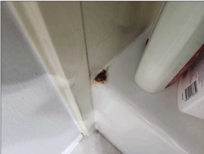
Rust has been noted in the tub, recommend repairs to help prevent deterioration. Mainly at - primary bath
