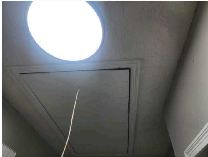
The attic pull-down stairs do not close properly, allowing conditioned air to be lost into the attic or attic air into conditioned space of the home.
