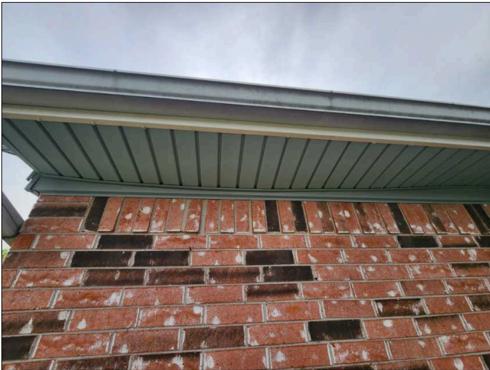
There is loose soffit material at the eave, recommend securing to help prevent damage and water penetration. Mainly at - front
