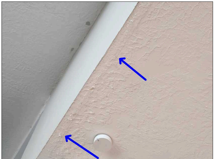
Settlement cracks were noted at the corner bead/tape joint in the drywall. Mainly at - kitchen
