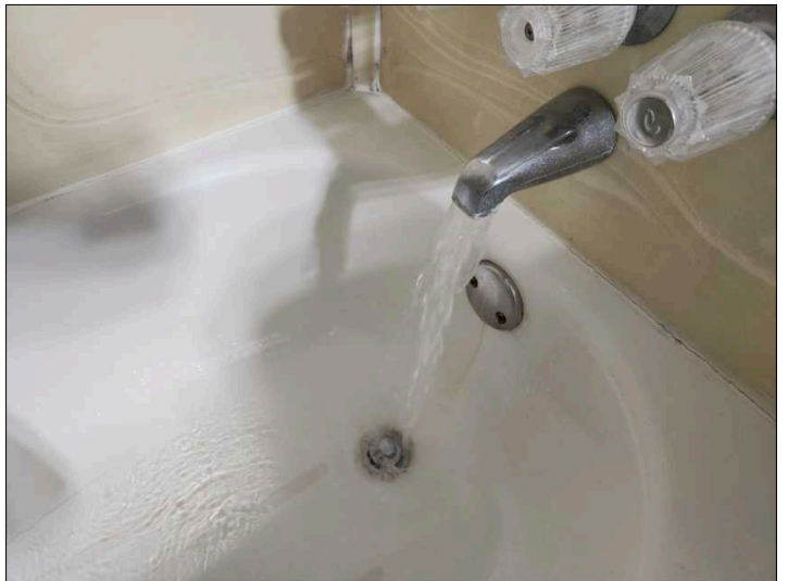
Overview of Plumbing Fixture(s) in Operation.
