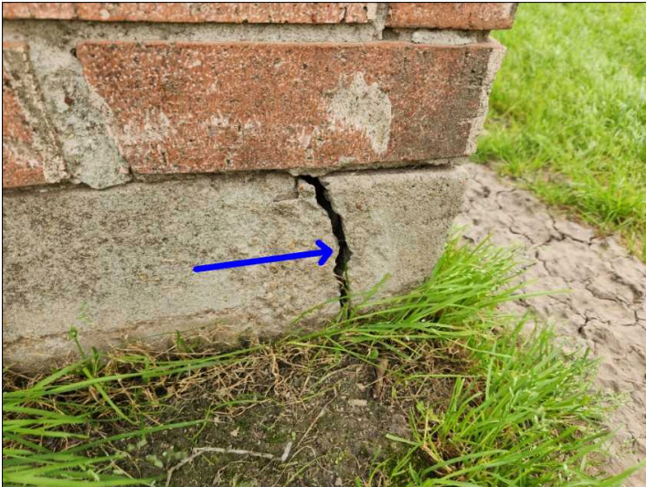
Corner pops were noted on one or more corners of the foundation. These are usually considered cosmetic in nature unless other movement is noted. Recommend sealing all cracks to help prevent further deterioration.
