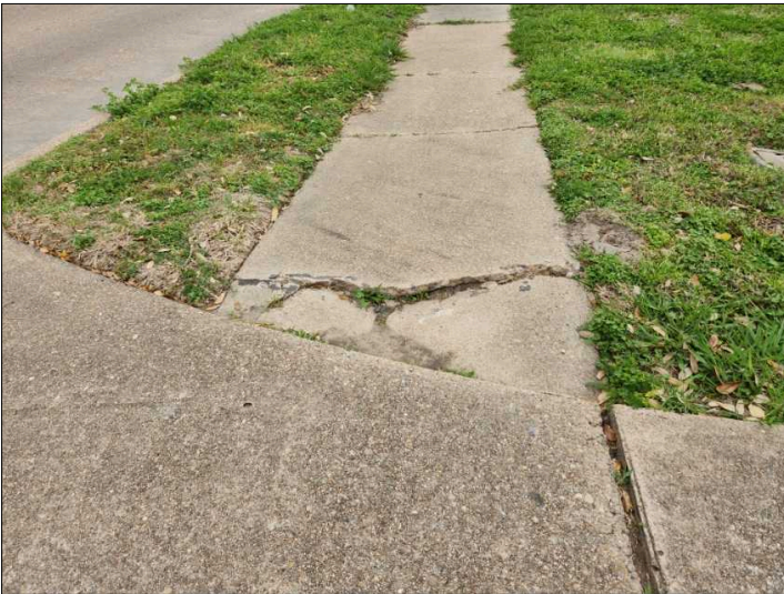
Cracks were noted in the pavement. The pavement is unlevel and can be a tripping hazard if not corrected, recommend repairs. Mainly at - sidewalk
