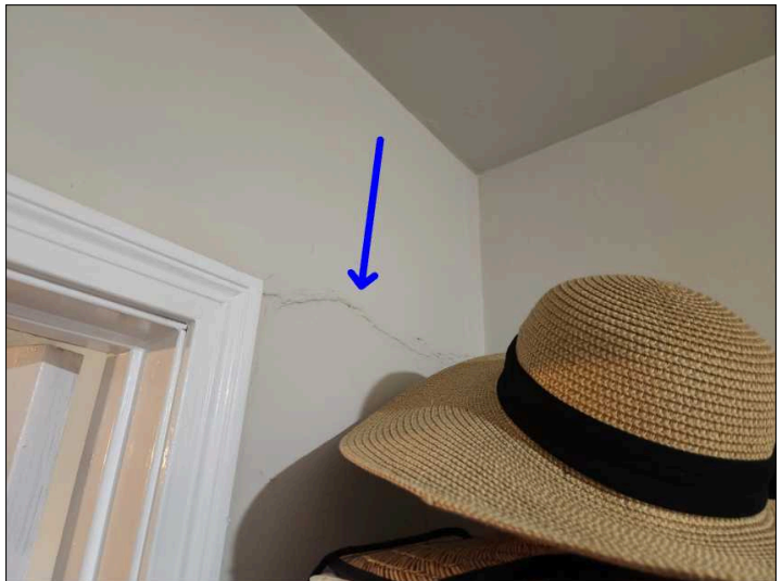
Settlement cracks were noted in the drywall. Mainly at - primary closet
