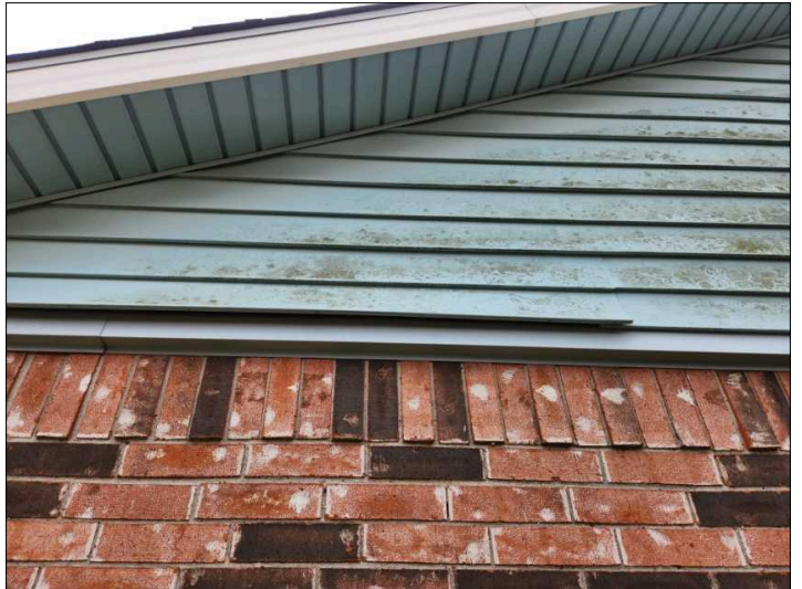
There is loose siding on the home, recommend securing all loose siding to help prevent damaged and water penetration. Mainly at - right
