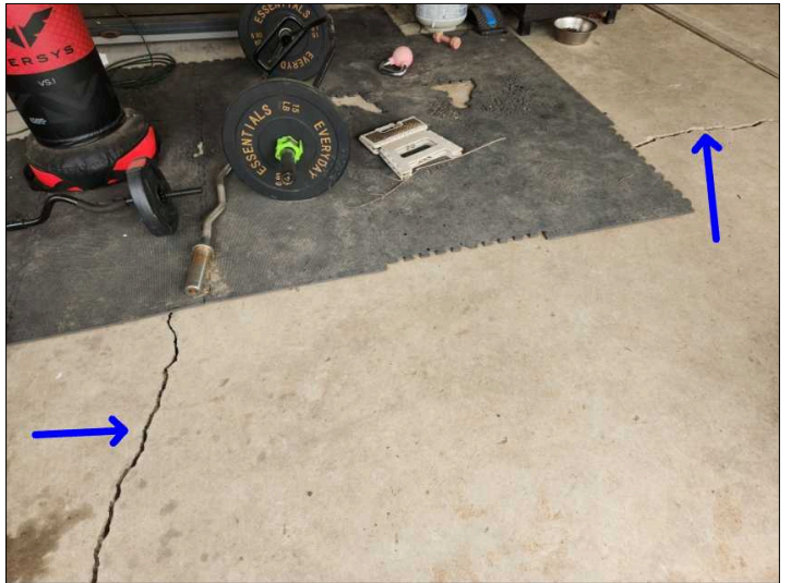
Cracks were noted in the pavement. The pavement is unlevel and can be a tripping hazard if not corrected, recommend repairs. Mainly at - back patio
