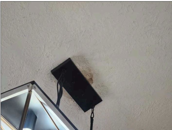
There is damage to the drywall, recommend repairs as needed. Mainly at - dining room
