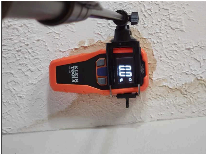
Checked water stain with a moisture meter and found it to be at a normal level. Unable to determine condition of the underlying materials. Mainly at - living room
