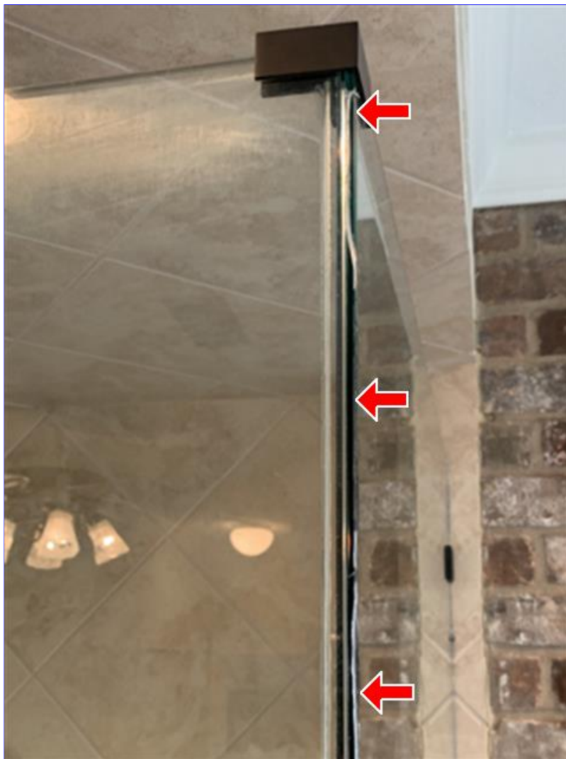
H. Photo 3(Picture) In the master bathroom, the shower glass is loose at the corner and has shifted towards the glass door. Recommend correction.
