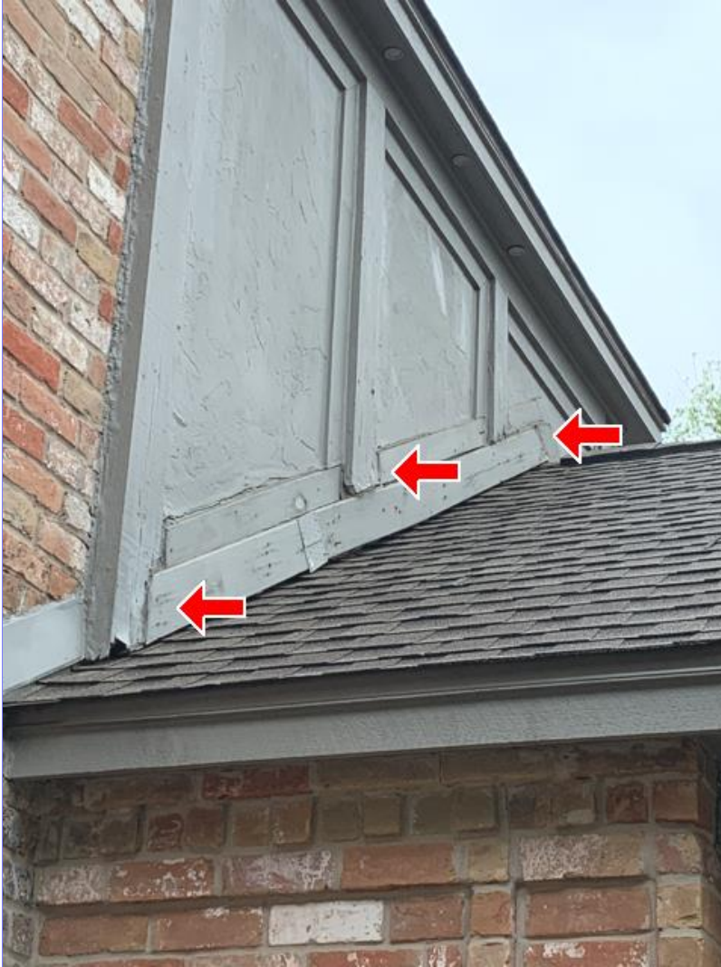
E. Photo 5(Picture) Wood rot was observed on the wood above the Porte Cochere on the left.
