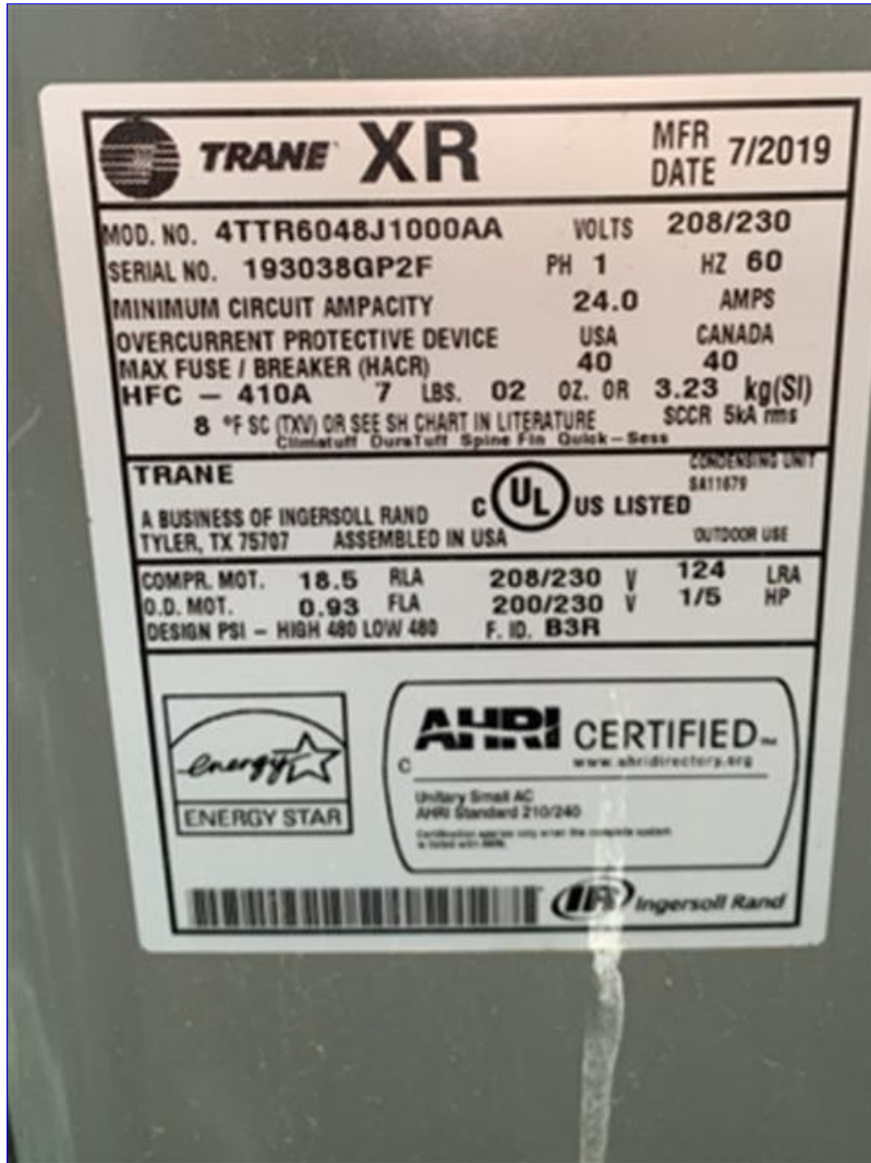
B. Photo 1(Picture) Air conditioner service tag.
