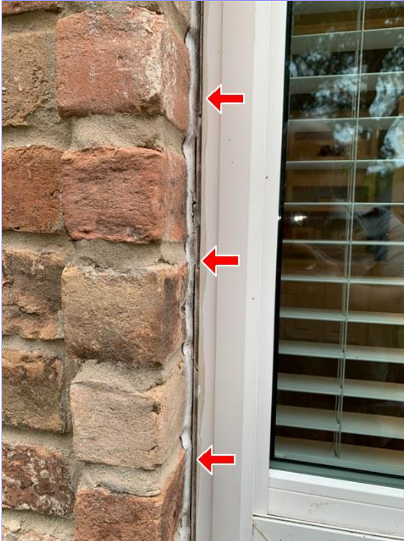
H. Photo 1(Picture) The perimeter sealant, has failed on some windows.
