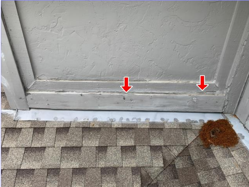
E. Photo 8(Picture) Wood rot was observed in areas of the siding and trim on the upper back side of the house.
