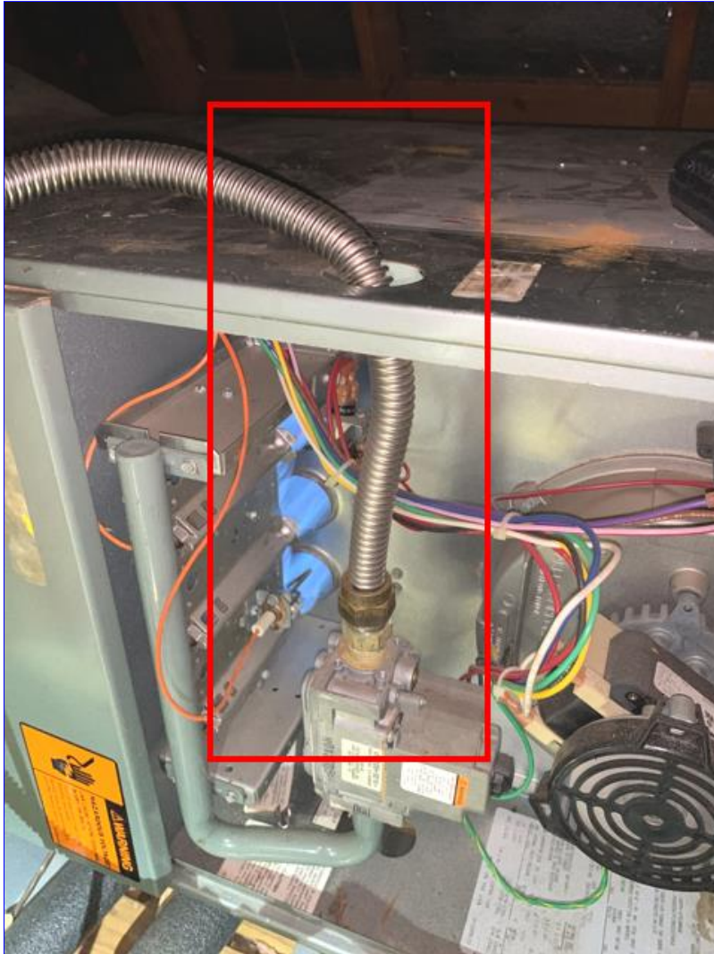
A. Photo 5(Picture) The flexible gas appliance hose is connected inside the unit. A hard gas line needs to be connected and extended outside the unit for the flexible gas line connection.
