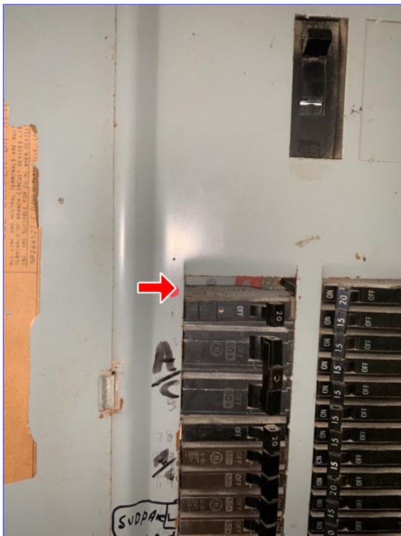
A. Photo 5(Picture) Open breaker knockouts need filler plates installed. Recommend correction.
