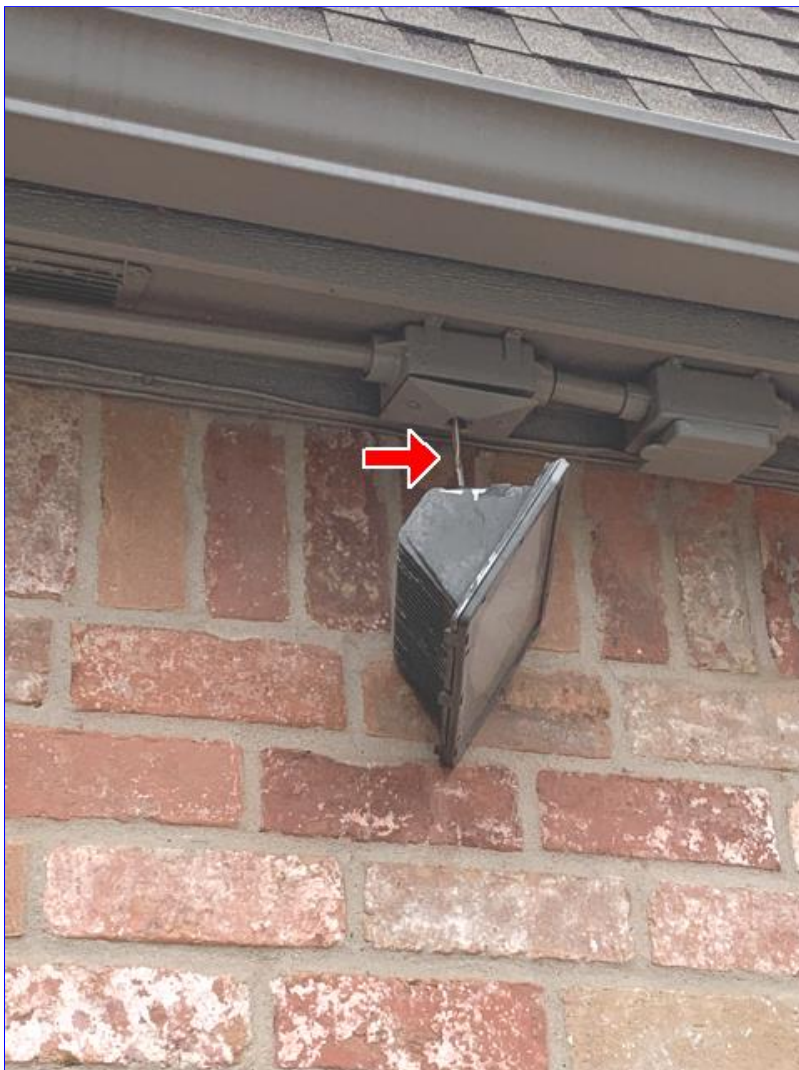
B. Photo 1(Picture) The back porch flood light is damaged and hanging by the electrical wiring.
