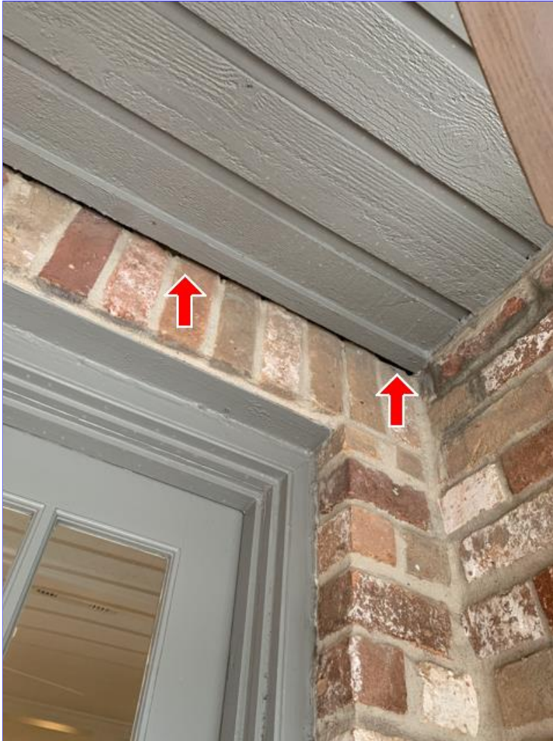
E. Photo 14(Picture) Areas were observed, where the brick, siding and/or trim needs to be resealed.
