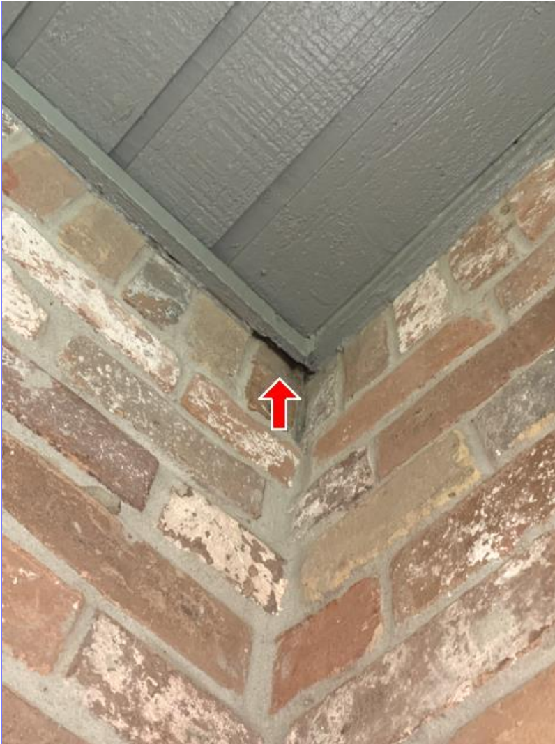
E. Photo 13(Picture) Areas were observed, where the brick, siding and/or trim needs to be resealed.
