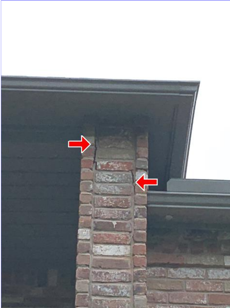
E. Photo 2(Picture) Brick veneer mortar cracks were observed. This condition is cosmetic in nature and not structurally significant. The cracking of the brick veneer is likely due to flexing of the foundation during repeated seasonal changes. The expansive clay soil in the area is prone to excessive swelling during rainy periods and shrinkage during dry periods.
