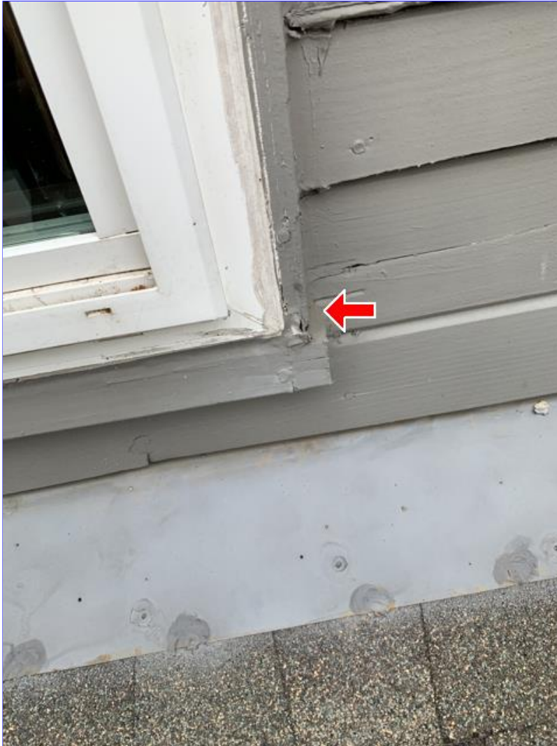
E. Photo 11(Picture) Wood rot was observed in areas of the siding and trim on the upper back side of the house.
