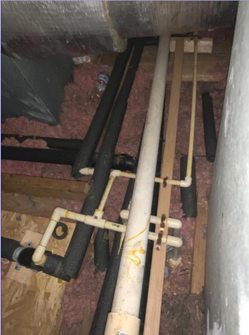
A. Photo 2(Picture) Exposed water pipes observed in the attic space are not properly protected from freezing. Water pipes should be buried under the insulation or properly wrapped to prevent breakage from freezing.
