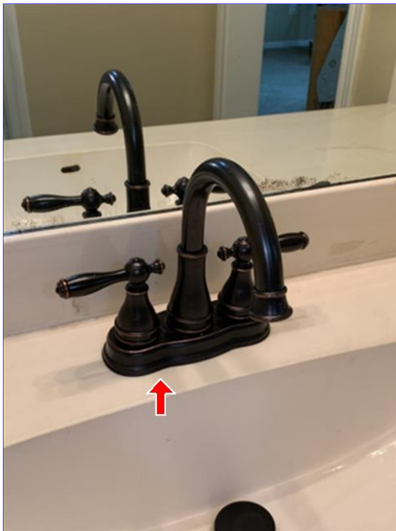
A. Photo 1(Picture) In the upstairs bathroom on the right, one of the sink faucets is loose at the vanity countertop.
