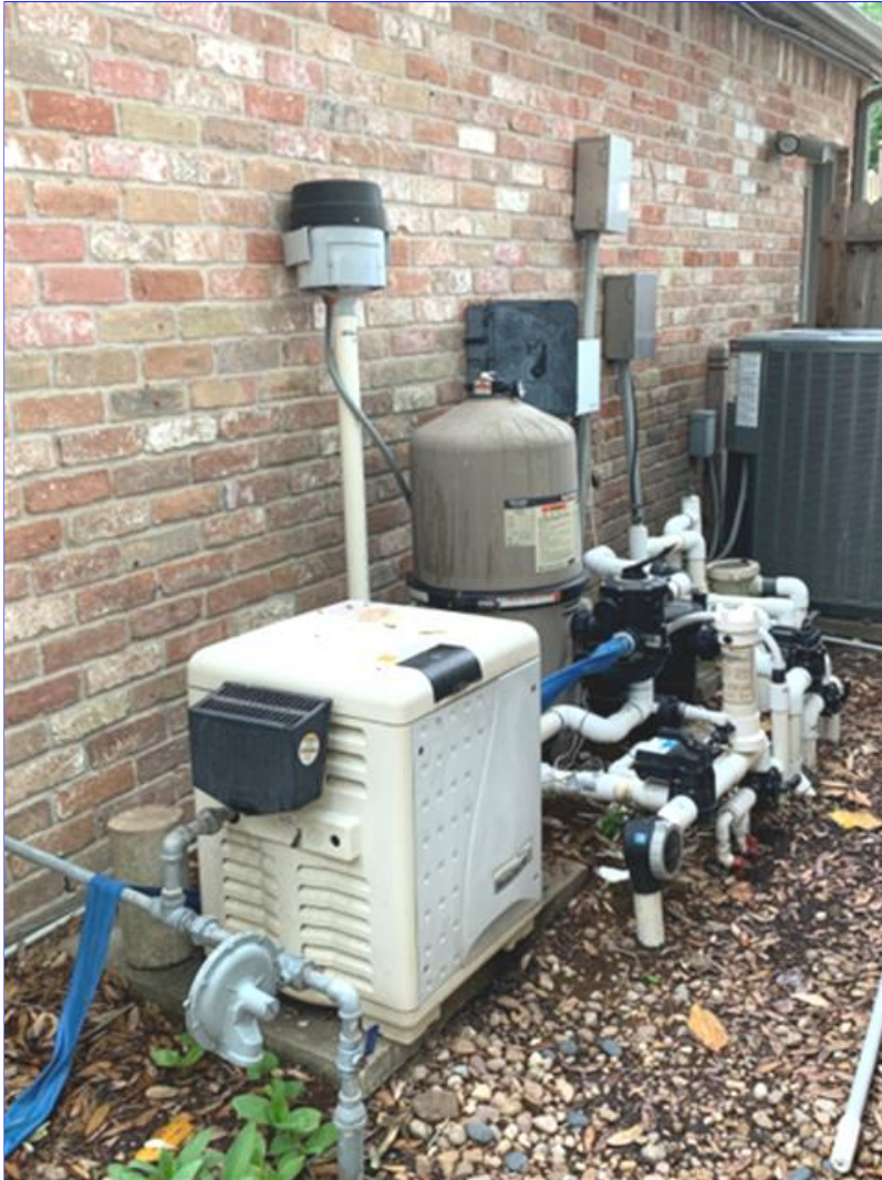
B. Photo 1(Picture) View of the installed pool equipment.
