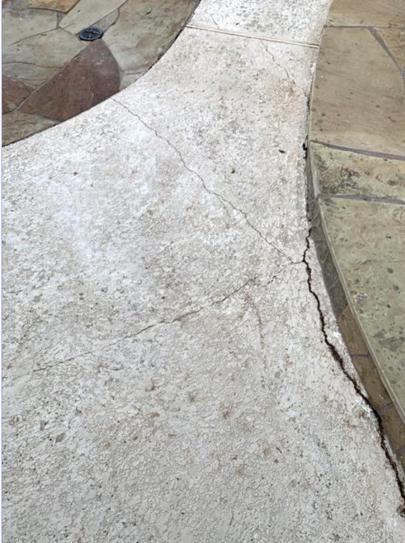
E. Photo 2(Picture) Concrete cracks were observed in the flat work around the pool.
