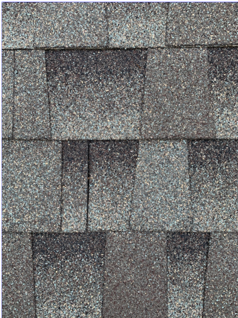
C. Photo 2(Picture) This roof is an Architectural style shingle that will typically last 20 years in this climate.
