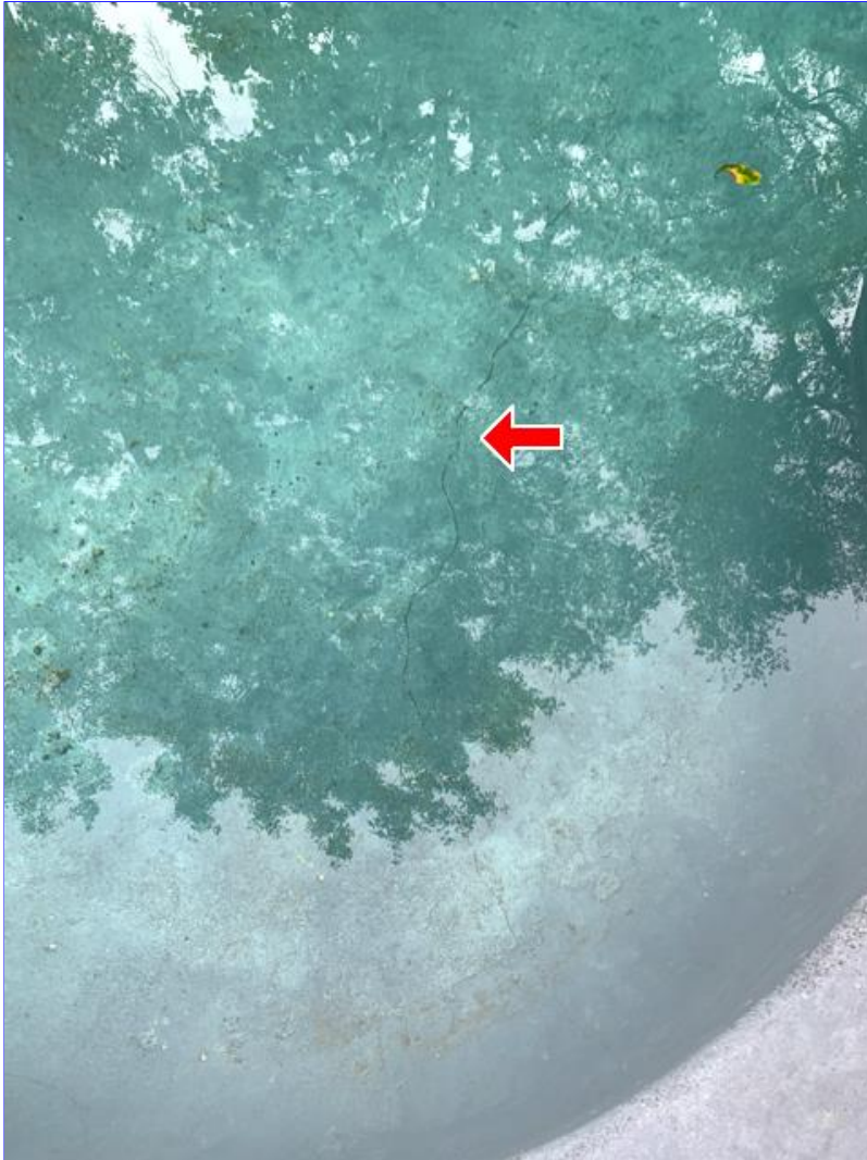
F. Photo 3(Picture) Crack observed in plaster finish. Recommend correction.
