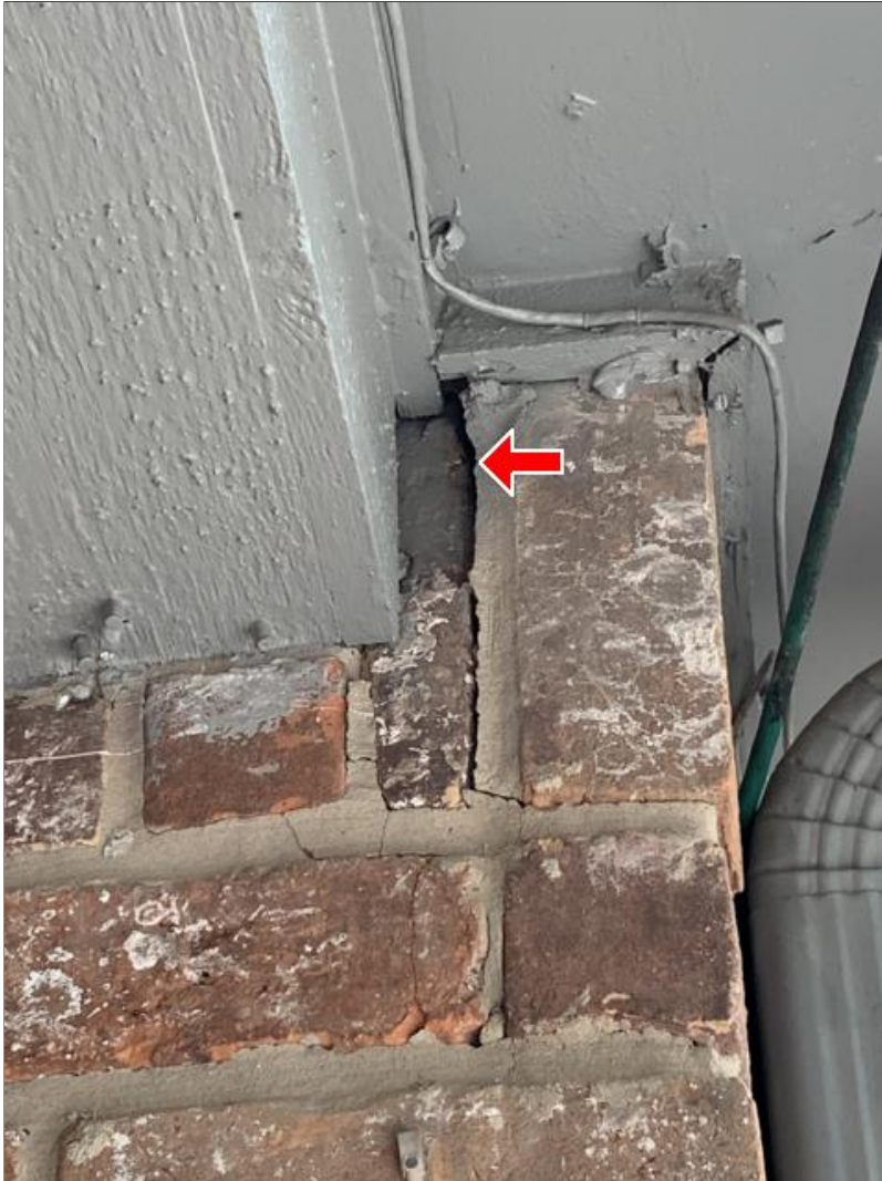
E. Photo 15(Picture) Areas were observed, where the brick, siding and/or trim needs to be resealed.
