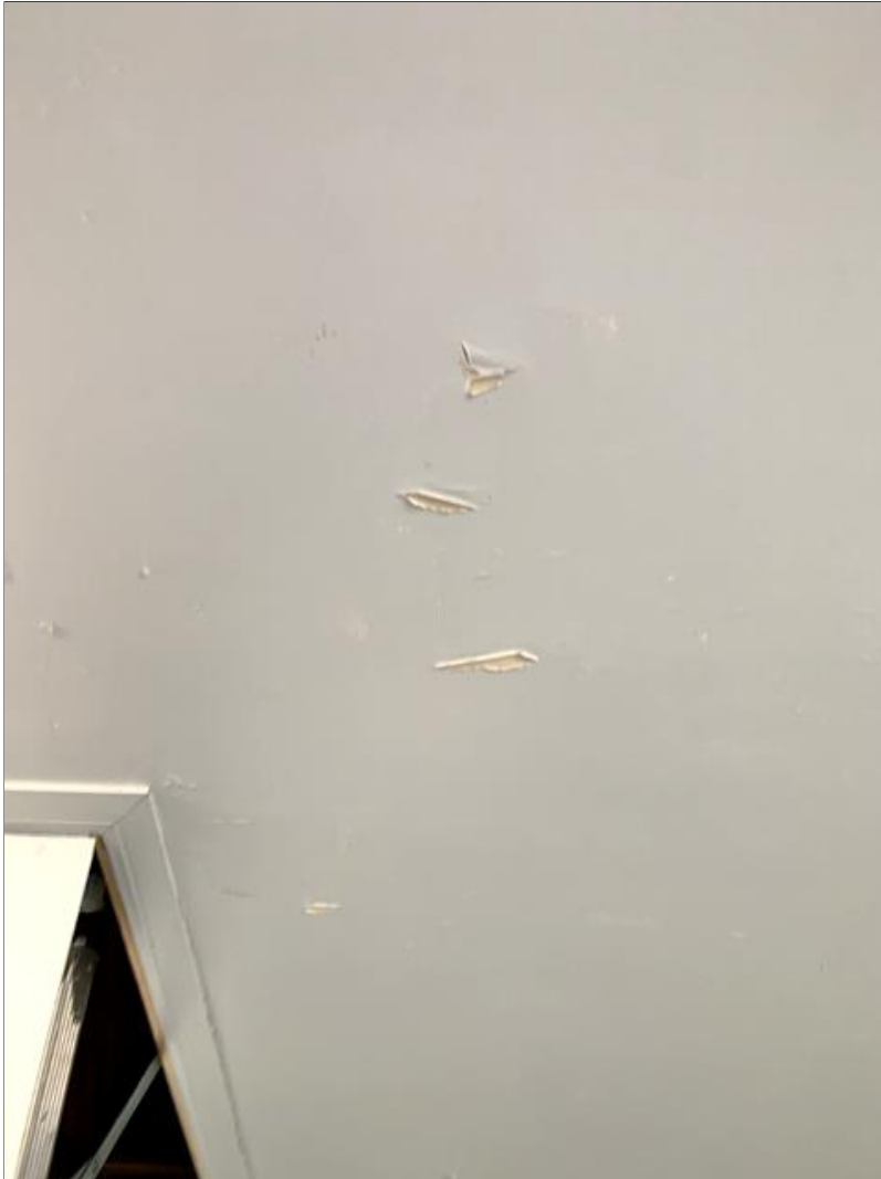
F. Photo 2(Picture) In the garage, areas were observed where are the paint has failed on the ceiling.
