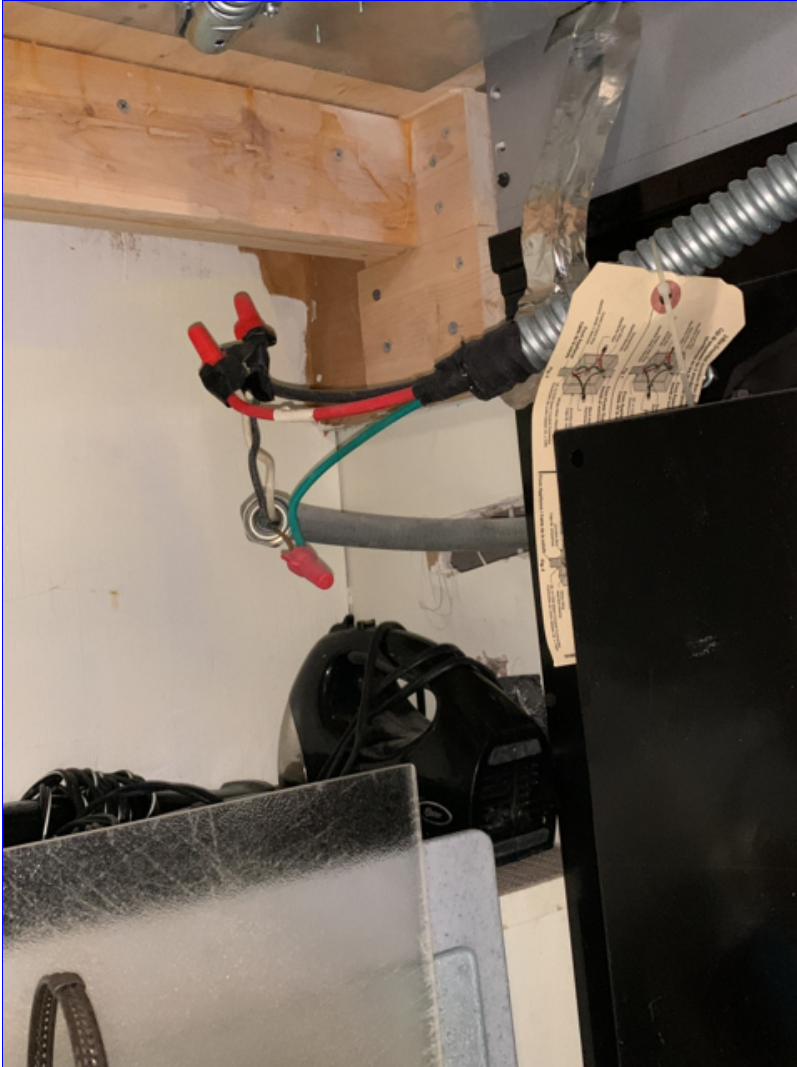
B. Photo 2(Picture) Exposed electrical connections were observed at the kitchen range. Recommend correction for safety purposes.
