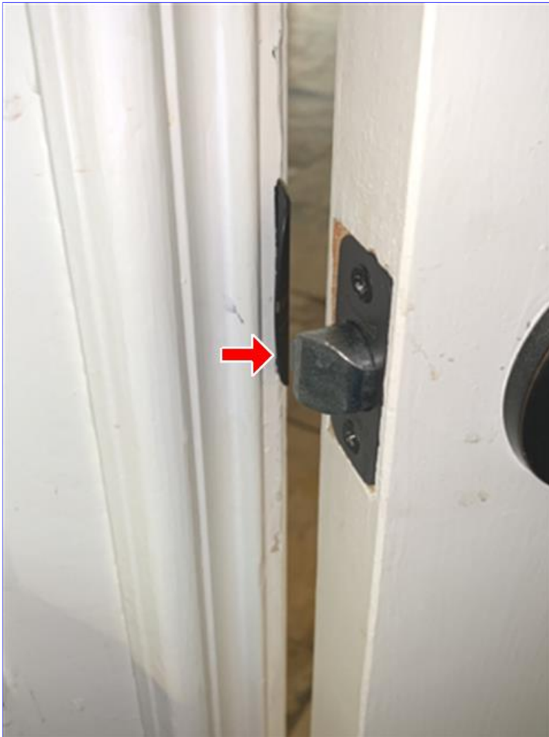
G. Photo 2(Picture) The door hardware at the wet bar location is installed backwards.
