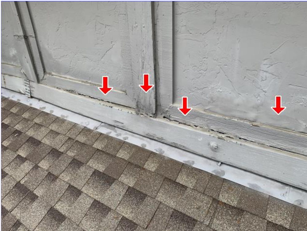
E. Photo 7(Picture) Wood rot was observed in areas of the siding and trim on the upper back side of the house.
