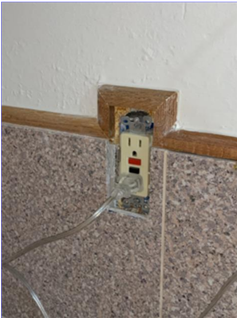
B. Photo 5(Picture) At the wet bar, a missing receptacle cover plate was observed. These plates should be replaced for safety reasons.
