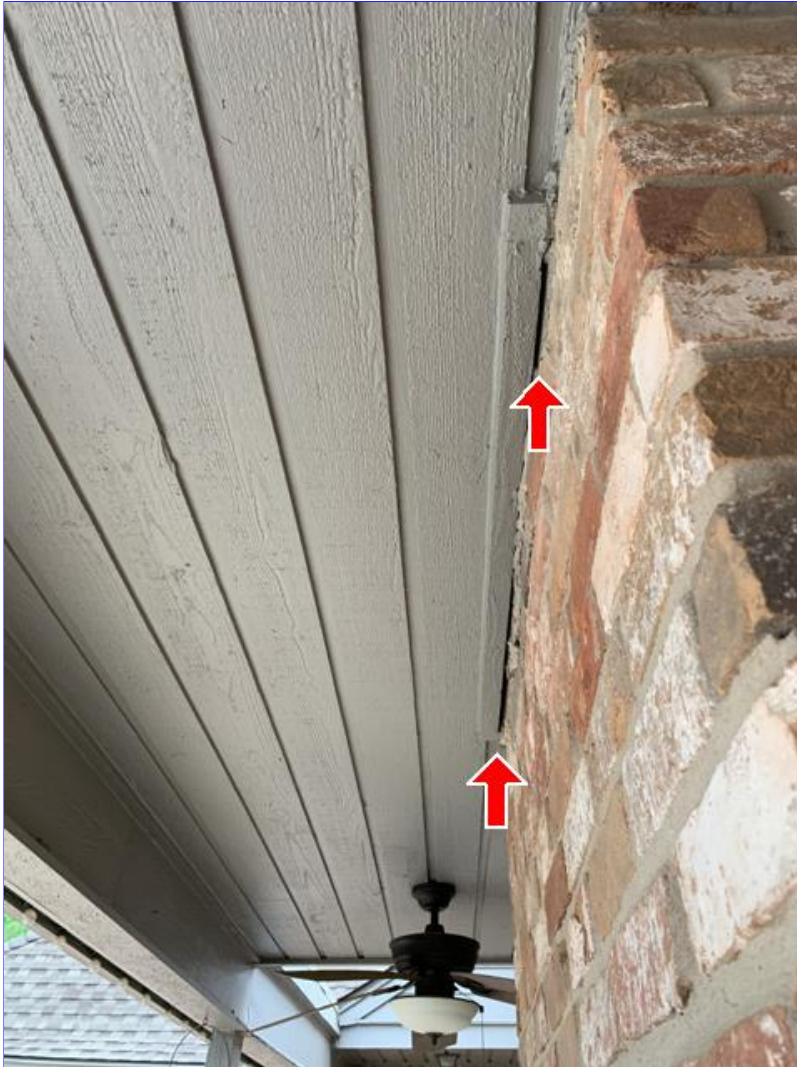
E. Photo 16(Picture) Areas were observed, where the brick, siding and/or trim needs to be resealed.
