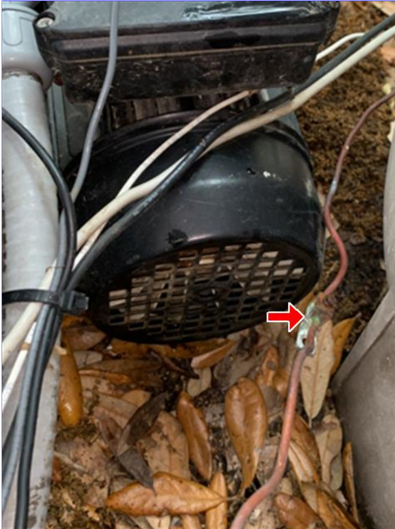
B. Photo 3(Picture) The cleaner pump motor housing and the Pool/ Spa Heater are not bonded to ground. Recommend correction.
