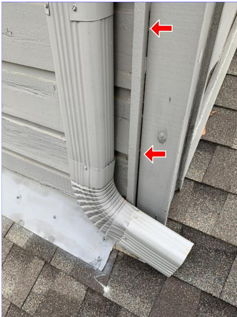
E. Photo 17(Picture) Areas were observed, where the brick, siding and/or trim needs to be resealed.
