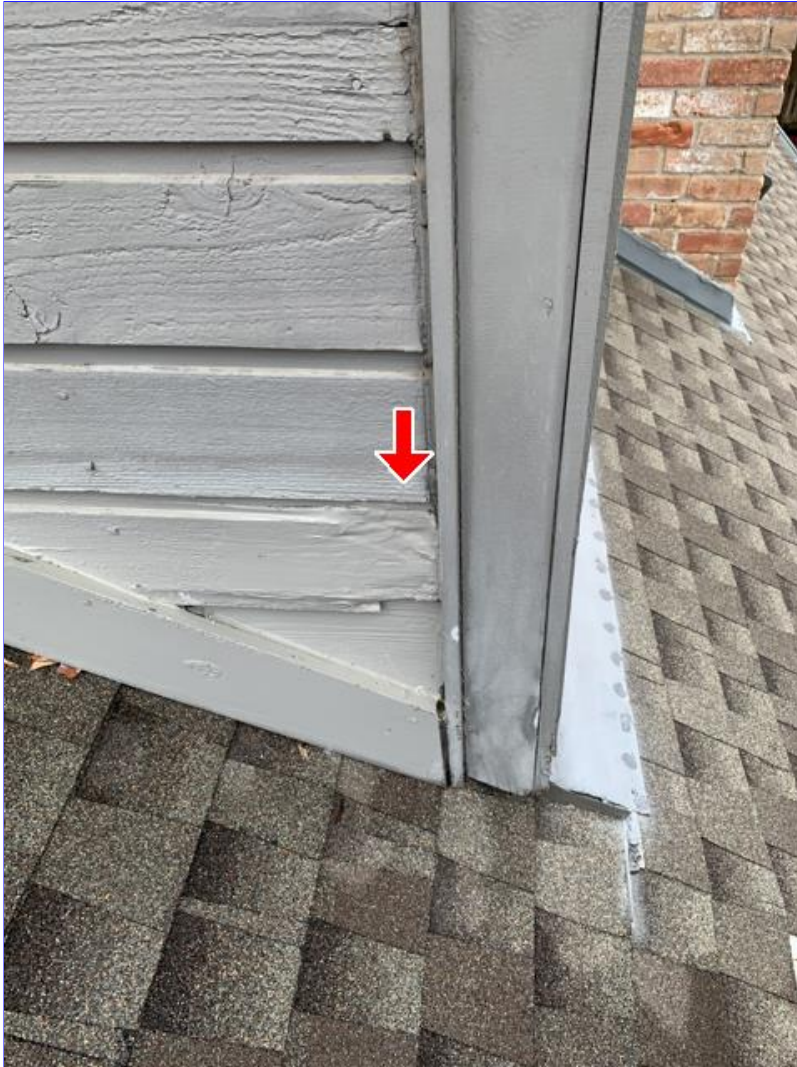
E. Photo 10(Picture) Wood rot was observed in areas of the siding and trim on the upper back side of the house.
