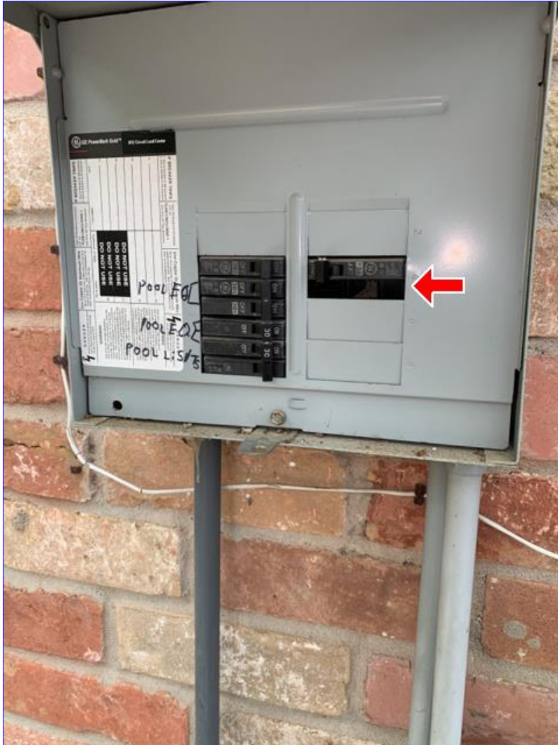
A. Photo 4(Picture) Open breaker knockouts need filler plates installed. Recommend correction.
