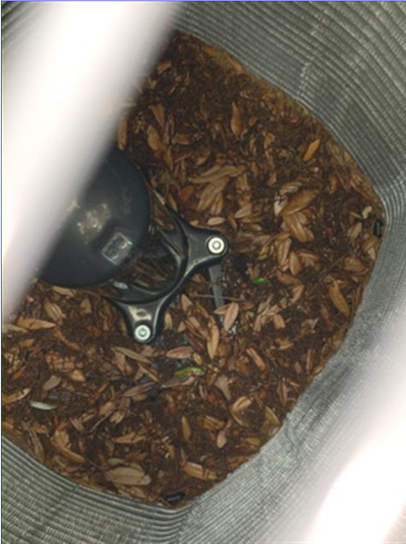
B. Photo 3(Picture) Debris and leaves need to be removed from the inside of the outside air conditioning units.
