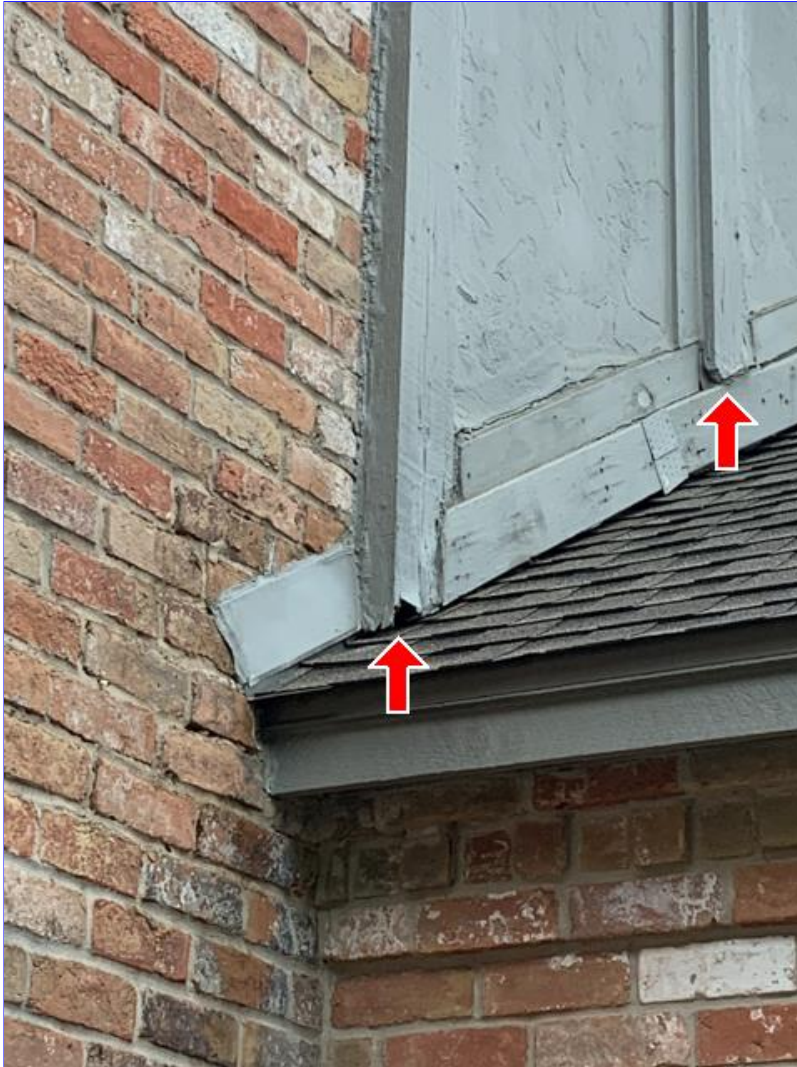
E. Photo 4(Picture) Wood rot was observed on the wood above the Porte Cochere on the left.
