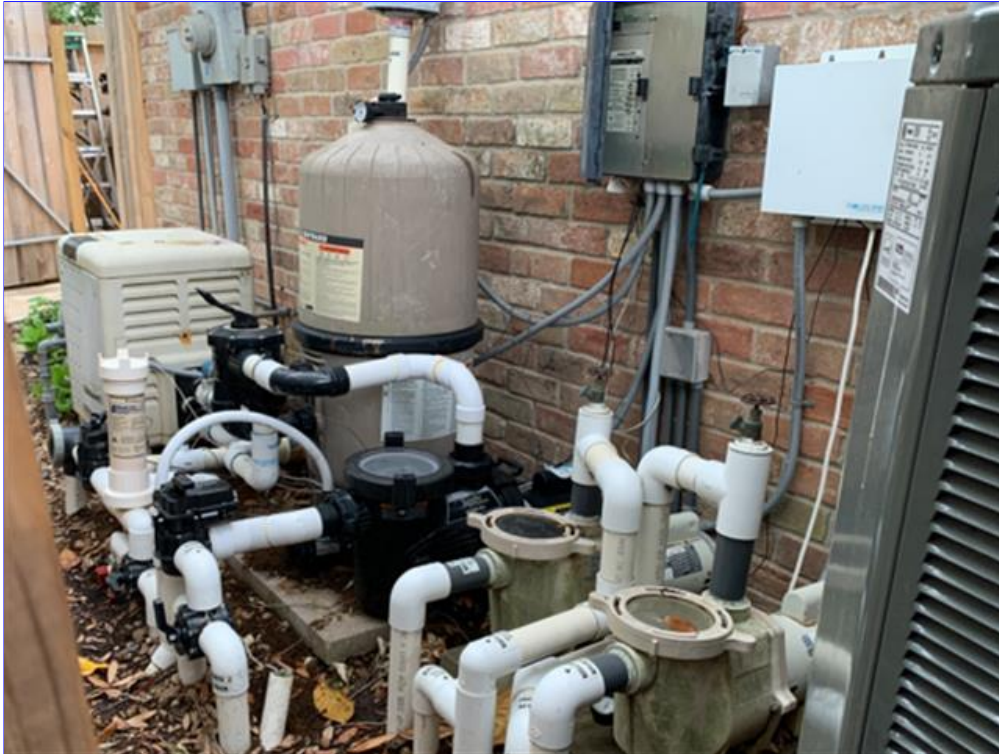
B. Photo 2(Picture) View of the installed pool equipment.
