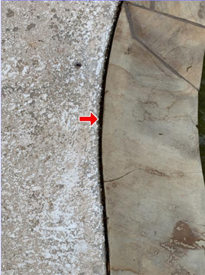
E. Photo 1(Picture) The sealant between the coping and the pool deck has failed.
