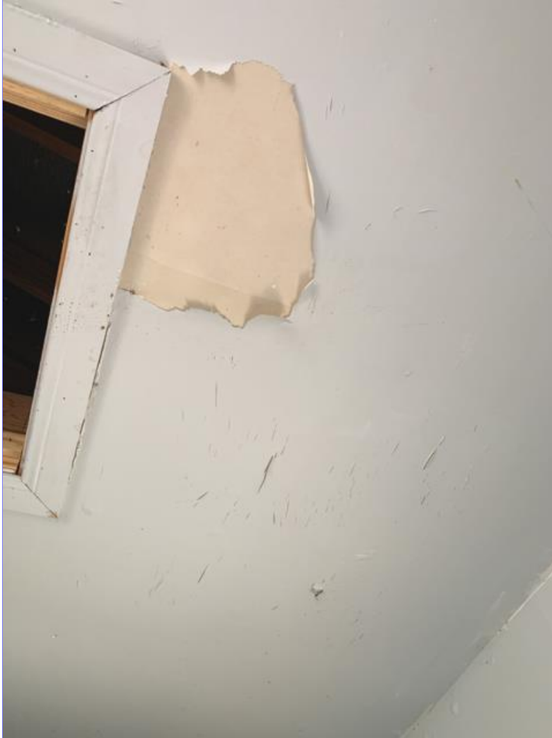
F. Photo 3(Picture) In the garage, areas were observed where are the paint has failed on the ceiling.
