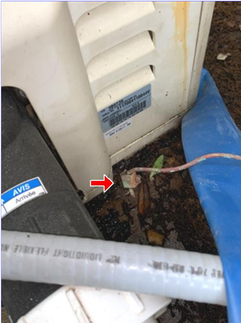
B. Photo 4(Picture) The cleaner pump motor housing and the Pool/ Spa Heater are not bonded to ground. Recommend correction.
