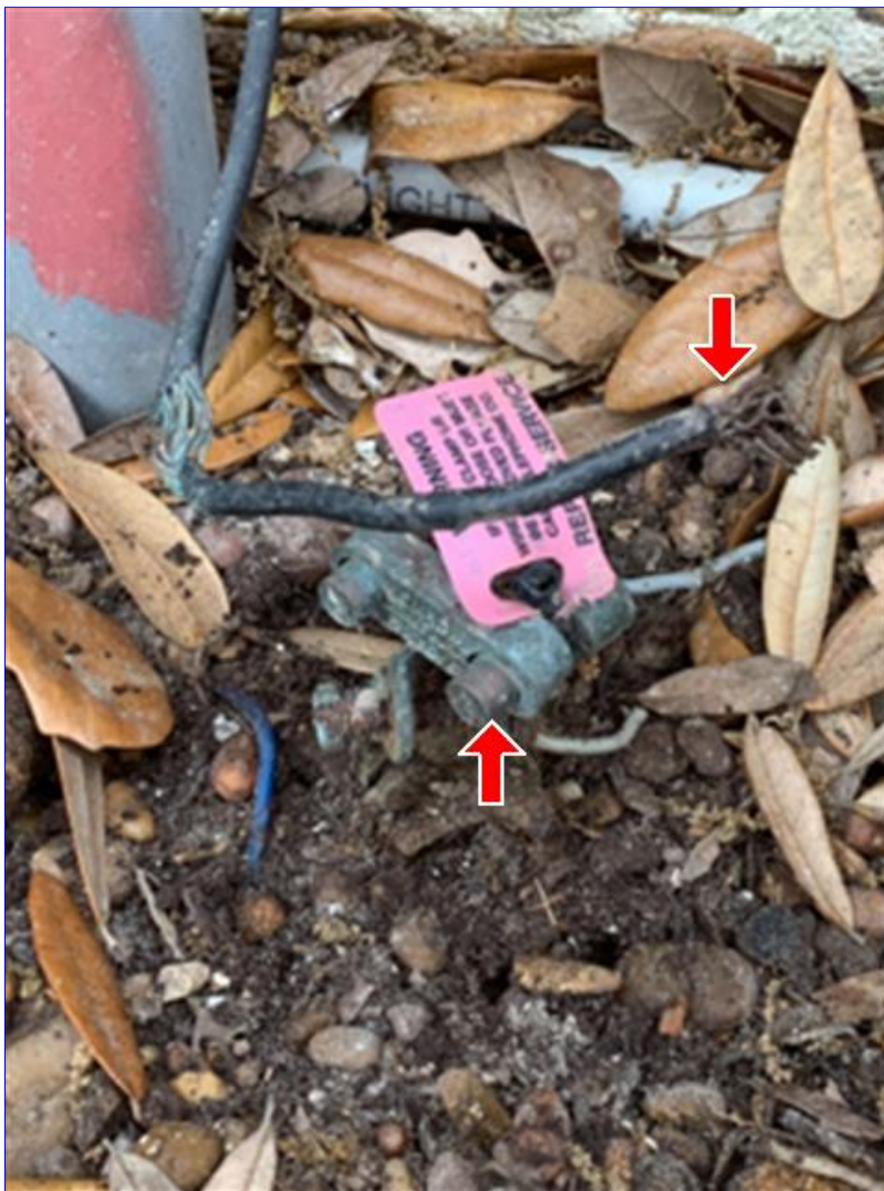
A. Photo 7(Picture) The system ground wire, is loose from the ground clamp or the ground clamp, is loose on the ground rod (electrode).
