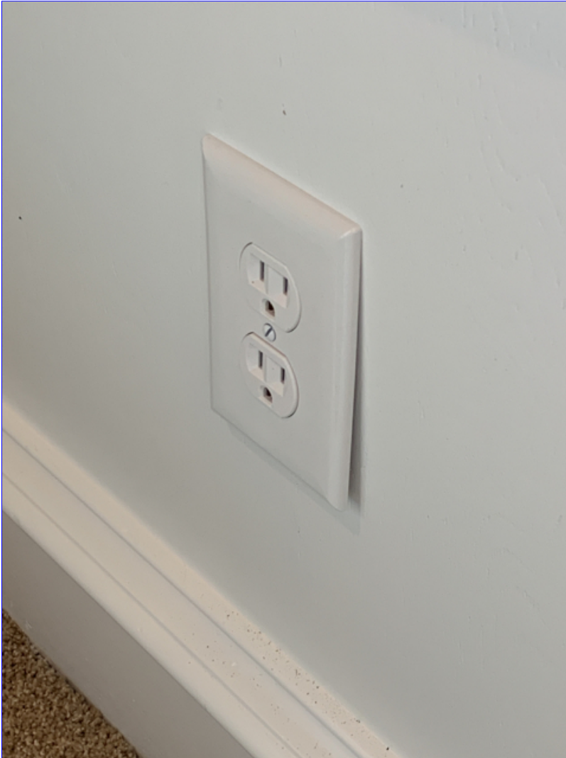
B. Photo 3(Picture) In the upstairs family room, an electrical outlet was observed, that needs to be re-secured at the wall.
