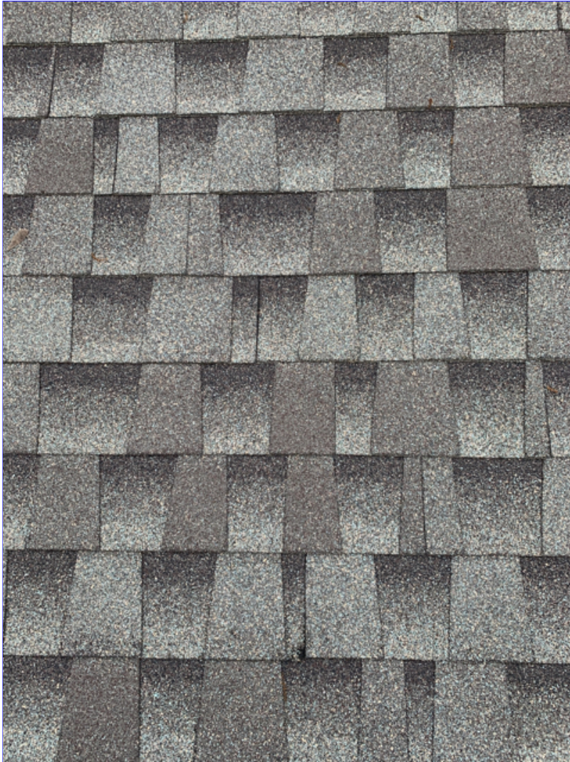
C. Photo 1(Picture) This roof is an Architectural style shingle that will typically last 20 years in this climate.
