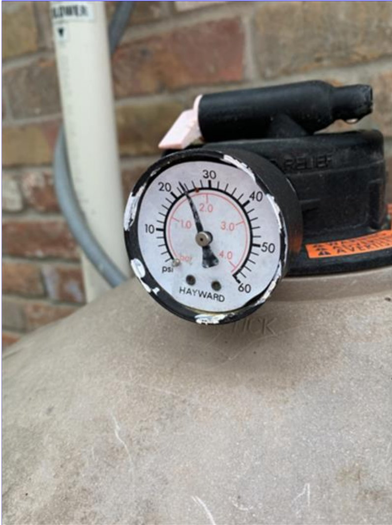
C. Photo 1(Picture) The pressure gauge is damaged. Recommend repair or replacement.
