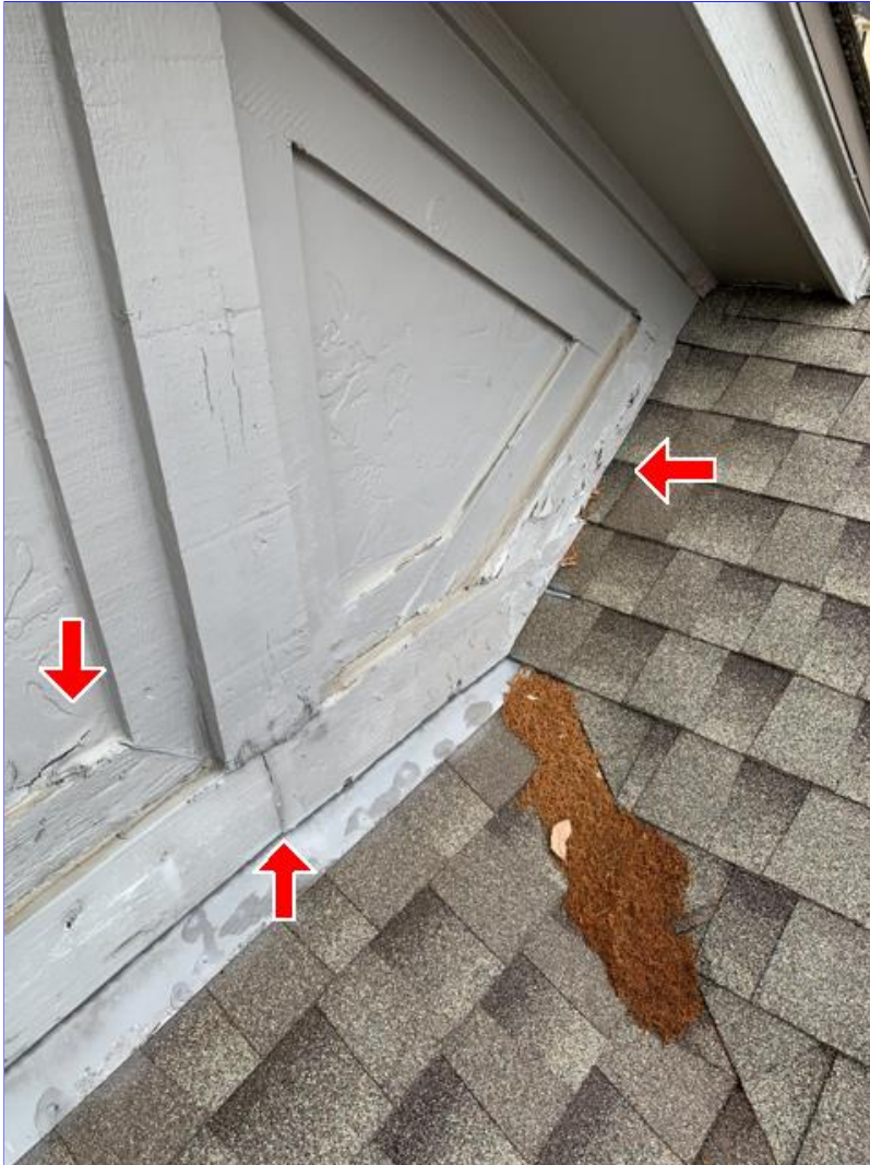
E. Photo 6(Picture) Wood rot was observed in areas of the siding and trim on the upper back side of the house.
