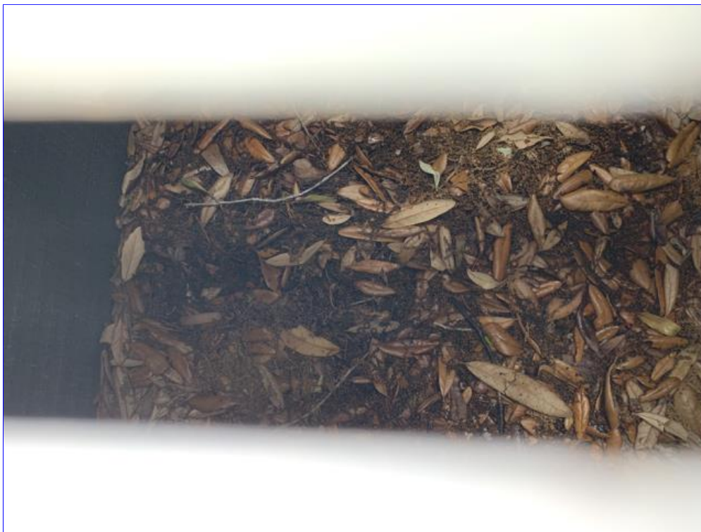
B. Photo 4(Picture) Debris and leaves need to be removed from the inside of the outside air conditioning units.
