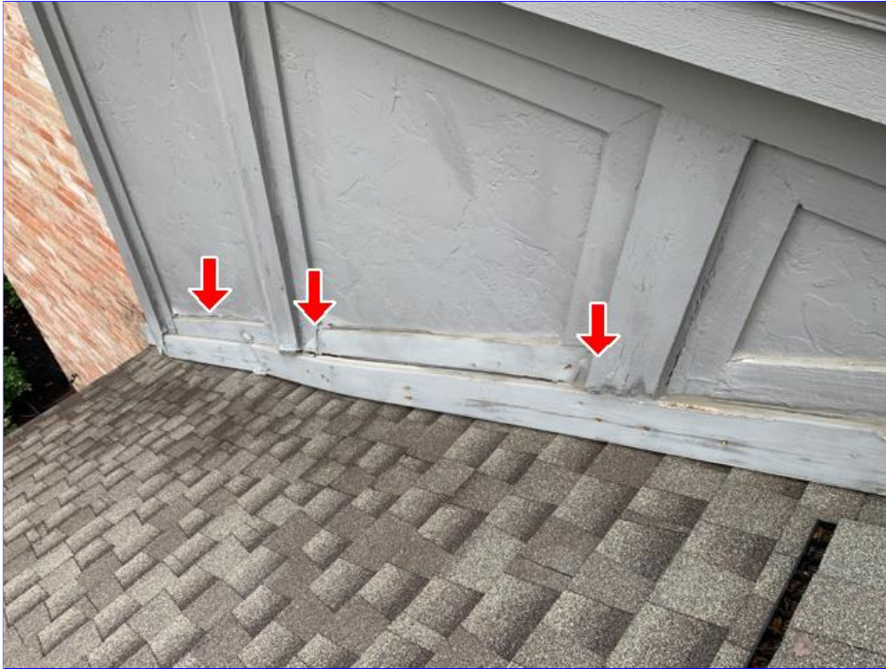
E. Photo 9(Picture) Wood rot was observed in areas of the siding and trim on the upper back side of the house.
