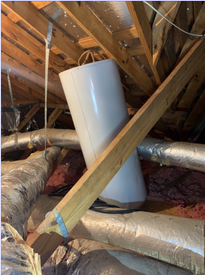
D. Photo 1(Picture) One of the old water heaters has been abandoned in the attic. Recommend the water heater be secured and strapped down.
