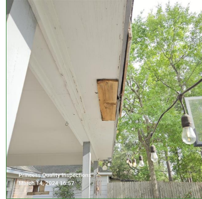
K. Item 2(Picture) Moisture damage observed at rear patio structure and mostly at fascia and recommend repair to prevent from creating an environment conducive to wood destroying insect activity.
