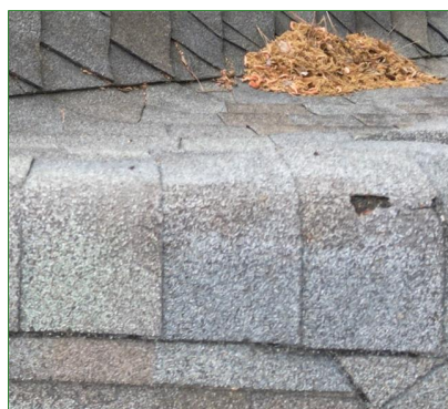
C. Item 10(Picture) Roof covering materials damage
