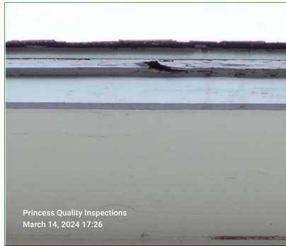
C. Item 31(Picture) Roof covering materials damage
