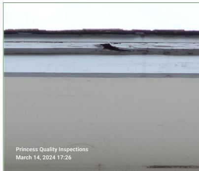
C. Item 35(Picture) Roof covering materials damage
