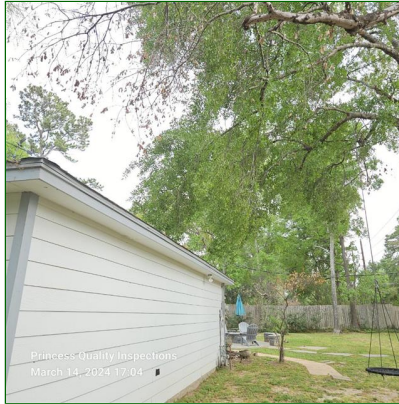
C. Item 1(Picture) Trimming tree branches away from structure is recommended to prevent damage.
