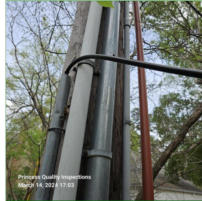
A. Item 13(Picture) A loose cable observed at the right rear corner of property and recommend further examination to identify the cable and correct as necessary.
