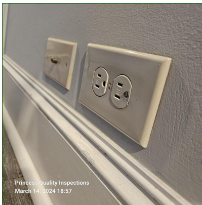
B. Item 3(Picture) A damaged prong what's observed stuck in a living room receptacle on exterior wall and recommend repair or replacement by a qualified electrical contractor for safety.
