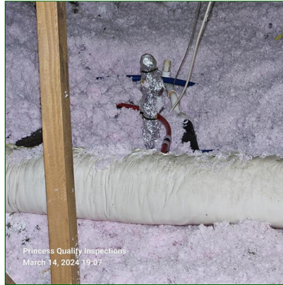
D. Item 5(Picture) Exposed water supply piping in attic space
