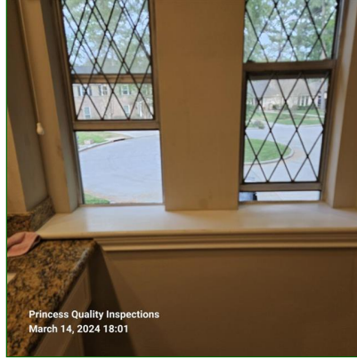
H. Item 10(Picture) One of the windows at the second floor hallway bathroom with only open a few inches with moderate force. FYI
