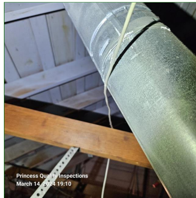
A. Item 3(Picture) The furnace exhaust Class B vent requires a 1-in clearance to combustible materials and recommend adjustment or relocating of signal wire that is in direct contact with furnace vent for safety.
