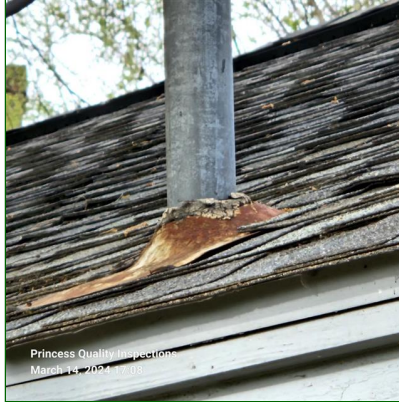
C. Item 2(Picture) The electric service mast boot is missing and recommend repair for long-term performance and to prevent moisture intrusions.
