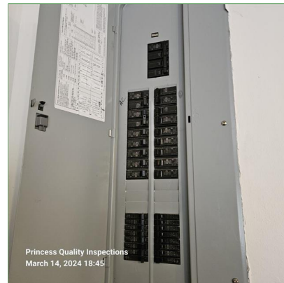
A. Item 4(Picture) The electrical distribution panel is located in the garage.
