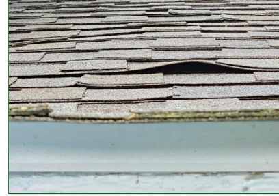
C. Item 28(Picture) Roof covering materials damage
