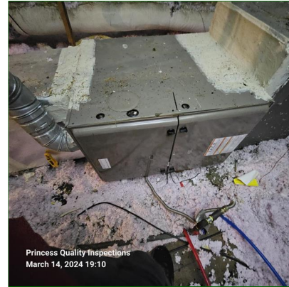
A. Item 2(Picture) The gas furnace is located in the attic. A solid service platform that extends 30 in to the front of the Furnace and evaporator is recommended and was required to be installed at last appliance installation.
