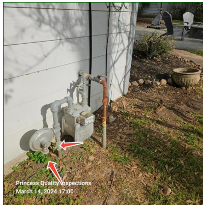
A. Item 14(Picture) The gas meter regulator/vent is closer to ground than the common 18" and the gas cut off valve is closer to the ground than the common 8 in. Any repairs to these items would be performed by the gas service provider with no charge. FYI
