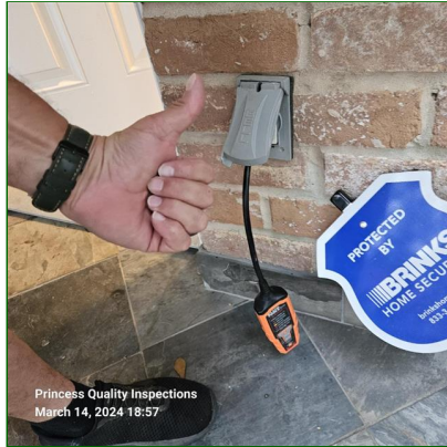
B. Item 4(Picture) The GFCI protected receptacles at rear patio, bathrooms and kitchen did respond to instrument testing at the time of inspection. FYI
