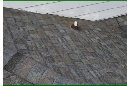
C. Item 20(Picture) Roof covering materials damage
