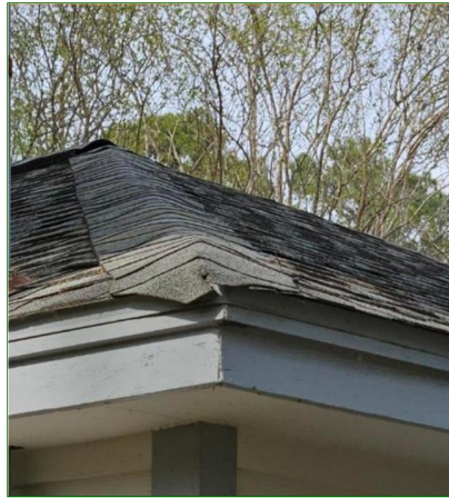
C. Item 29(Picture) Roof covering materials damage
