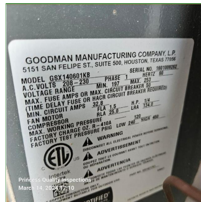
B. Item 4(Picture) The condenser was manufactured in 2016
