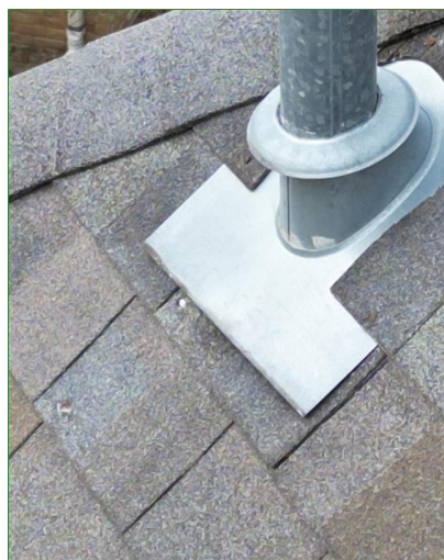
C. Item 16(Picture) Roof covering materials damage.
