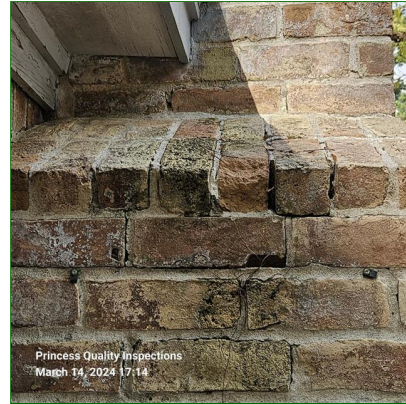
J. Item 6(Picture) Gaps in brick and mortar observed on chimney exterior and recommend repair of all gaps and cracks to prevent moisture seepage.
