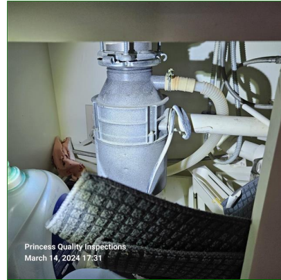
A. Item 2(Picture) The dishwasher drain line was installed without the benefit of an air gap or high loop in drain line to prevent food particles from reentering dishwasher.
