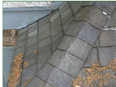
C. Item 4(Picture) Roof covering materials damage
