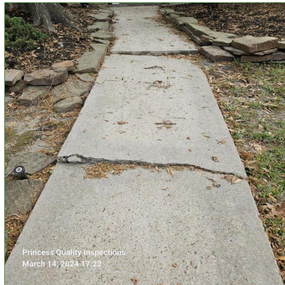
A. Item 33(Picture) Uneven walkways, driveway and or garage apron
