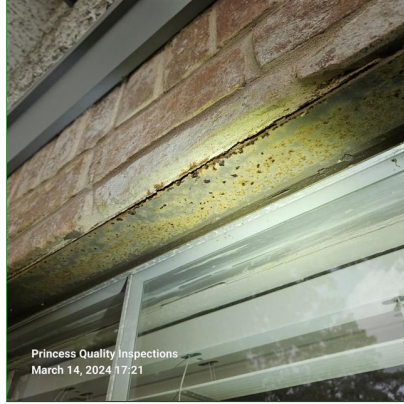
H. Item 4(Picture) Corrosion observed on metal load-bearing lintels above exterior windows and recommend removal of rust and treat with a rust inhibitor to prevent further deterioration of load bearing lintels.
