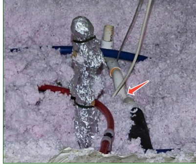
B. Item 11(Picture) The primary condensate drain line trap is not insulated. Insulating the Trap is recommended to prevent condensation and moisture damage.
