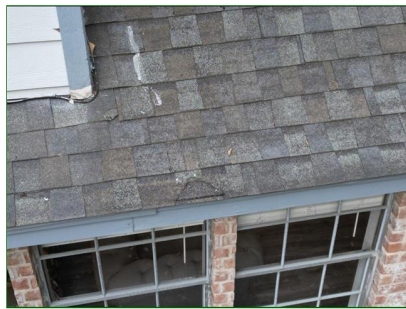
C. Item 21(Picture) Roof covering materials damage
