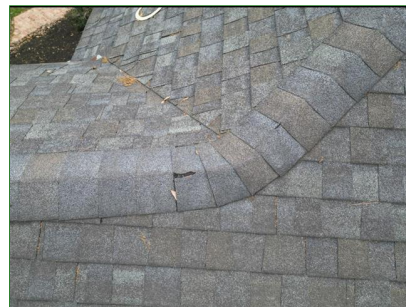
C. Item 24(Picture) Roof covering materials damage
