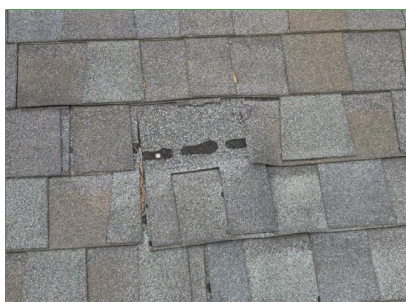
C. Item 17(Picture) Roof covering materials damage
