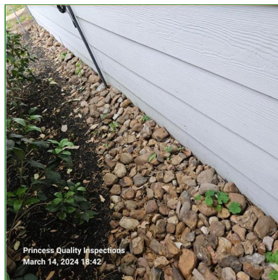
A. Item 31(Picture) Foundation not visible
