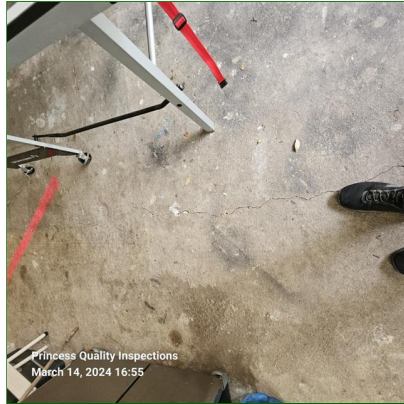
A. Item 21(Picture) Cracks observed in garage floor were cosmetic at the time of inspection and recommend monitoring for changes in size and shape and repair if necessary.
