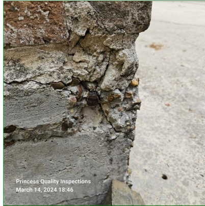
A. Item 39(Picture) Exposed metal Foundation support observed at right front corner and on right side under window with cracked the glass and recommend patching with a high strength concrete patch to prevent premature deterioration of metal Foundation support.
