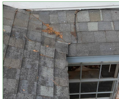
C. Item 22(Picture) Roof covering materials damage
