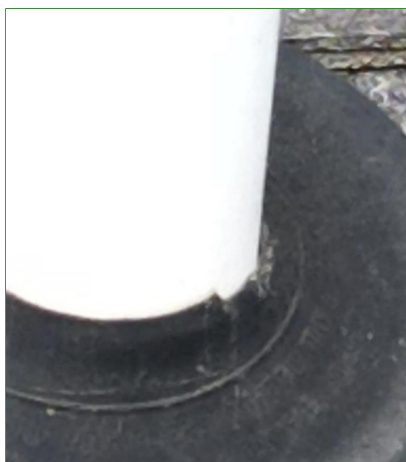
C. Item 15(Picture) Roof covering materials damage
