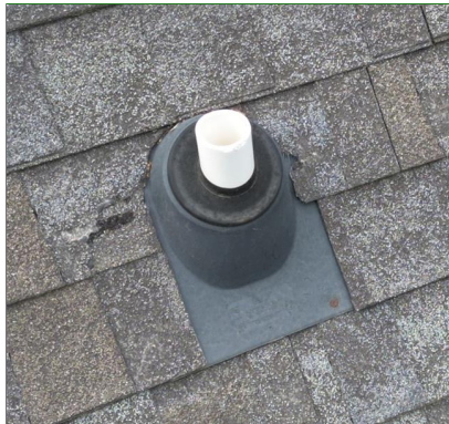
C. Item 13(Picture) Roof covering materials damage
