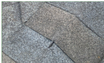
C. Item 25(Picture) Roof covering materials damage
