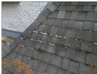
C. Item 5(Picture) Roof covering materials damage
