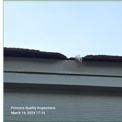
C. Item 34(Picture) Roof covering materials damage
