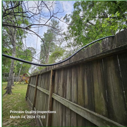
A. Item 12(Picture) A loose cable observed at the right rear corner of property and recommend further examination to identify the cable and correct as necessary.
