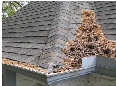
C. Item 8(Picture) Roof covering materials damage
