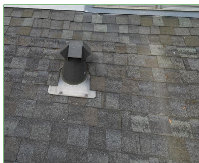
C. Item 18(Picture) Roof covering materials damage
