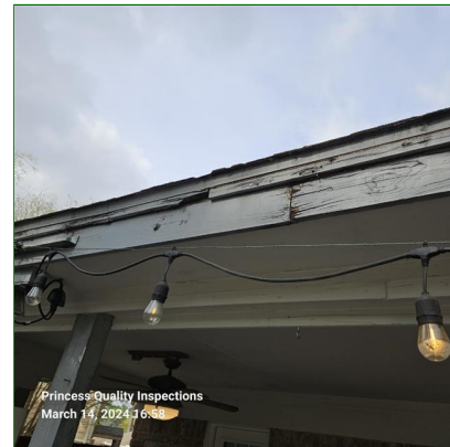
K. Item 4(Picture) Moisture damage observed at rear patio structure and mostly at fascia and recommend repair to prevent from creating an environment conducive to wood destroying insect activity.
