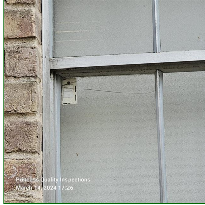
H. Item 7(Picture) Broken glass observed on window at right side of Home facing rear and recommend replacing broken glass.
