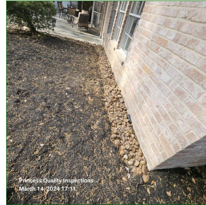
A. Item 28(Picture) Weep holes not visible
