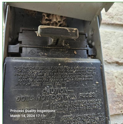
B. Item 7(Picture) Wasp nests observed inside of the condenser service disconnect panel and recommend removal by qualified HVAC or electrical contractor for safety.
