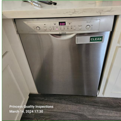
A. Item 1(Picture) The dishwasher was performing at the time of inspection.
