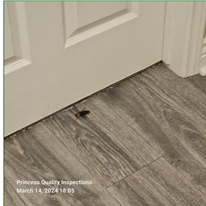
F. Item 15(Picture) Live roaches were observed at 2 locations at second floor and recommend further examination by a qualified pest control contractor to identify and treat as necessary to prevent infestations in the home.
