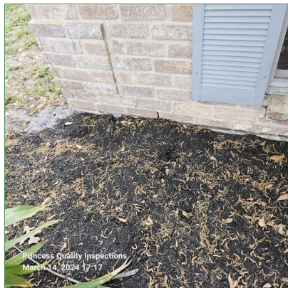
A. Item 29(Picture) Soil or flower beds obscure Foundation and or damage from View
