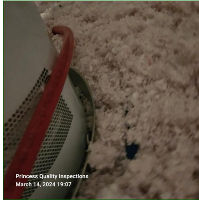
C. Item 4(Picture) Removal of all debris from water heater drip pan is recommended to prevent clogging of drain.
