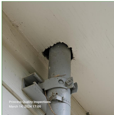
A. Item 11(Picture) Sealing off gap in soffit at electrical service mask penetration at rear of garages recommended to prevent flying insect and Vermin nesting Within structure.
