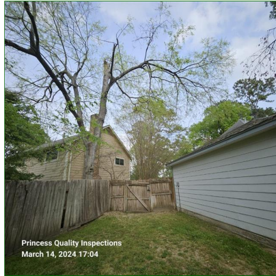
B. Item 3(Picture) Neighbors tree branches observed hanging over onto property
