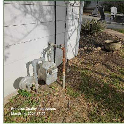
A. Item 2(Picture) The natural gas service entrance and cut off is located at the rear of the garage. FYI
