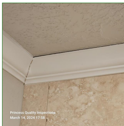
F. Item 10(Picture) Gaps/ separation in crown molding observed at master bathroom.
