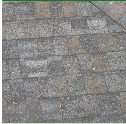
C. Item 19(Picture) Roof covering materials damage
