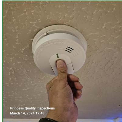
B. Item 1(Picture) The smoke detectors present in the home did respond to testing at the time of inspection and are interconnected as required by modern standards. FYI
