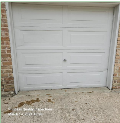
G. Item 3(Picture) One car garage door panels observed to contain creases from buckling but did not hinder the operation of the door. FYI
