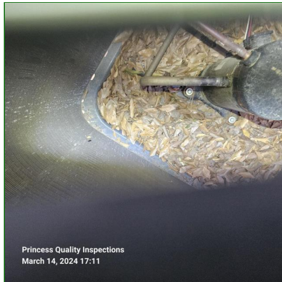
B. Item 5(Picture) Debris observed inside condenser housing and service or repair by a qualified HVAC contractor to prevent reductions inefficiency from debris blockages.
