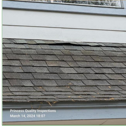
C. Item 27(Picture) Roof covering materials damage
