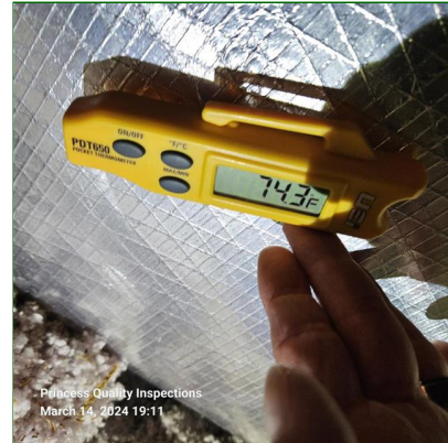
B. Item 2(Picture) Air return temperature
