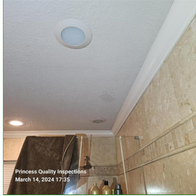
F. Item 3(Picture) Moisture stains observed in drywall ceilings at various locations.
