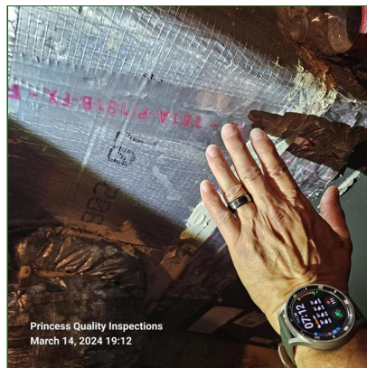
B. Item 12(Picture) Air leaks in air handler seams observed at various locations and recommend further examination by a qualified HVAC contractor and repair all air leaks to prevent condensation and moisture damage.
