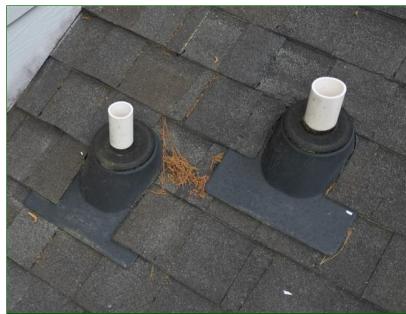
C. Item 23(Picture) Roof covering materials damage
