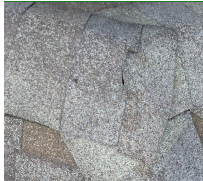
C. Item 14(Picture) Roof covering materials damage
