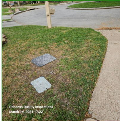
A. Item 1(Picture) The water meter and Municipal cutoff is located next to the driveway at the left side of Home facing front. FYI
