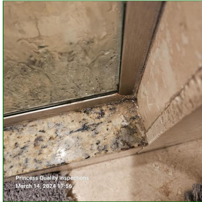
A. Item 12(Picture) Shower enclosure leaks observed at 2 or locations of Master shower and recommend repairing leaks to prevent moisture damage to materials.
