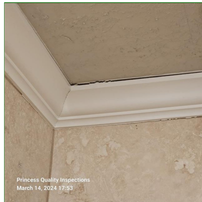
F. Item 8(Picture) Gaps/ separation in crown molding observed at master bathroom.
