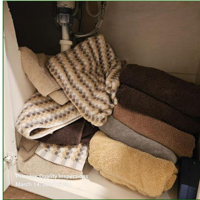
B. Item 1(Picture) Occupant stored items under sinks obscured items to be inspected
