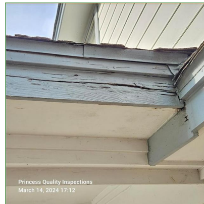
C. Item 36(Picture) Roof covering materials damage
