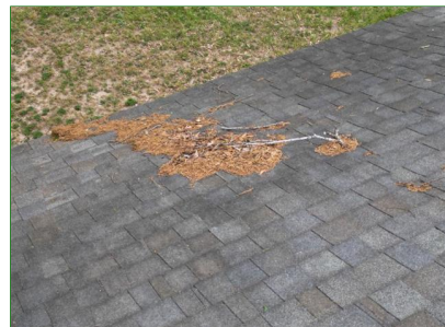
C. Item 26(Picture) Roof covering materials damage
