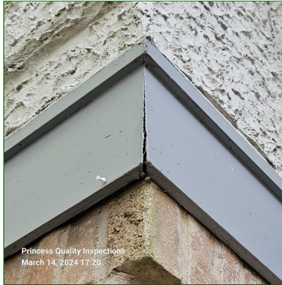
E. Item 6(Picture) uneven gap in frieze board
