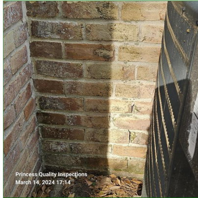
J. Item 5(Picture) Gaps in brick and mortar observed on chimney exterior and recommend repair of all gaps and cracks to prevent moisture seepage.
