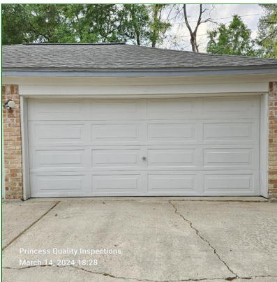
G. Item 4(Picture) A slight sag observed at center of garage opening/header and common in this age of home. The header may need reinforcing in the future if sagging worsens. FYI
