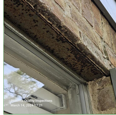
H. Item 5(Picture) Corrosion observed on metal load-bearing lintels above exterior windows and recommend removal of rust and treat with a rust inhibitor to prevent further deterioration of load bearing lintels.
