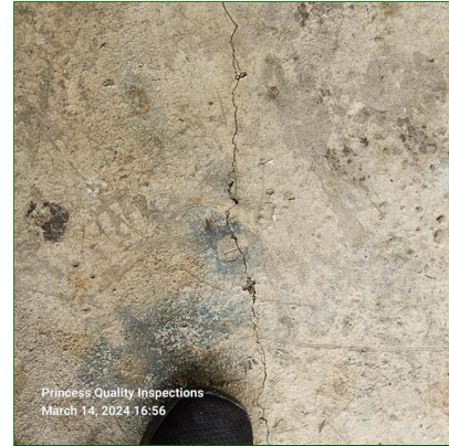
A. Item 22(Picture) Cracks observed in garage floor were cosmetic at the time of inspection and recommend monitoring for changes in size and shape and repair if necessary.
