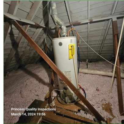
C. Item 2(Picture) The water heater is located in the high attic
