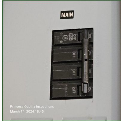
A. Item 5(Picture) 4x200 amp service disconnect
