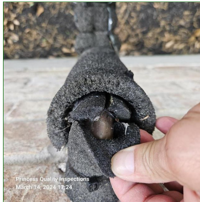
A. Item 3(Picture) Copper water service entrance
