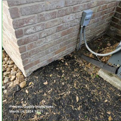
A. Item 27(Picture) Weep holes not visible
