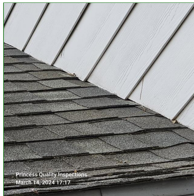
E. Item 5(Picture) Cement fiber siding observed in direct contact with roof coverings at various locations and obscuring from view any metal flashing. Due to the age and condition of roof coverings, the wall flashing will be exposed and can be repaired if needed at the next roof covering change. Cement fiber manufacturers recommend a minimum clearance to roof covering materials of an inch and a half to prevent premature deterioration of cement fiber. FYI
