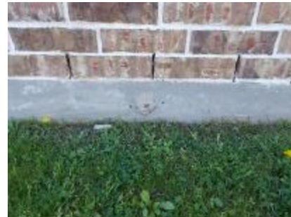
exposed cable ends rear
