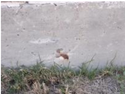
Exposed cable end left
