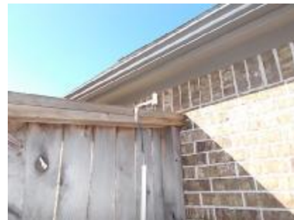
sprinkler rain sensor
