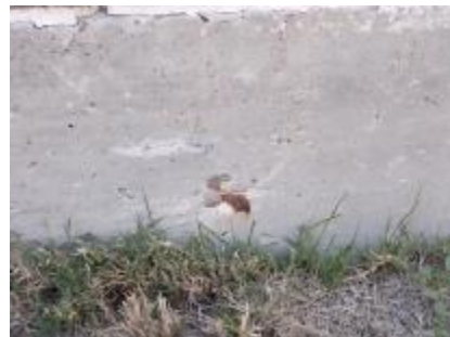
left side exposed cable end
