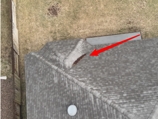
Debris rear of roof
