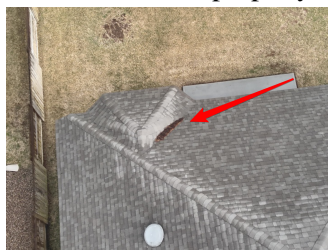
Debris rear of roof
