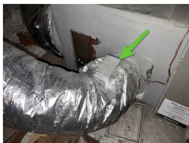
Fresh Air Control Box
