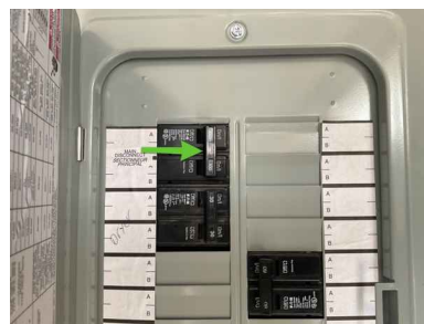
Main Disconnect for Sub-Panel
