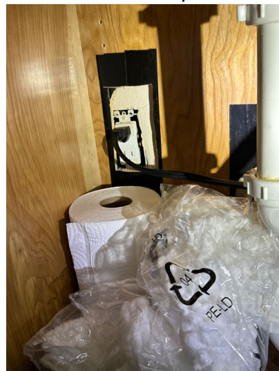
Outlet cover was missing above the microwave and at the disposal.
