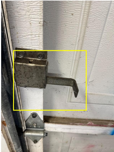
Door lock should be disabled since opener is present.
