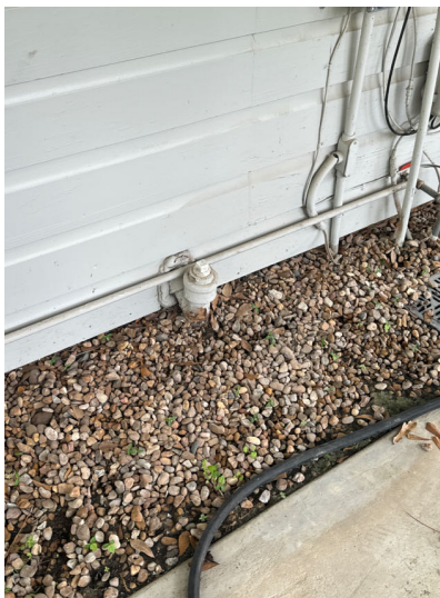
Cast iron drain pipe was observed. Hydrostatic pressure testing and/or video camera testing of drain pipe is recommended due the age and type of piping.
