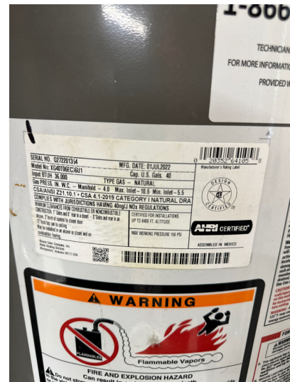
Water heater was gas powered and appeared to be manufactured by Rheem in 2022.
