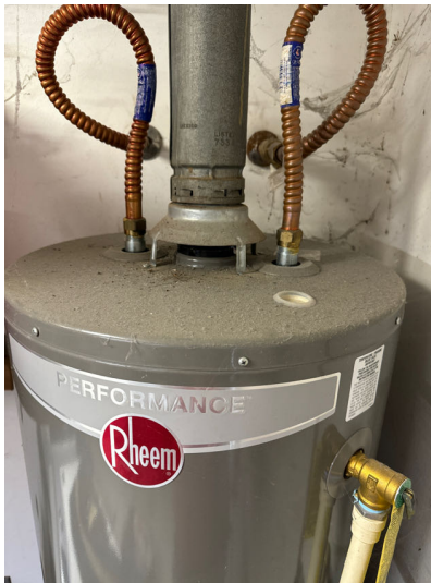
Plumbing System Water Heating Equipment
