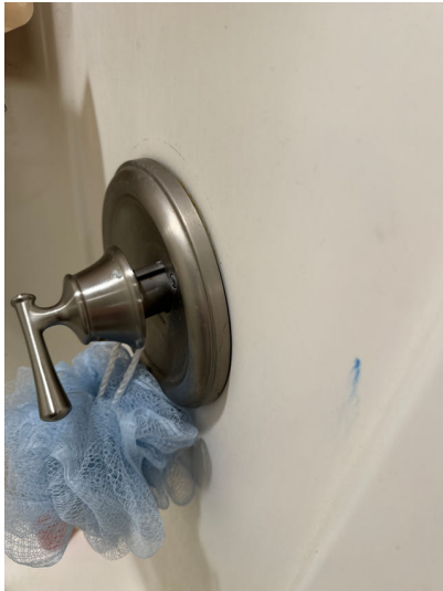
Plumbing fixtures in the shower were not sealed.
