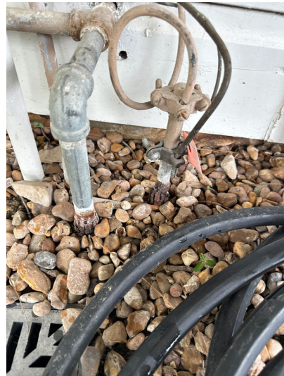
Gas supply pipe near the electric panel contained significant rust.
