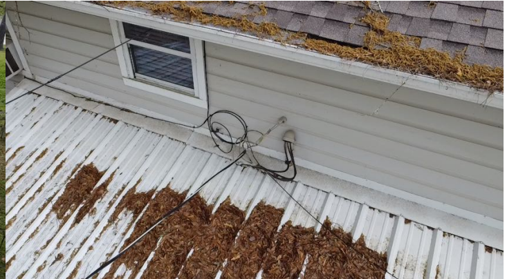
Pine needles and tree debris should be cleared from valleys and walls, to allow unimpeded flow of rain water.
