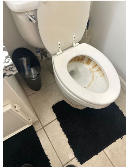
Toilet was loose in the upper guest bathroom . Examine flange and replace wax ring and seal toilets to the floor.
