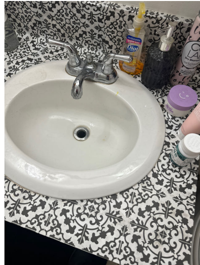
Sink stopper were not present in the upper bathrooms.
