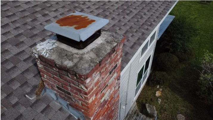
The chimney cap was rusted and should be sealed to stop oxidation.
