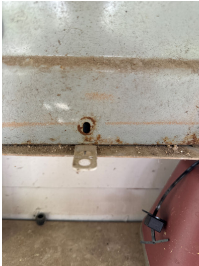
The panel cover was missing its fastener.
