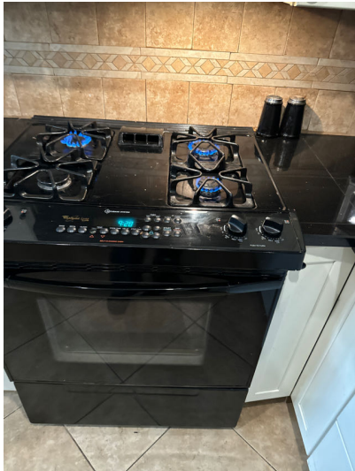
The ignition for the two burners on the right side of the cook top was inoperative. Burners can be lit with a lighter.
