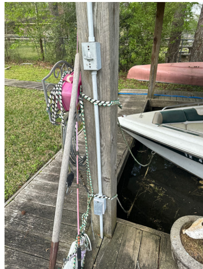
The boat dock electrical receptacles and motors did not appear to be GFI protected.
