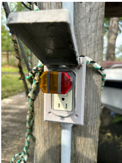
The boat dock electrical receptacles and motors did not appear to be GFI protected.
