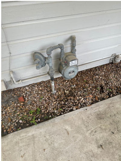
Gas meter was at the front of the home.
