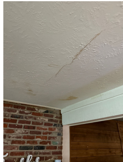
Ceiling stains were noted in the lower bedroom and the lower living area. No moisture was detected at the time of inspection.
