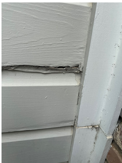
Wood deterioration was noted at some areas of siding including the left side of the garage and the right side wall.
