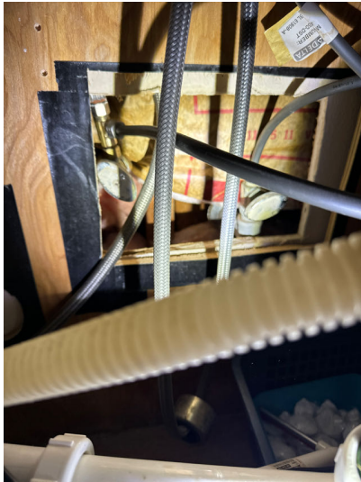
The wall under the sink should be covered with drywall.
