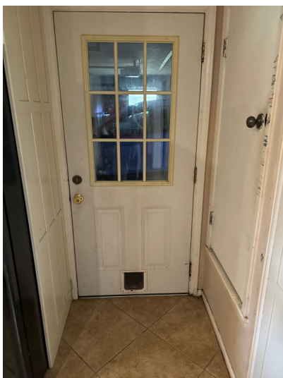
The garage pedestrian door fire separation was compromised with a pet door.
