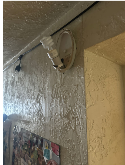
The fixtures in the upper left bedroom were damaged.
