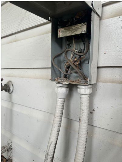
One AC disconnect was missing its cover.
