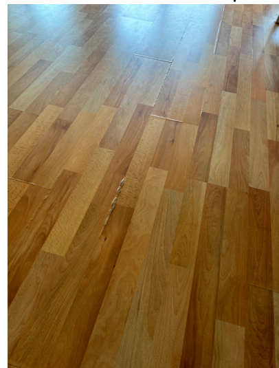
Small areas of water damage was noted on the upper level living area.
