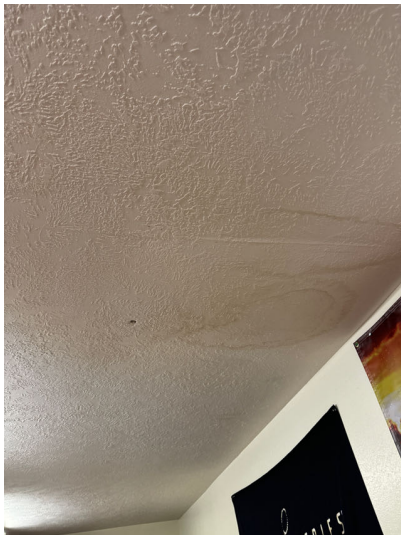
Ceiling stains were noted in the lower bedroom. No moisture was detected at the time of inspection.
