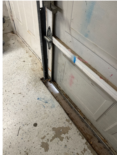
Electronic sensor was not present. This is a safety issue.
