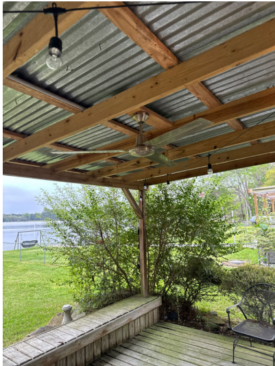
The right side patio fan did not operate.
