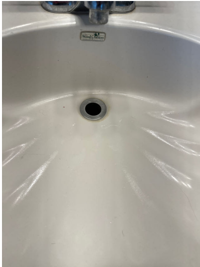
Sink stopper were not present in the primary bathroom.
