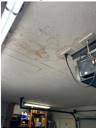
Ceiling stains were noted in the lower bedroom and the lower living area, the garage. No moisture was detected at the time of inspection.
