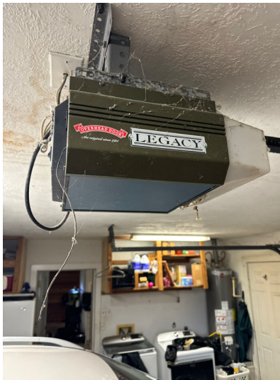
Garage door opener was an Overhead Door type chain drive without sensors.
