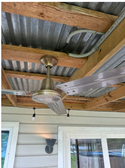
Conduit should continue to the ceiling fan junction boxes.
