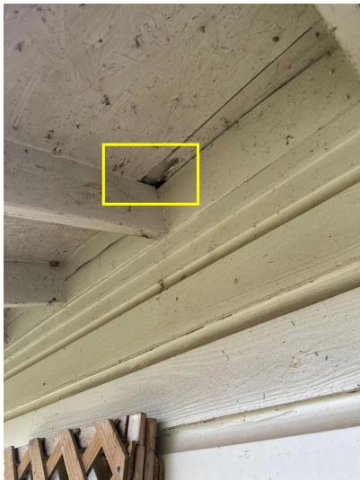
Wood deterioration was noted at some areas of siding including the left side of the garage and the right side wall.
