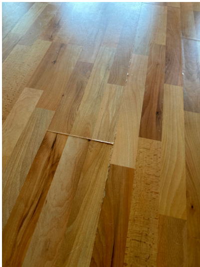
Small areas of water damage was noted on the upper level living area.
