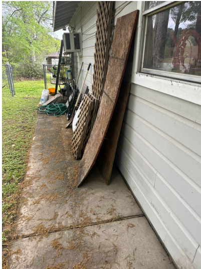
Building material and personal items should be moved away from the exterior walls.
