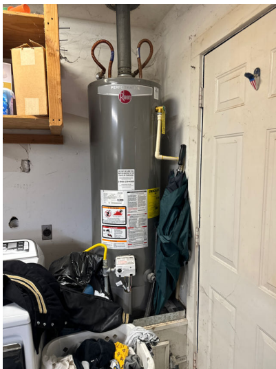
Plumbing System Water Heating Equipment
