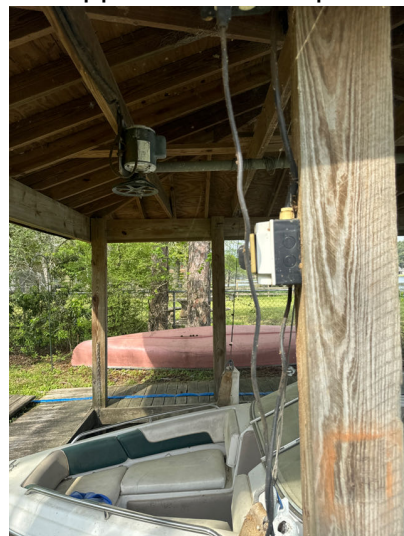
The boat dock electrical receptacles and motors did not appear to be GFI protected.
