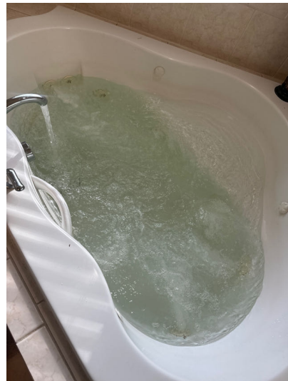
Hydro-massage unit in master bathroom appears to be operating normally.
