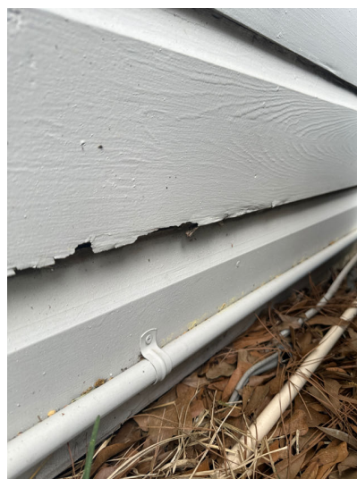
Wood deterioration was noted at some areas of siding including the left side of the garage and the right side wall.
