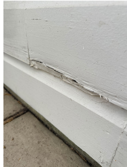
Wood deterioration was noted at some areas of siding including the left side of the garage and the right side wall.
