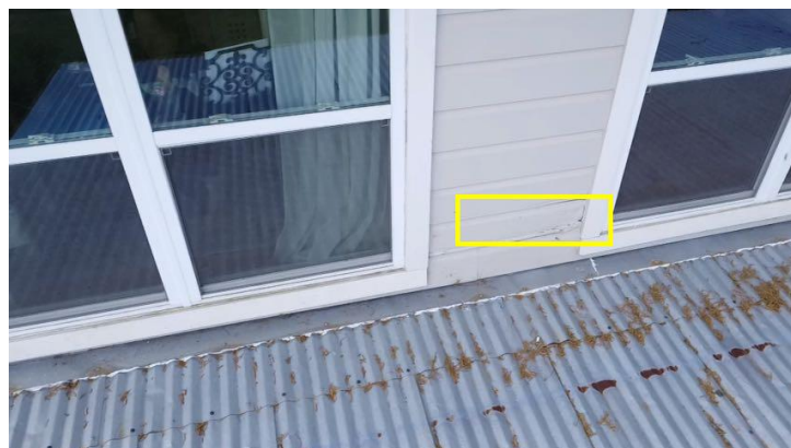
Wood deterioration was noted at some areas of siding including the left side of the garage and the right side wall.
