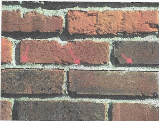
brick crack on right wall
