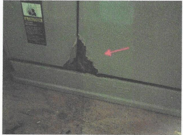
rust to coil / housing
