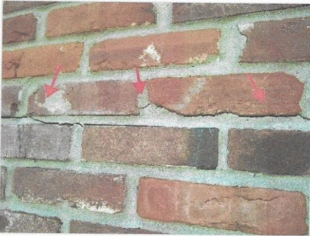
brick crack on left wall
