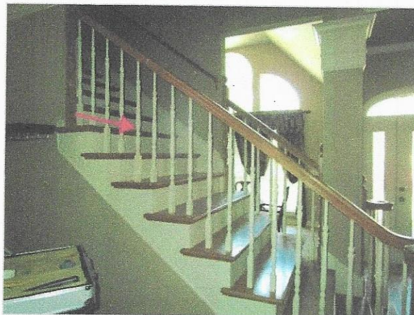
posts too wide
