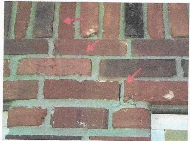
brick crack between doors
