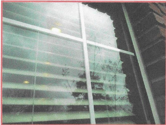
Failed Thermal Seal at Office Window
