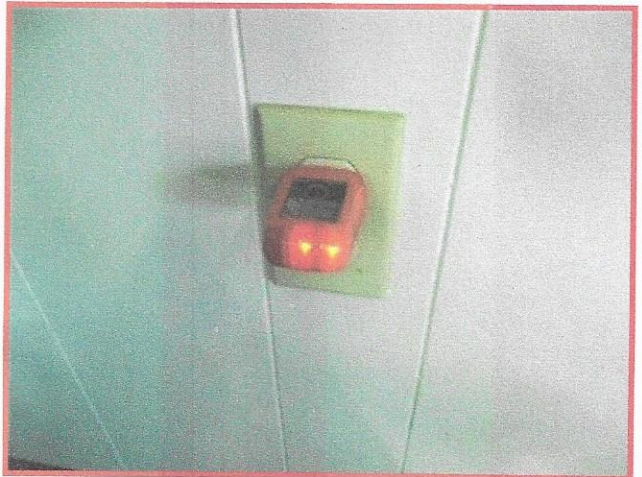
Missing GFI Protection at Garage Outlet
