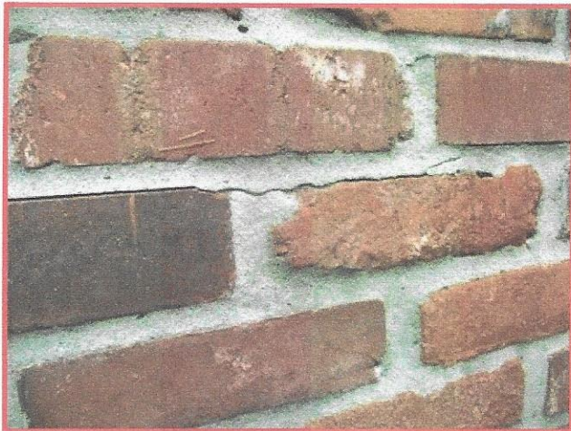
Cracked Mortar at Right Side
