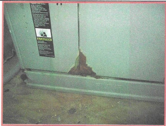
Corroded Upper Level HVAC Cabinet
