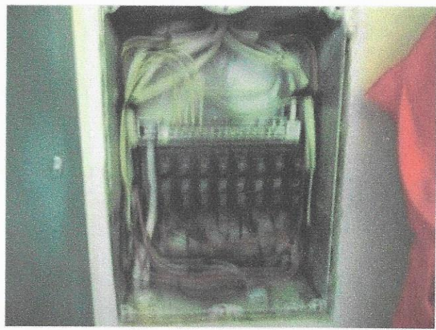
Closet Electric Sub-Panel
