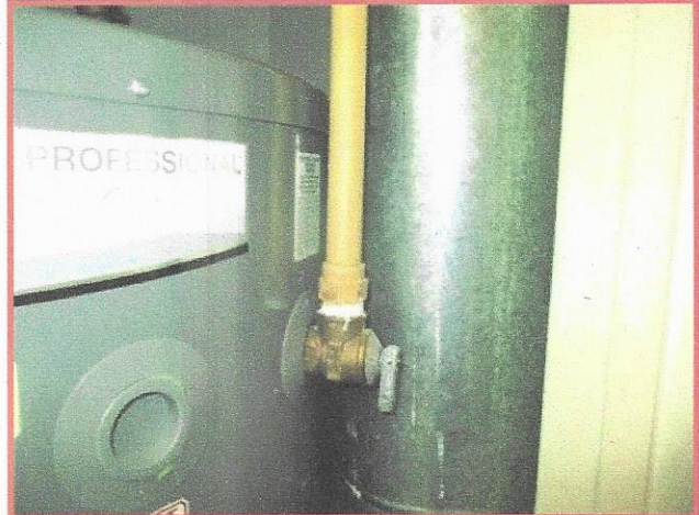
Water Heater TPR Valve Extension Runs Uphill
