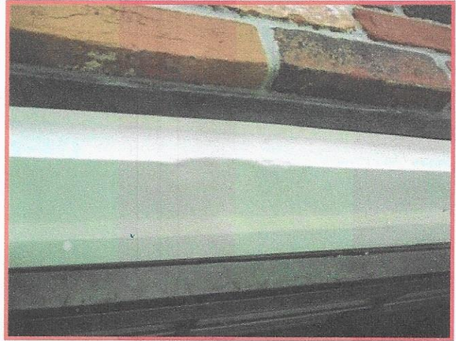
Damaged Header at Garage Door
