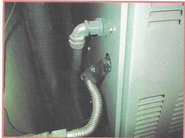
Flexible Fuel Line Penetrates Furnace Cabinet
