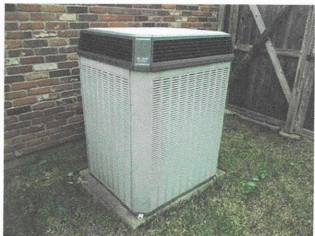
Main Level A/C Unit
