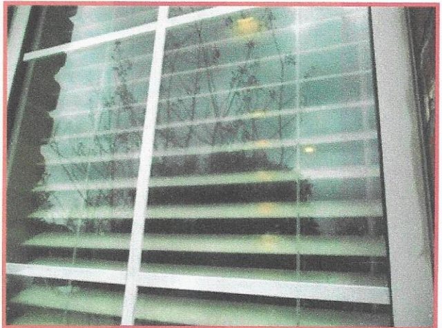
Failed Thermal Seal at Office Window
