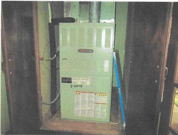
Main Level Heating Equipment
