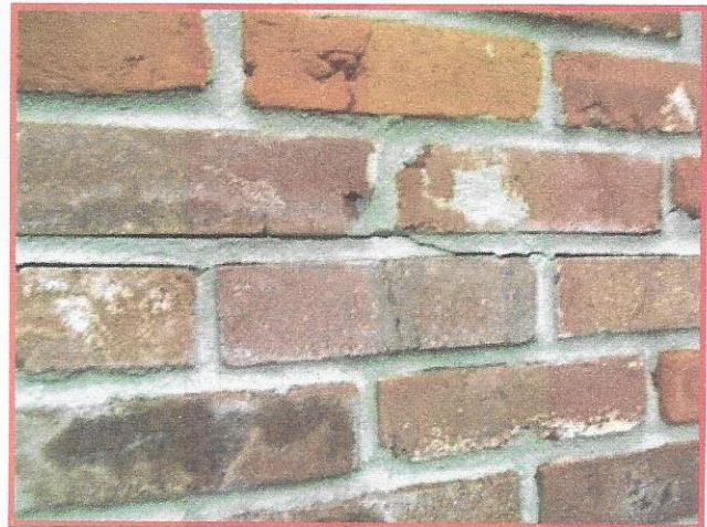
Cracked Mortar Left Side of Garage
