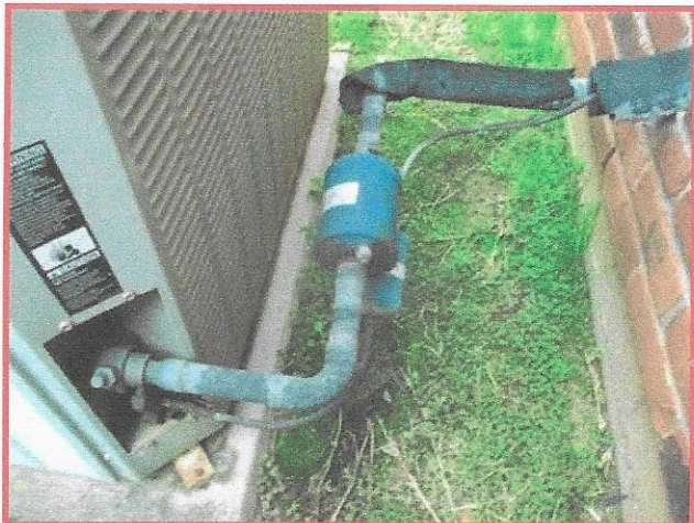
Damaged Insulation on Refrigerant Line
