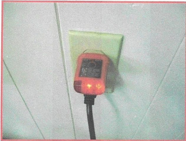
Missing GFI Protection at Garage Outlet
