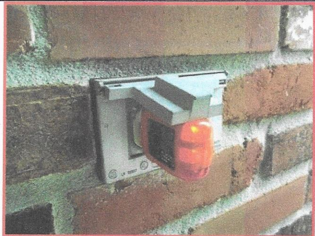
Missing GFI Protection at Exterior Outlet
