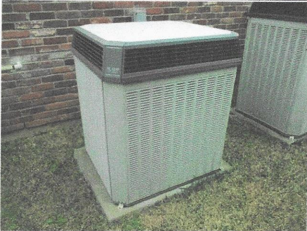
Upper Level A/C Unit
