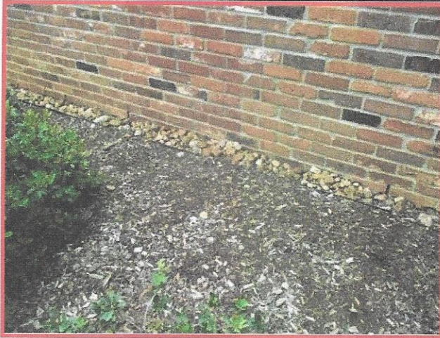
High Grading at Rear
