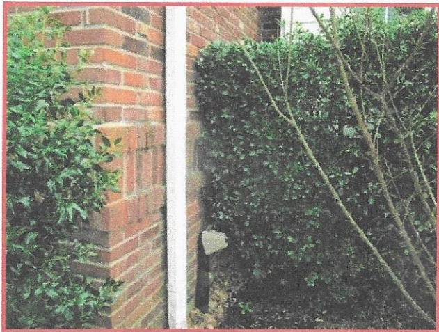
Vegetation in Contact with Structure
