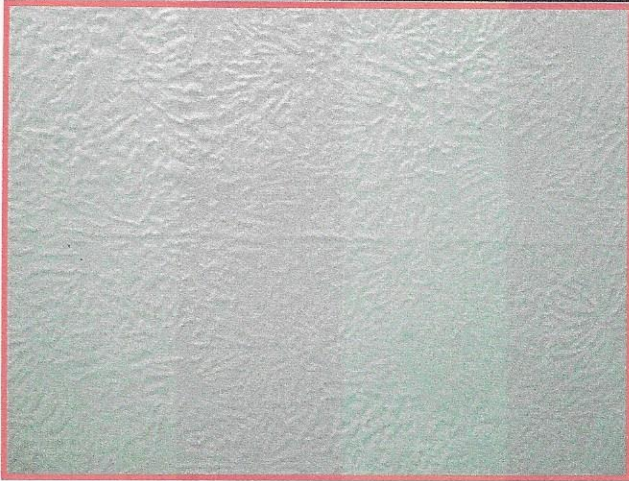
Cracked Garage Ceiling
