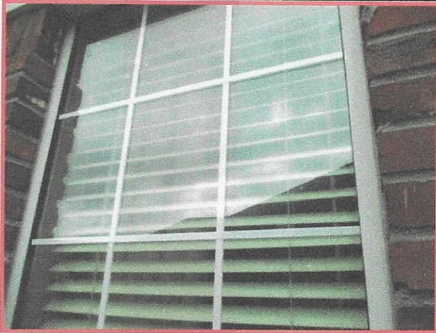
Failed Thermal Seal at Primary Bedroom Window
