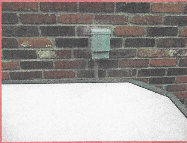
Electric Disconnect Behind Unit
