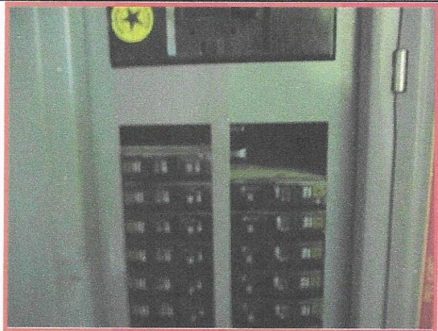
Open Knockouts at Electric Panel
