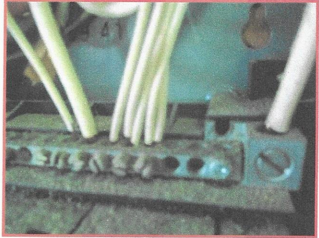
Double Tapped Neutrals on Sub-Panel Buss Bar
