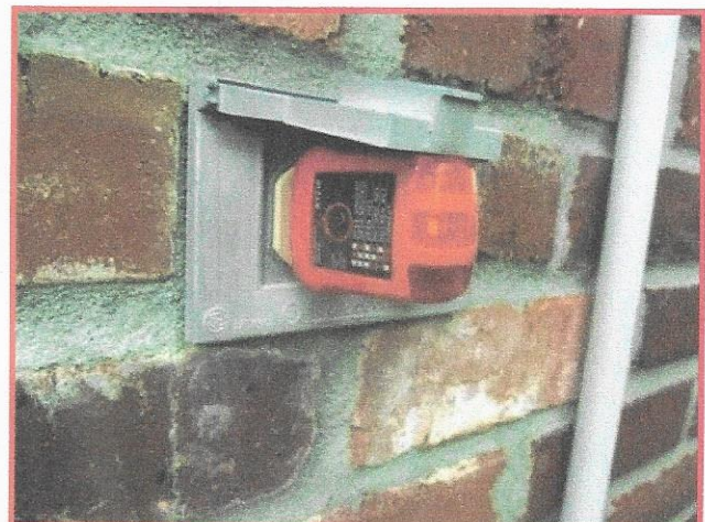
Missing GFI Protection at Garage Exterior Outlet
