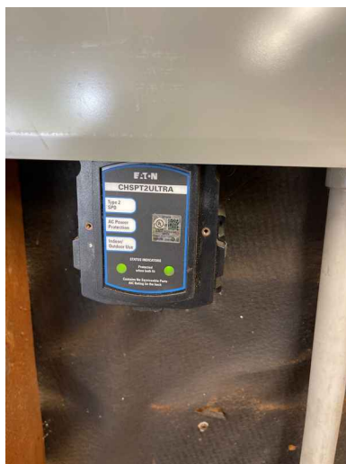
Main Service Panel Location: Garage
