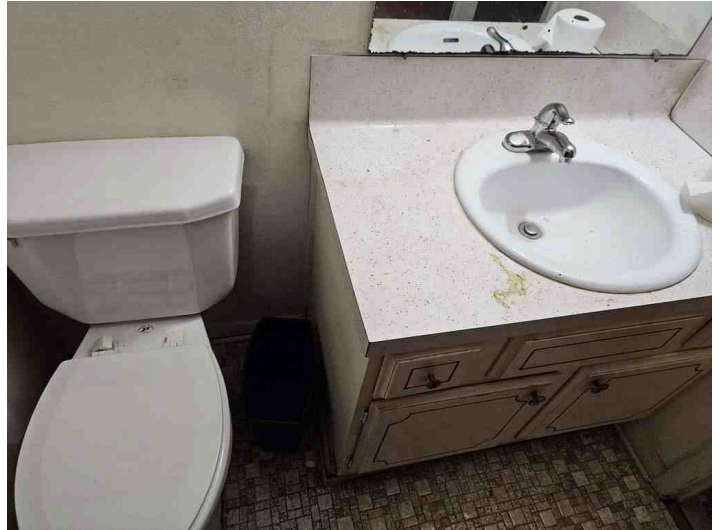
Typical Interior Photo
