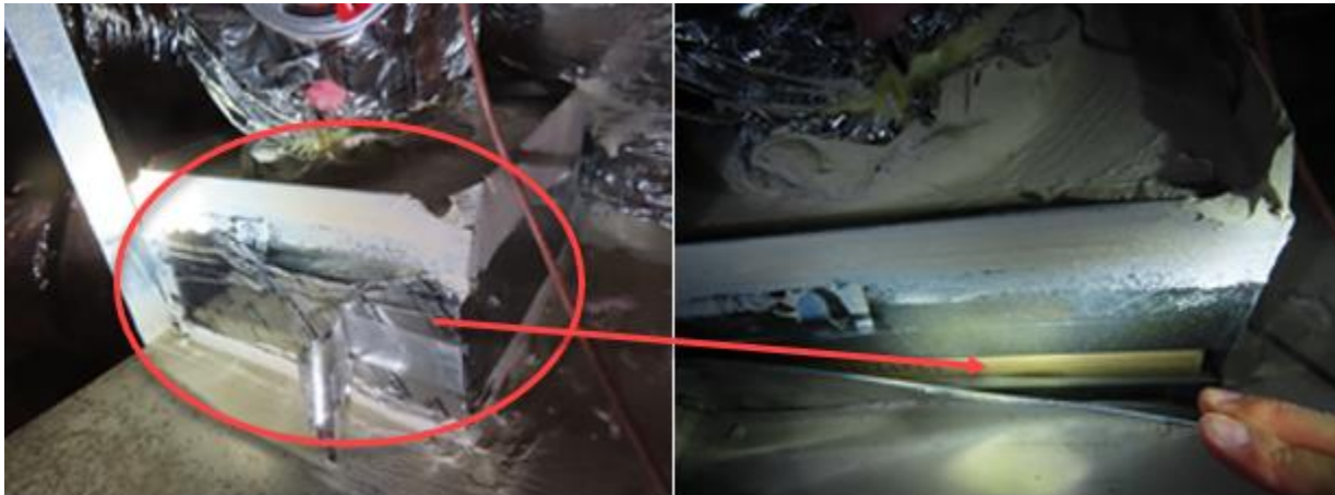
Filter ( size: 12x12) was dirty and needs to be replaced every few months on furnace 1
