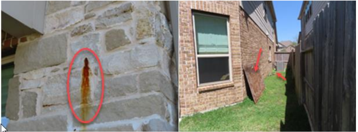
Rust stain was visible on stone wall
