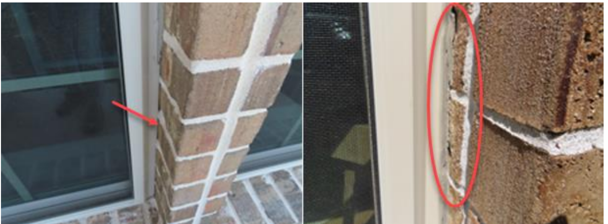
Some caulking was missing on front window jamb
