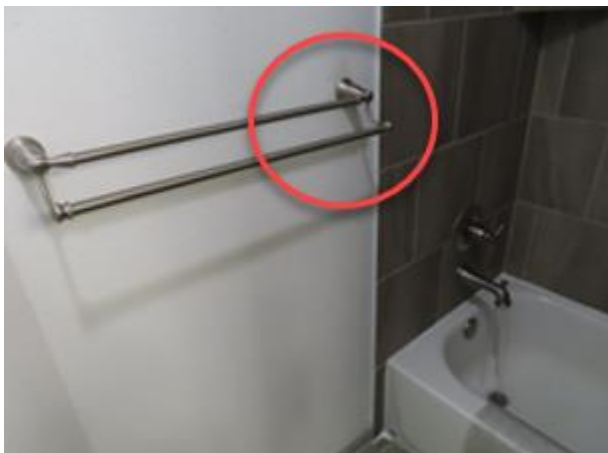
Damaged finish at tub in right bath on second floor
