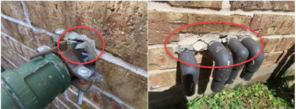
All penetrations through brick should be sealed to prevent water infiltration
