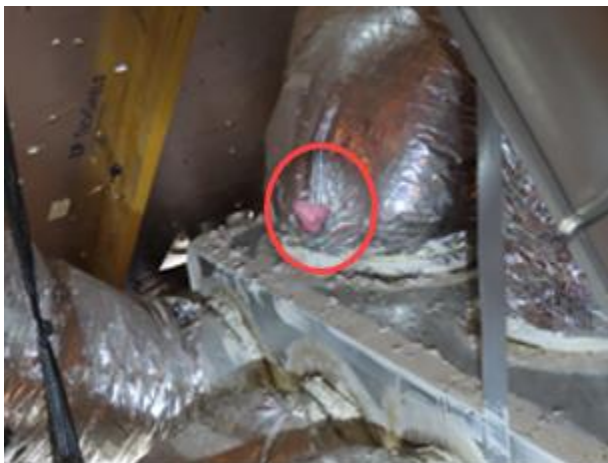
Damaged wrap was visible on some ducts
