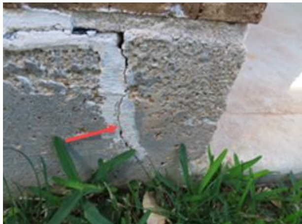
Small crack was visible on some foundation corner
