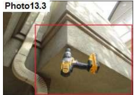
Substrate Damage / Assess, Repair & Install Relief
