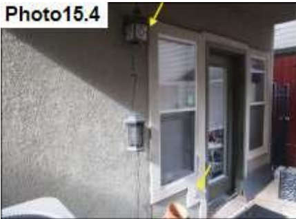
Penetration Sealants / Seal
