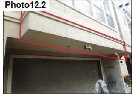
Substrate Damage / Assess, Repair & Install Relief
