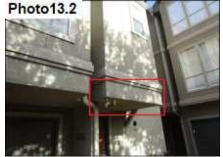
Substrate Damage / Assess, Repair & Install Relief
