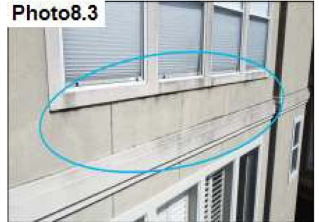
Run-off Stains / Clean (Aesthetic)
