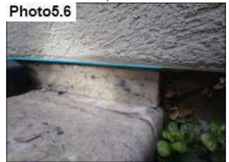
Stucco In Contact with Tile / No Modification Repaired
