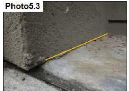
Stucco In Contact with Grade/ Apply a Kant Bead Repaired
