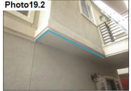
No Relief / No Modification but Maintain Sealants Above
