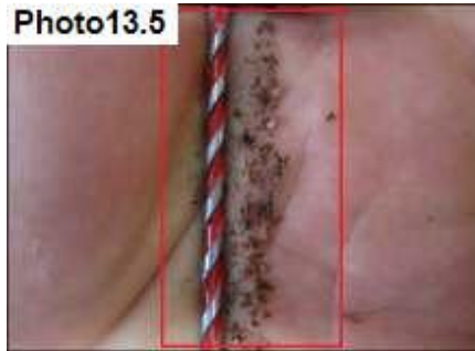
Substrate Damage / Assess, Repair & Install Relief
