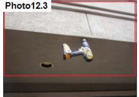
Substrate Damage / Assess, Repair & Install Relief
