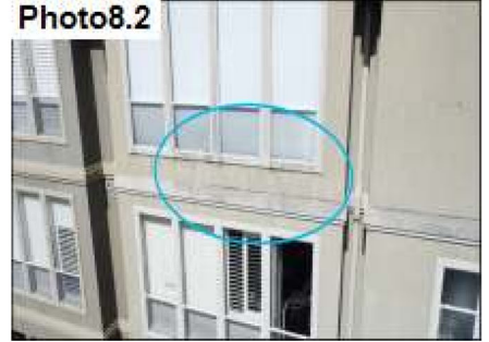
Run-off Stains / Clean (Aesthetic)
