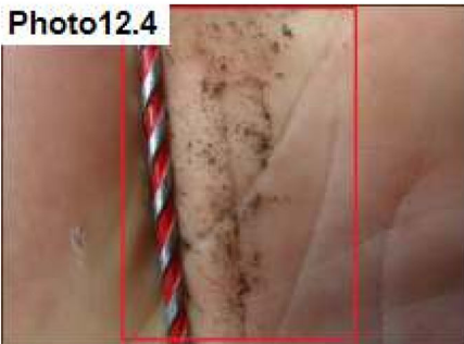
Substrate Damage / Assess, Repair & Install Relief
