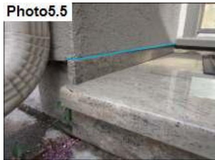
Stucco In Contact with Tile / No Modification Repaired
