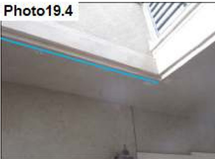
No Relief / No Modification but Maintain Sealants Above
