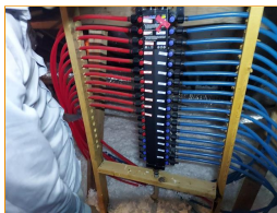
Water manifold in the attic area
