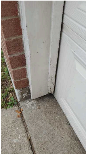
Damaged siding front side of house.
