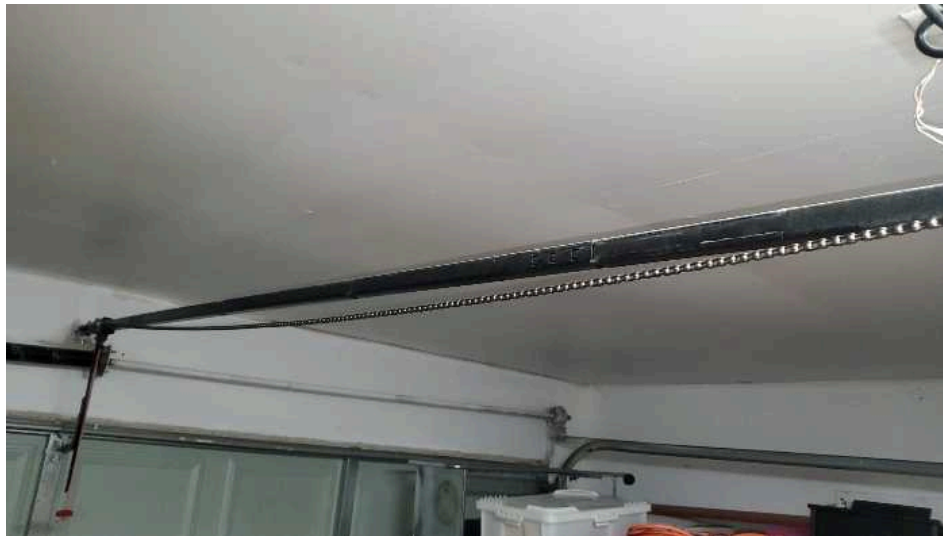
The drive chain is loose and in need of adjustments.
