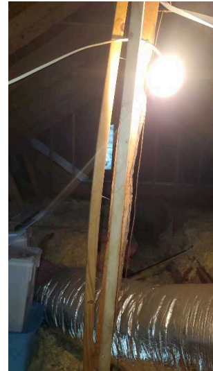
One or more of the rafter supports are loose.
