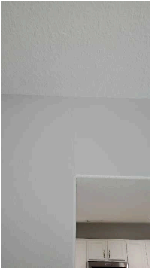
Tape Joint fractures were observed in one or more areas.
