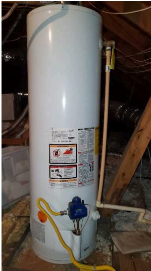
Picture of water heater
