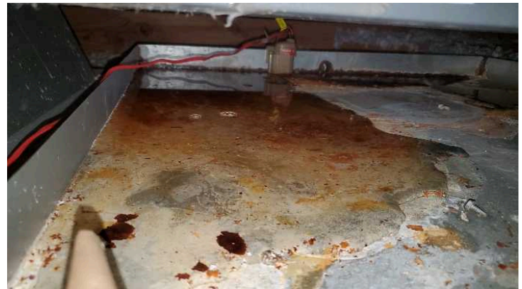
Rust and/or corrosion was noted in the condensate drip pan
