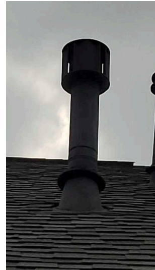
Furnace exhaust pipe
