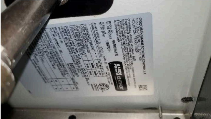
Furnace Data Tag
