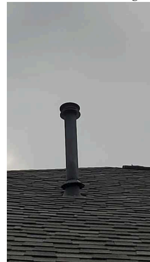
Water heater exhaust pipe
