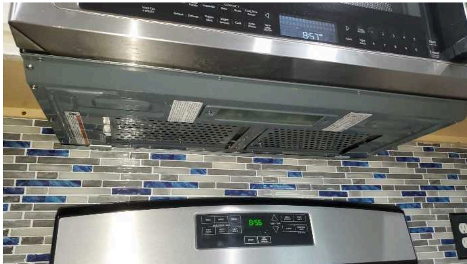
One or more of the grease screens are missing.
