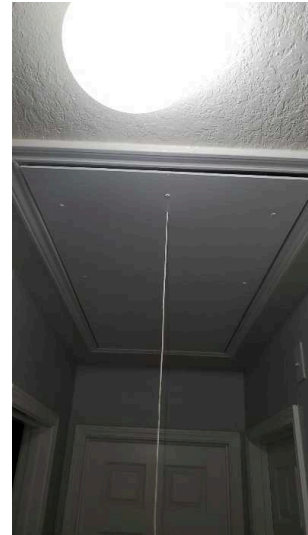
The attic ladder does not close properly and should be further evaluated
