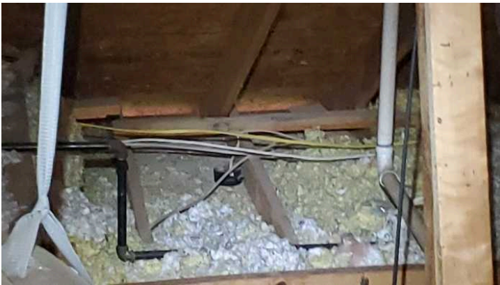
The attic insulation was observed to be low or compacted in areas. It is recommended that additional insulation be added to achieve a minimum of R-30.
