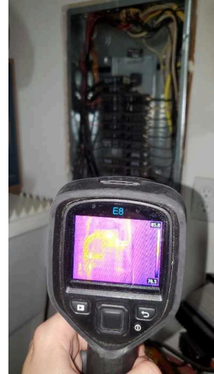
Thermal imaging camera used to detect over heating electrical components. No issues.
