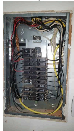
Picture of breakers
