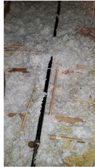
Water lines in the attic.
