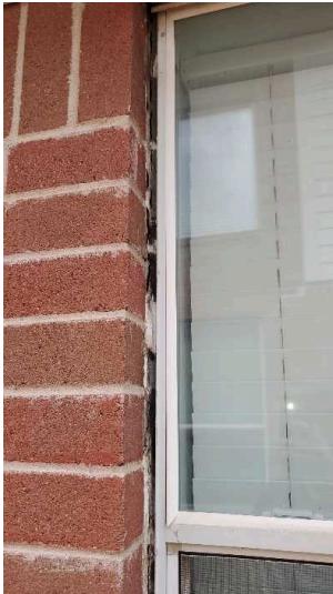
Elastomeric caulking improvements are recommended between the exterior veneer and the window frames in one or more areas of the home.
