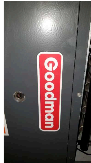
Furnace brand name
