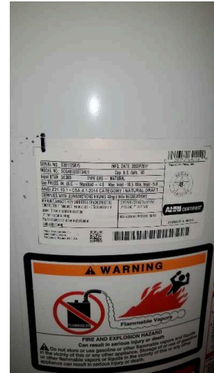
Water heater data tag
