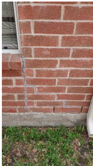
Right side. Brick separation.
