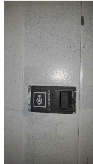
Electrical service panel brand name.
