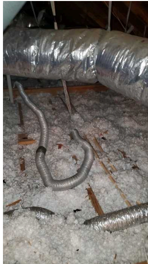
The bathroom exhaust fan noted to be terminated in the attic space.
