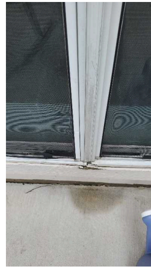
Damaged siding back side of house.
