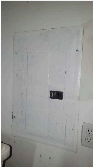
Picture of electrical service panel.
