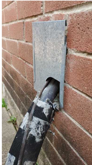
Refrigerant lines noted with damaged / missing insulation at the Condensing Unit.
