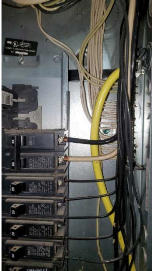
Hot white wires in the panel.
