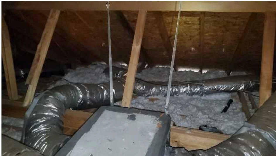
Ductwork in attic space was observed to be sagging and/or kinked and is not supported at {4'} spacing as recommended
