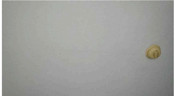
Tape Joint fractures were observed in one or more areas.
