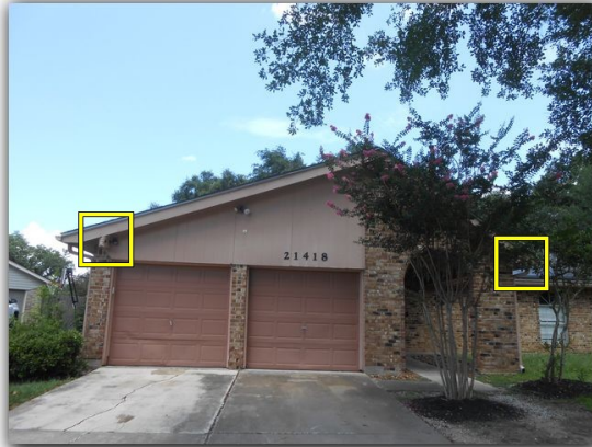
The decorative beam is missing at the peak at the front of the home exposing an opening into the attic space. This is an entry point of water and pests.
