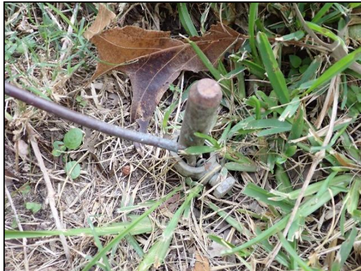
23. Copper - ground rods
