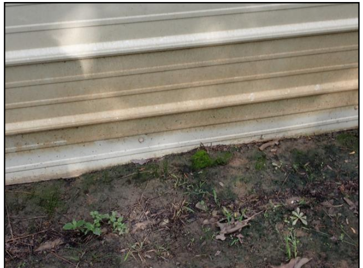
14. Too close to grade
