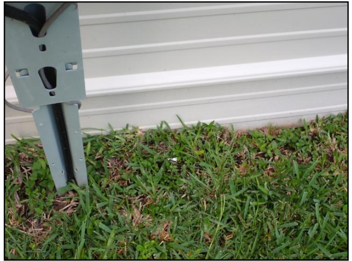
12. Too close to grade
