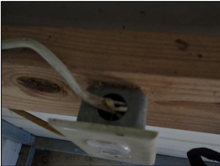
27. Not well secured
