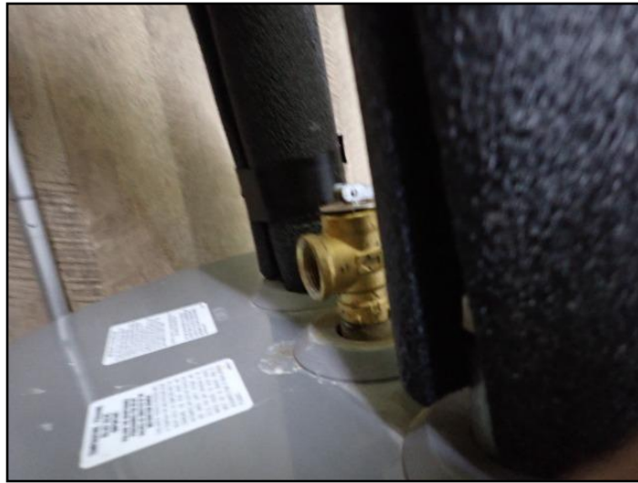
50. Discharge tube missing
