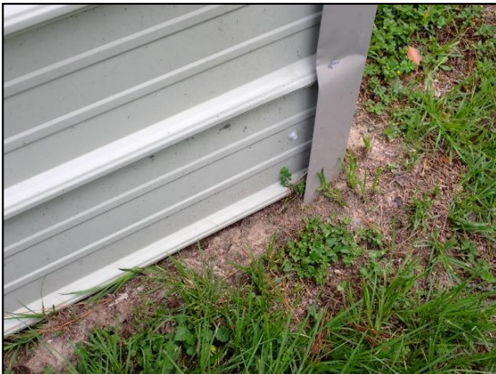
13. Too close to grade
