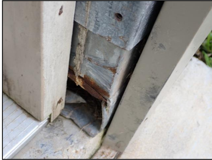
10. Loose or missing pieces
