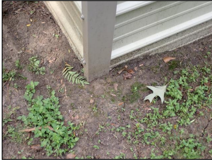
15. Too close to grade
