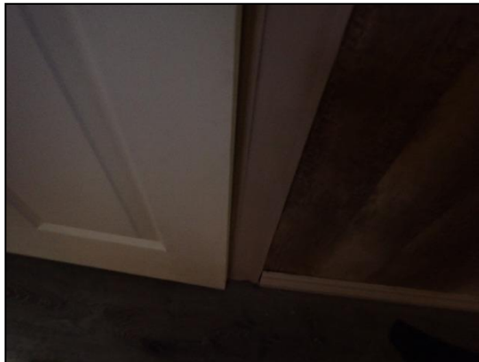
56. Loose or poor fit
