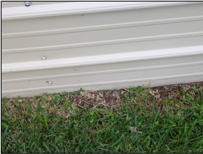
11. Too close to grade
