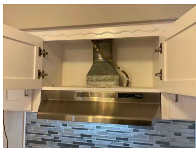
Range Exhaust: vents to the exterior
