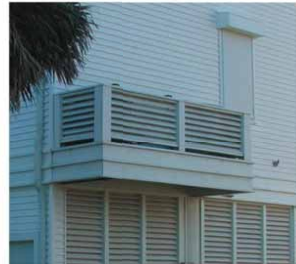
Screened AC unit
