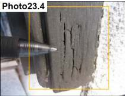
Wood Rot on Door Trim / Repair
