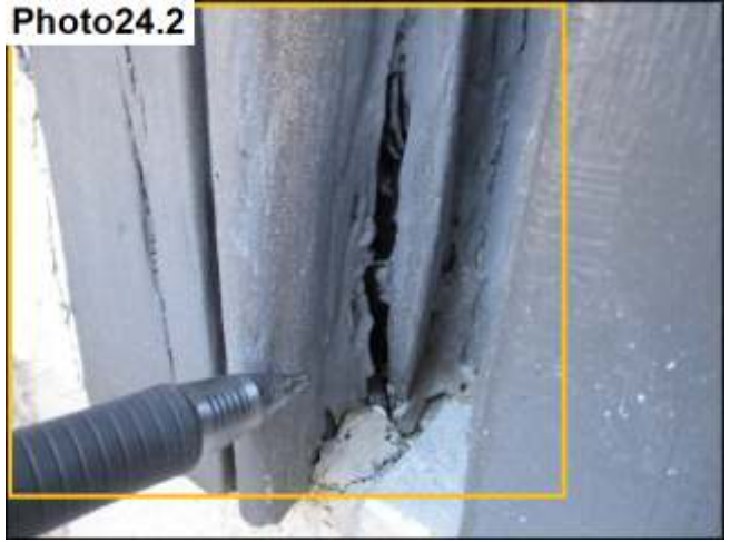
Wood Rot on Door Trim / Repair
