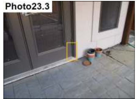
Wood Rot on Door Trim / Repair
