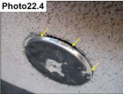
Penetration Sealants / Seal
