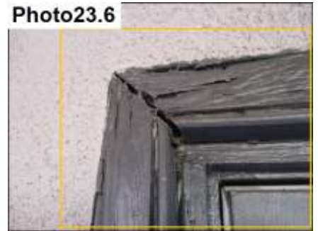
Wood Rot on Door Trim / Repair
