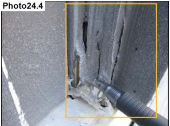
Wood Rot on Door Trim / Repair
