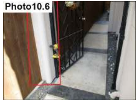
Damaged Entryway / Assess And Repair
