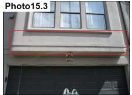
Substrate Damage / Assess, Repair & Install Relief
