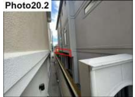
Damage / Core Sample & Repair As Needed
