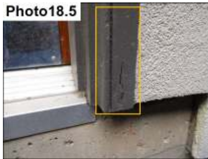
Wood Rot on Door Trim / Repair
