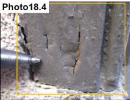
Wood Rot on Door Trim / Repair
