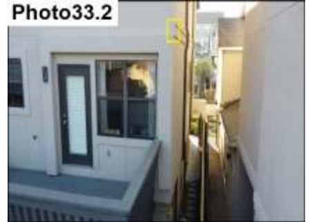
Cracks / Seal or Paint (Aesthetic)
