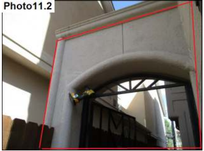
Damaged Entryway / Assess And Repair
