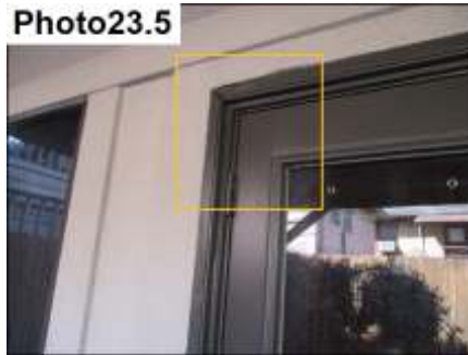
Wood Rot on Door Trim / Repair
