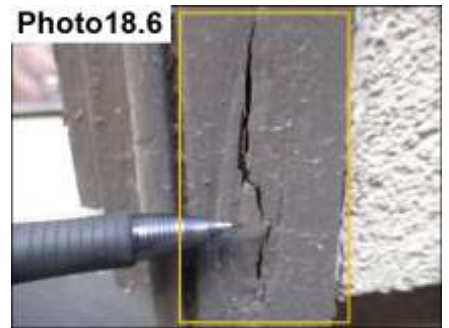
Wood Rot on Door Trim / Repair
