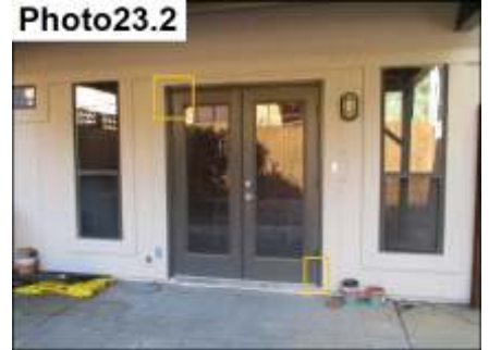
Wood Rot on Door Trim / Repair
