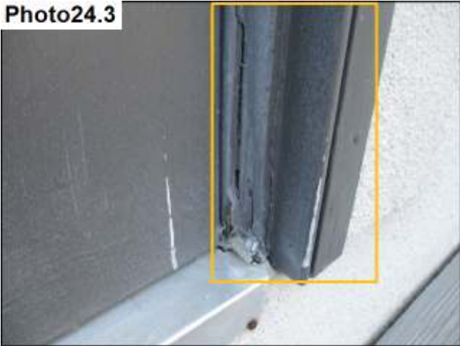
Wood Rot on Door Trim / Repair
