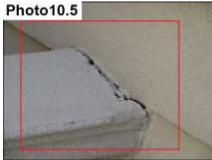
Damaged Entryway / Assess And Repair
