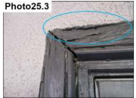
Missing Door Head Flashing / Install
