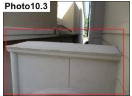
Damaged Entryway / Assess And Repair
