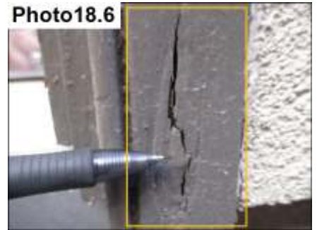
Wood Rot on Door Trim / Repair
