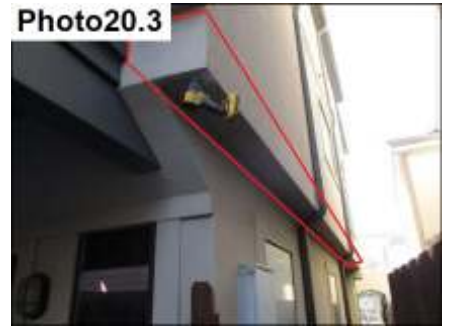
Damage / Core Sample & Repair As Needed
