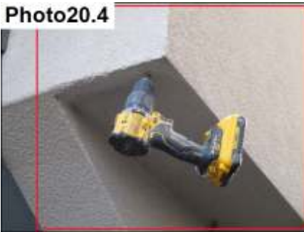
Damage / Core Sample & Repair As Needed
