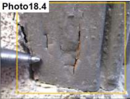
Wood Rot on Door Trim / Repair
