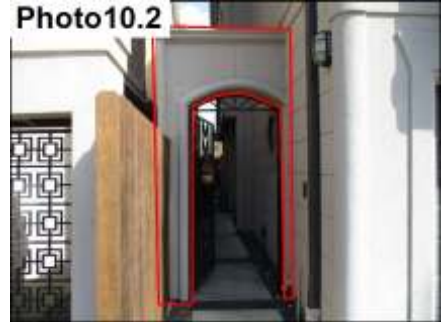
Damaged Entryway / Assess And Repair
