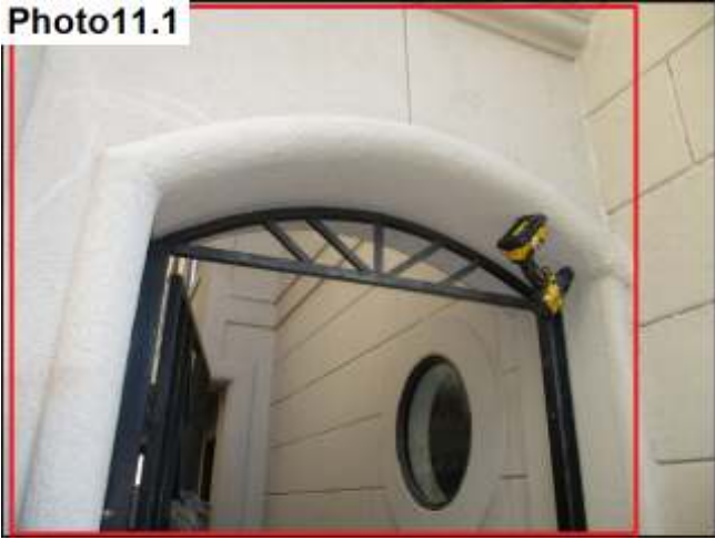
Damaged Entryway / Assess And Repair
