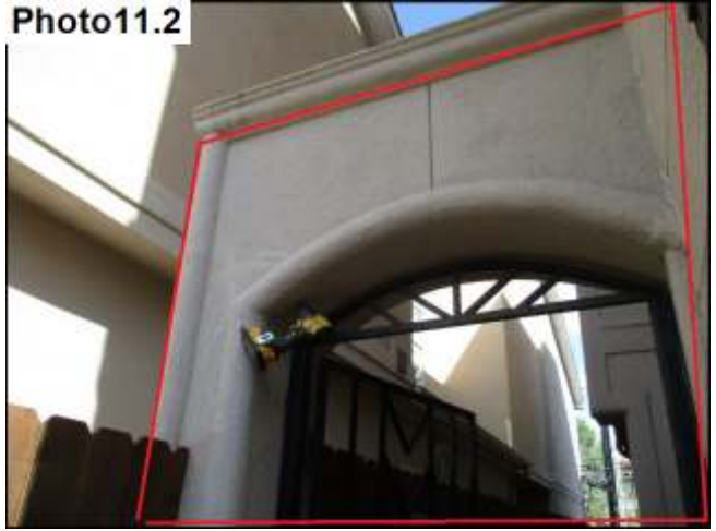
Damaged Entryway / Assess And Repair
