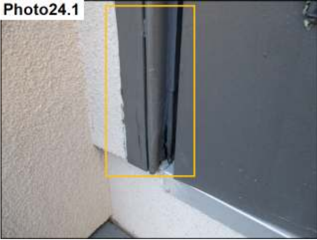
Wood Rot on Door Trim / Repair
