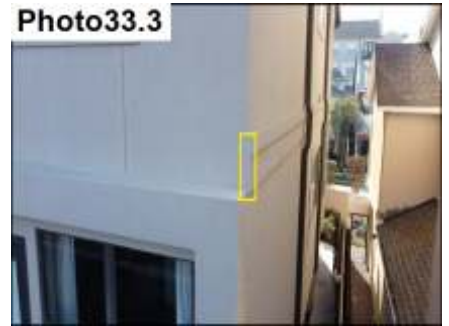
Cracks / Seal or Paint (Aesthetic)
