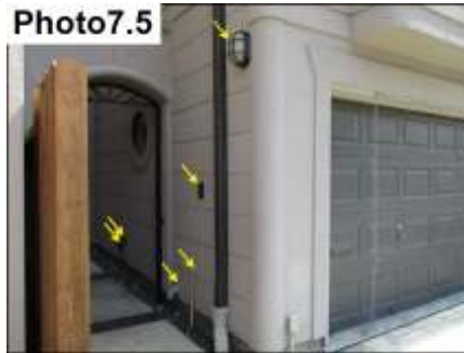
Penetration Sealants / Seal
