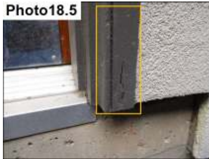
Wood Rot on Door Trim / Repair
