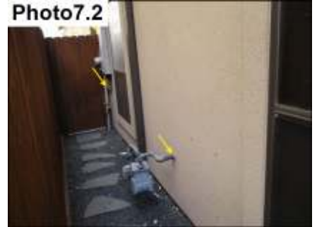
Penetration Sealants / Seal
