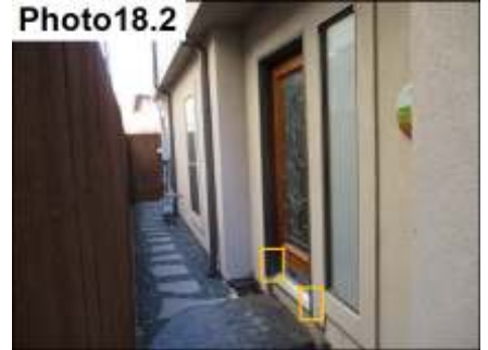
Wood Rot on Door Trim / Repair
