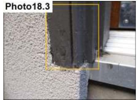
Wood Rot on Door Trim / Repair
