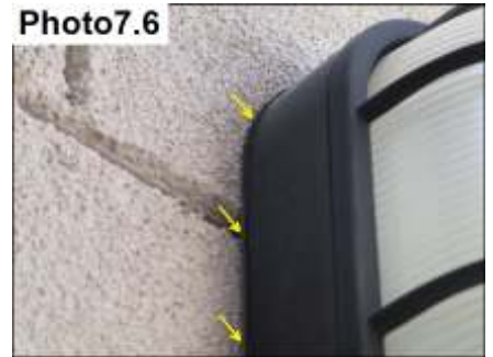
Penetration Sealants / Seal
