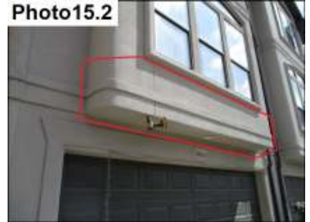
Substrate Damage / Assess, Repair & Install Relief
