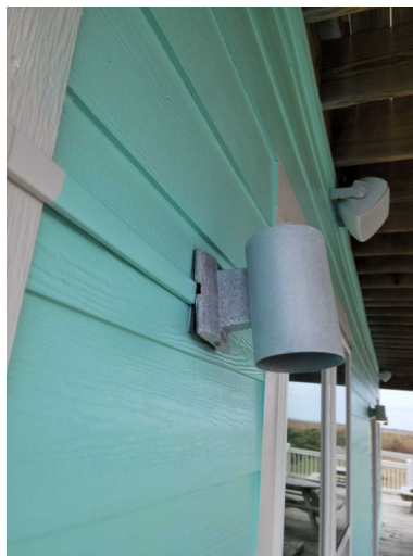
All exterior lights
