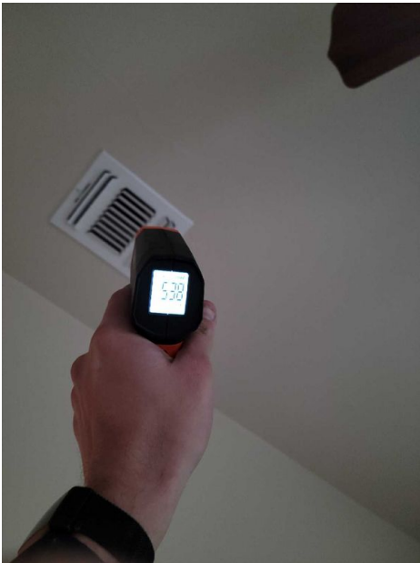
Photo(s) of return(s): Returns deliver air back to HVAC air handler, furnace, and evaporator.
