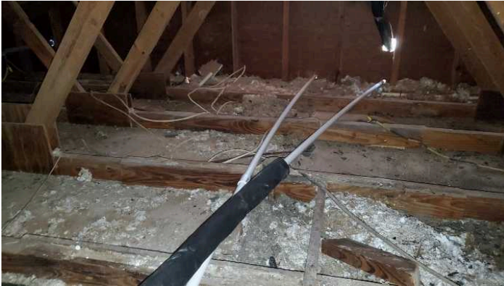
The hallway and main bedrooms do not have insulation installed in the attic space of above them.
