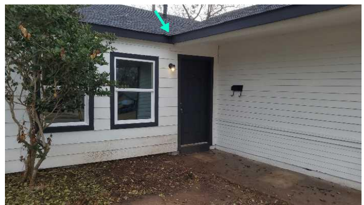
Recommend adding a gutter above the front entryway to prevent water from splashing mud onto the walk way.
