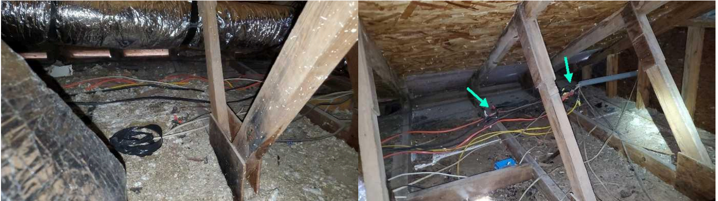
The wire connections to the main electrical panel have been spliced in the attic. These splices should be contained in a junction box or made inside the electrical panel.
