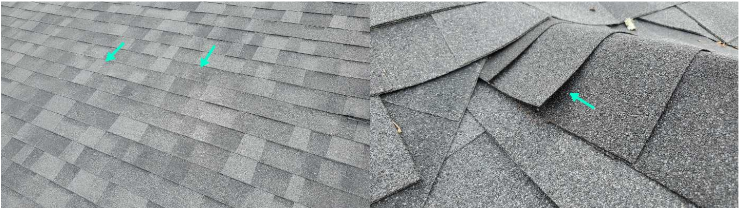
The singles at the start of the front ridge cap are not sealed at the edges.
