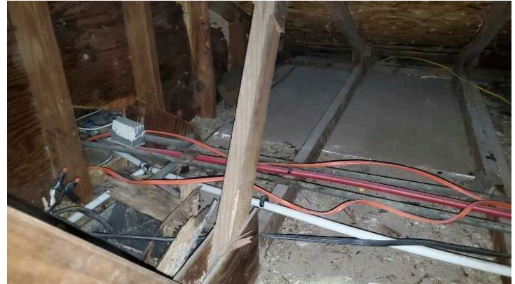
PEX plumbing lines in the attic.
