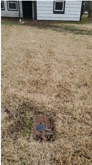
Water meter in front of the house with shut off valve.
