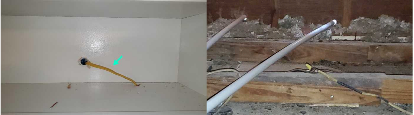
The wiring for the oven vent hood should be protected from damage with conduit.
