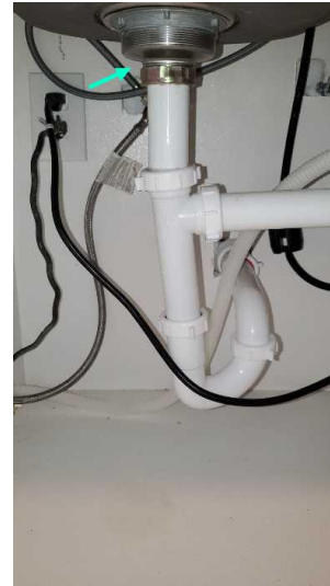
Leak at the kitchen sink to drain connection.
