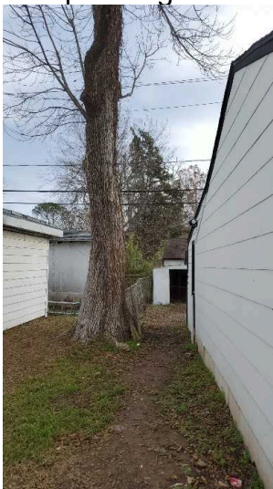
Recommend removing trees that are within 6ft of the house as they can cause foundation movement over time from root growth and moisture build up next to the house.
