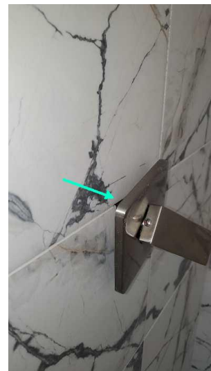
The main shower faucet bezel is loose.
