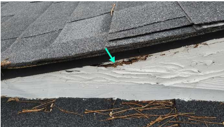
Damaged fascia board on the roof to wall connection on the left side of the house.
