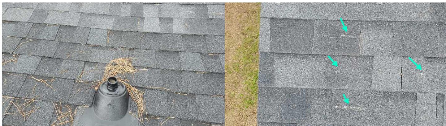
Current standards mandate all plumbing vents stacks extend a minimum of {6"} above the roof.
