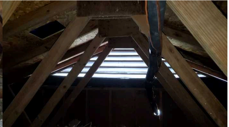
The gable vent is missing a screen to prevent pest entry.
