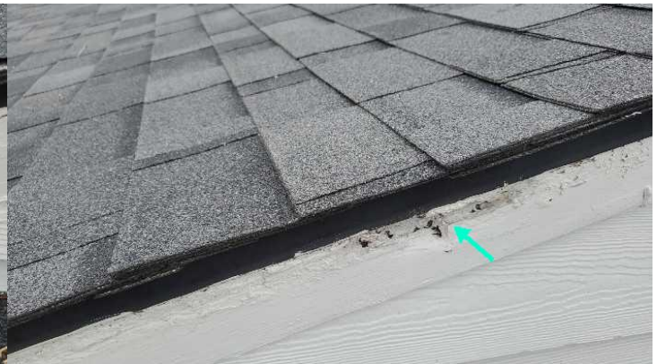
Damaged fascia board on the roof to wall connection on the left side of the house.
