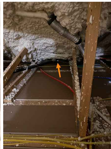
Not sealed at right side wall eaves
