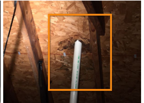
Sewer vent pipe at the center of the attic
