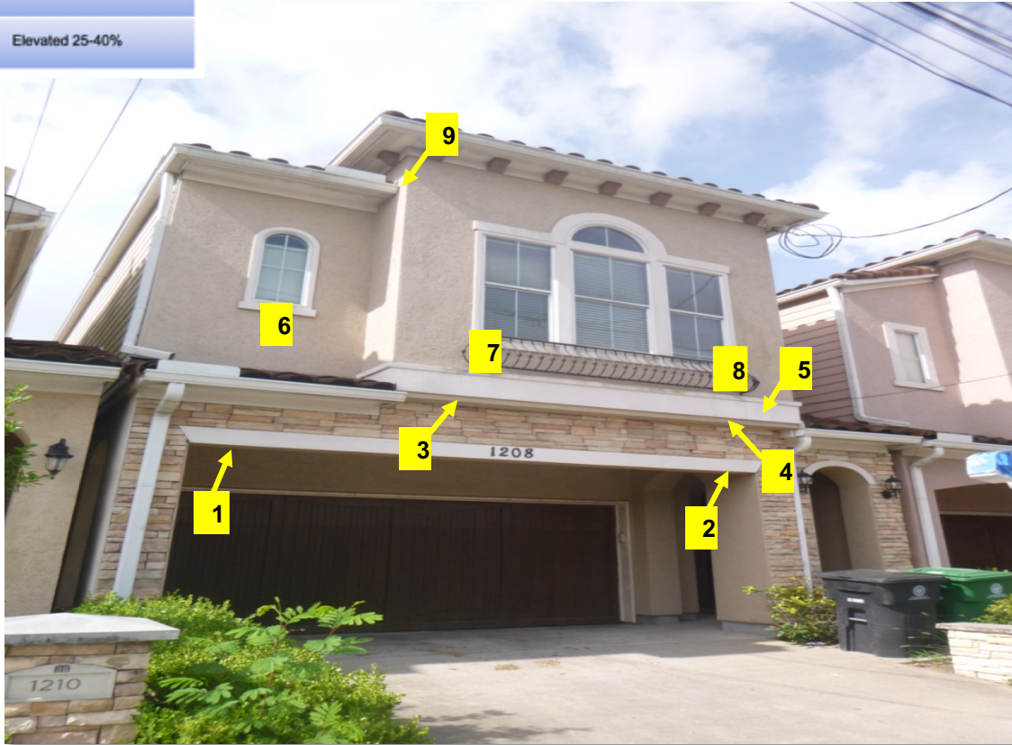
Note: Delmhorst 2100 Moisture Probe Reading. Probes Range from 6%-40%
