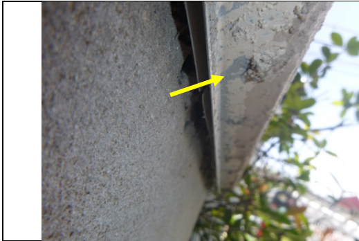
The base of the stucco walls terminates with a weep screed and proper clearance above grade. This is a favorable condition.
