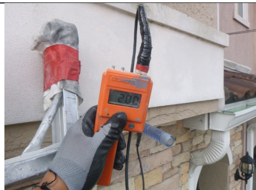
Mid moisture and firm substrate (possible framing) at the crack along the overhang at the time of inspection.
