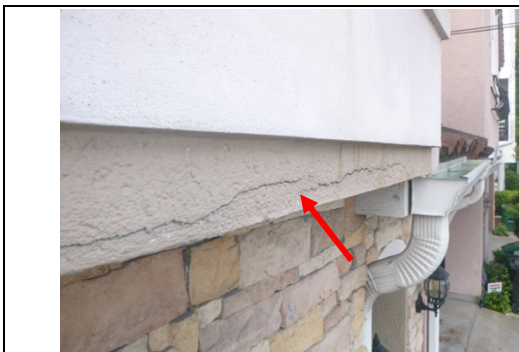
Severe cracking noted along the front right corner of the overhang. This can lead to moisture intrusion if not sealed/repaired.
