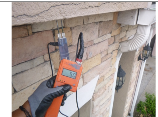
Low moisture and firm substrate (possible framing) below the front elevation overhang at the time of inspection. This is favorable.
