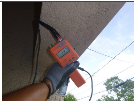
Low moisture and firm substrate (possible framing) below the front elevation overhang at the time of inspection. This is favorable.
