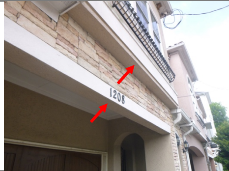
The front overhangs are closed in with stucco & have no drainage accessory. This can lead to trapped moisture and possible future damages. To help prevent future issues it is suggested to install drainage accessories at all locations noted with this deficiency.
