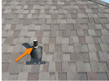
Right Side- needs to be fully painted
