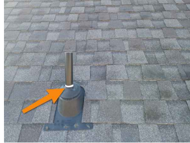
Left Side- needs to be fully painted
