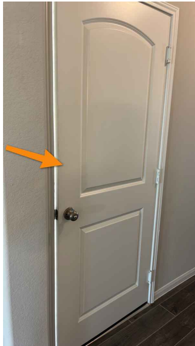
Garage entry door- does not fully close
