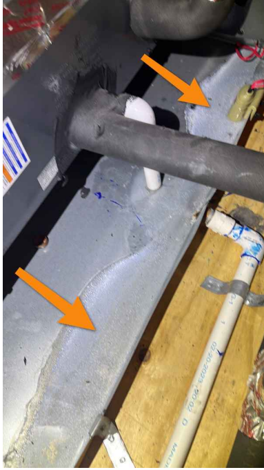
Standing water in pan
