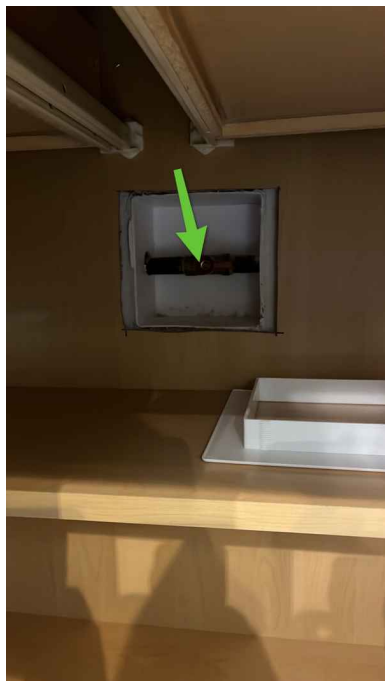
Gas shut off valve
