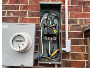
Service panel - Cover off
