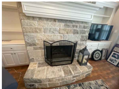
Photo of Fireplace Ignited:
