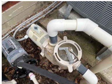
Water feature pump
