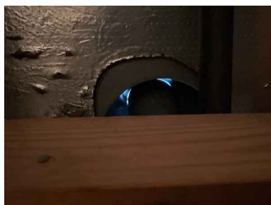
Example Water heater flue
