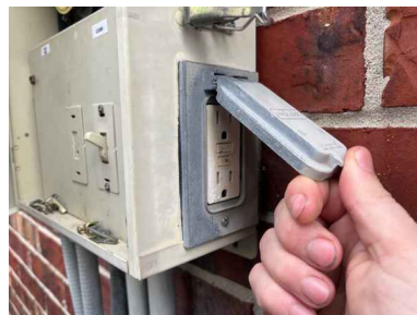
Pool light GFCI
