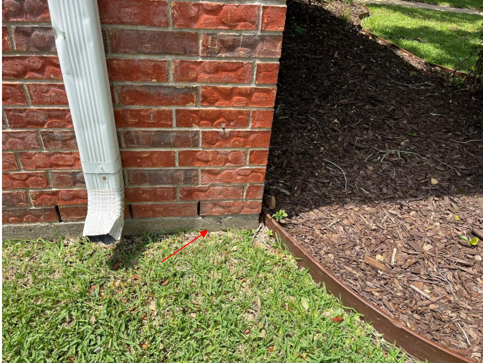
Photograph 3: Non-structural corner cracking.
