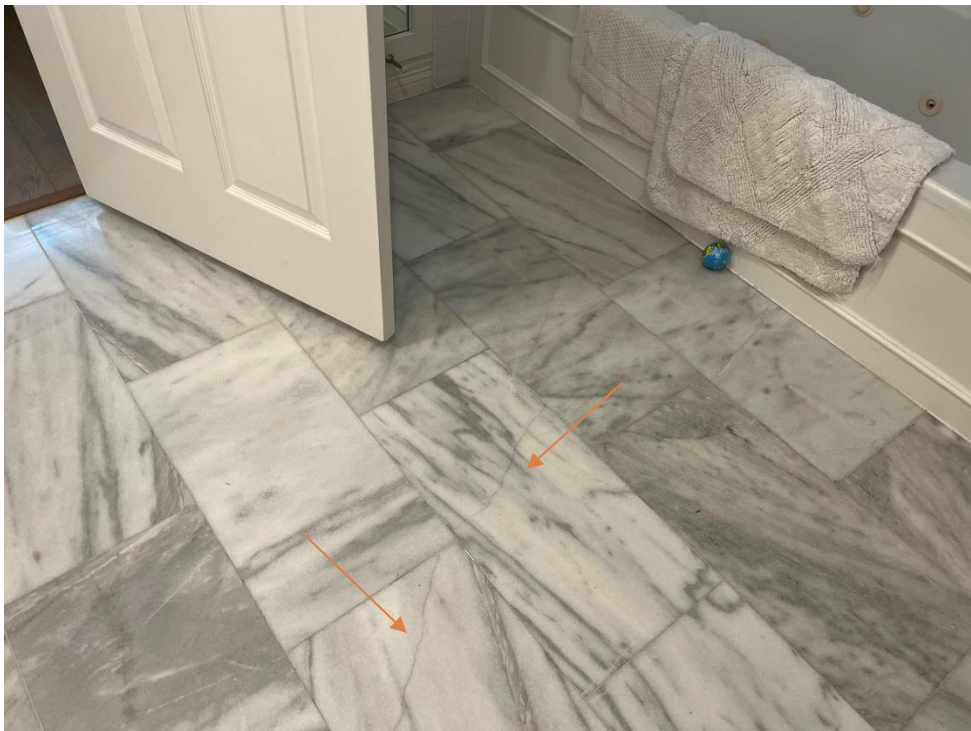
Photograph 4: Cracks in master bathroom tile
