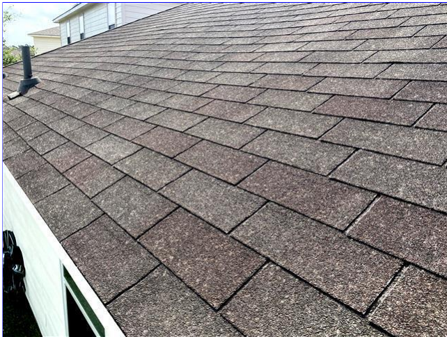
C. Item 2(Picture) Hail damage
