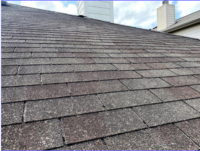
C. Item 1(Picture) Hail Damage
