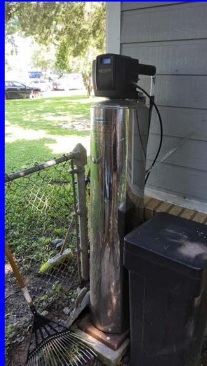
water conditioner back right (not inspected)
