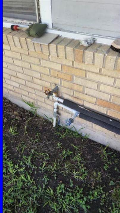
water main shut off out front
