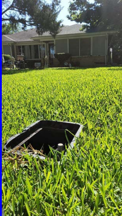
water meter front right by street
