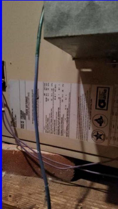
furnace data plate
