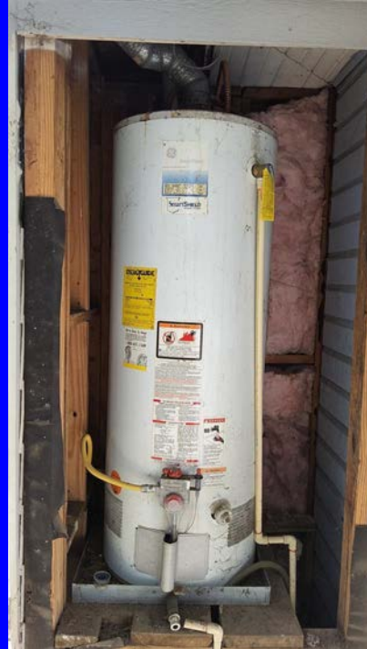
50gal gas water heater in utility room
