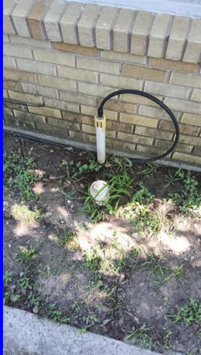
plumbing main clean out back right
