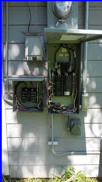
150amp main service panel and sub panel backyard
