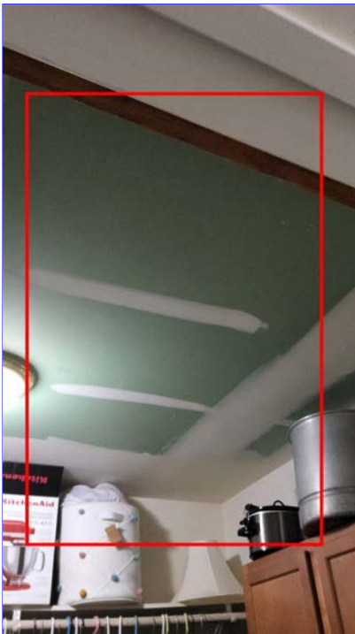
F. Item 19 (Picture) utility room
