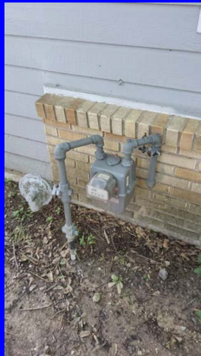
gas meter back left
