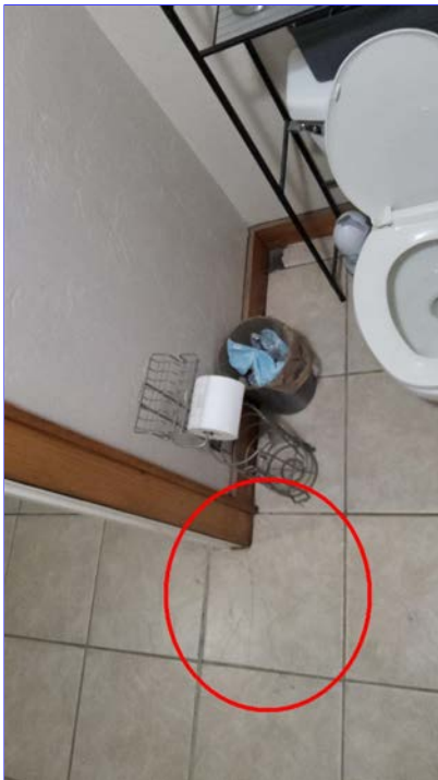
F. Item 3 (Picture) utility room
