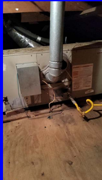
gas furnace in attic
