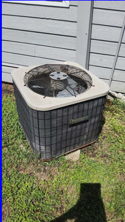
HVAC system backyard
