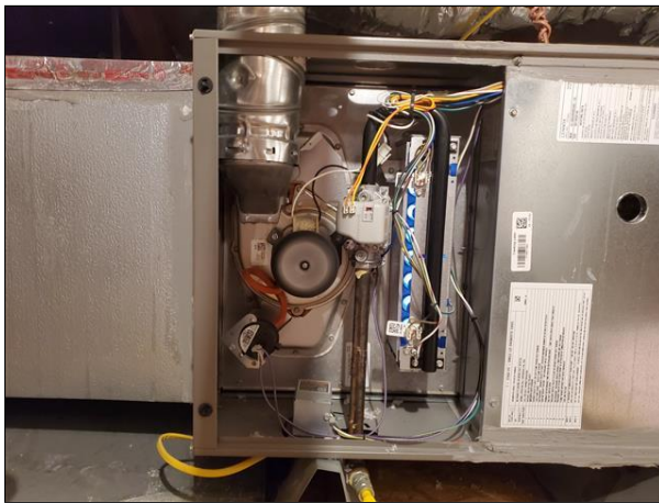
Furnace in operation
