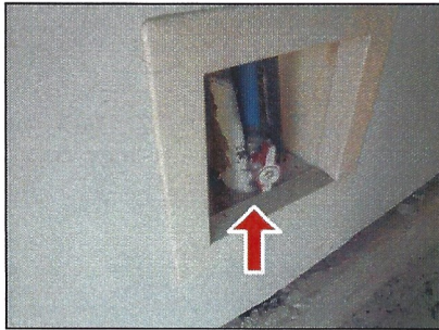
Main water shut off located within garage.
