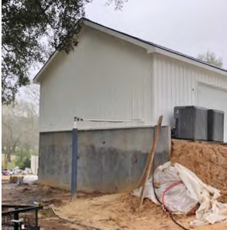
View of West and South sides of garage showing A/C condenser units. (02-07-2019)
