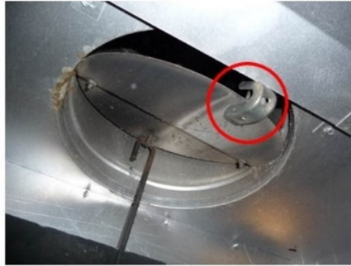
HEI file photo showing c-clamp in metal fireplace
