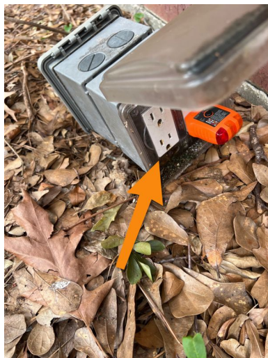
Loose Conduit and No Power - Front Exterior
