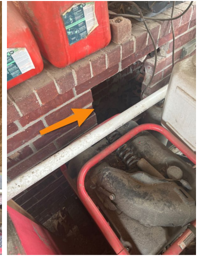
Manual Cut Out at Gazebo
