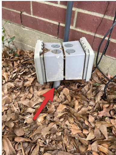
Loose - Front Exterior
