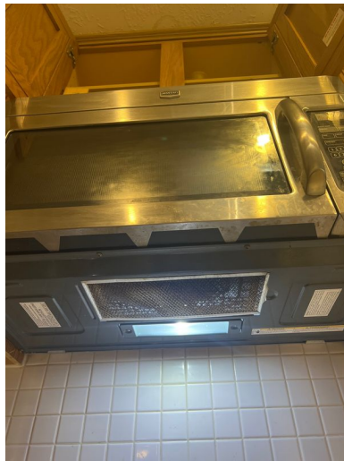
Exhaust hood recirculates :
