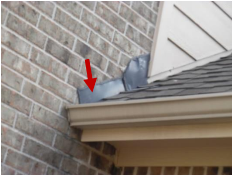
Kick out flashing missing
