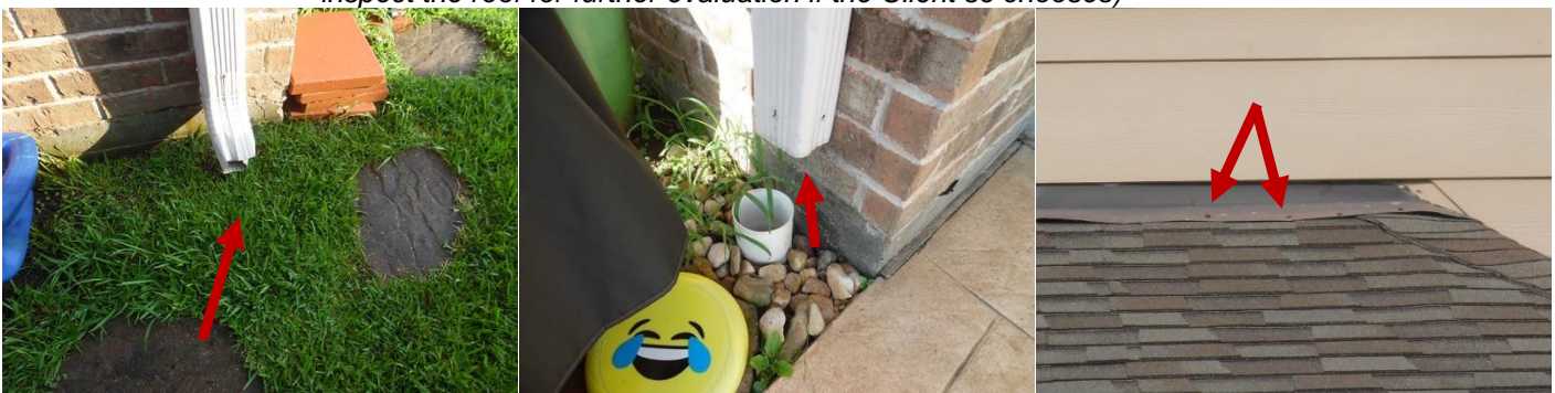
Splash block missing
