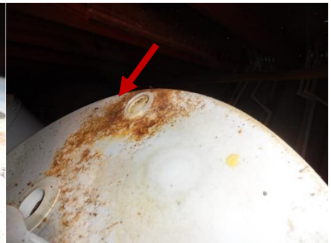
rust on top of the left unit
