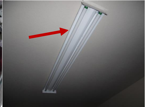
lens cover missing
