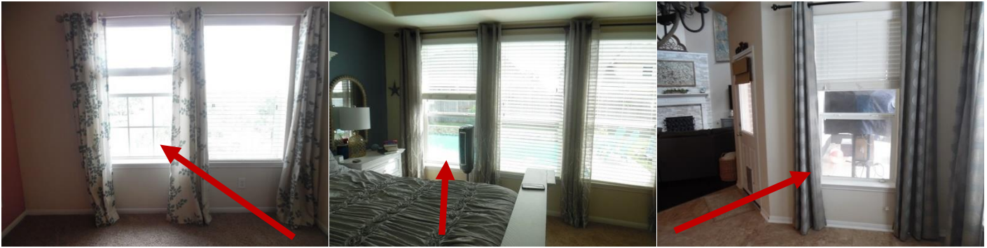
Windows were stuck and would not open
