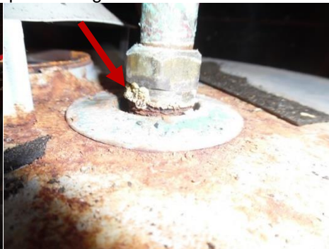
rust / corrosion on right unit
