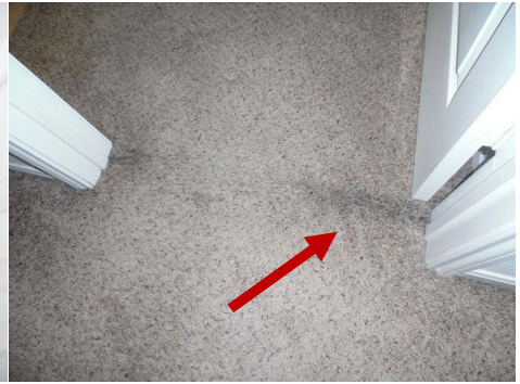
carpet stains under bedroom doors
