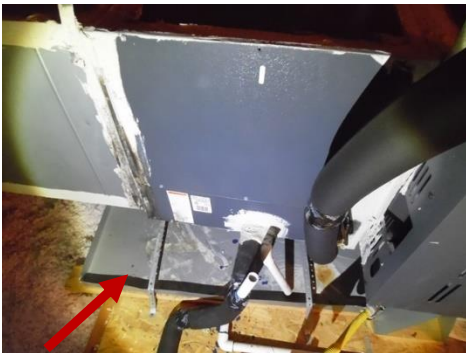
No float switch in pan
