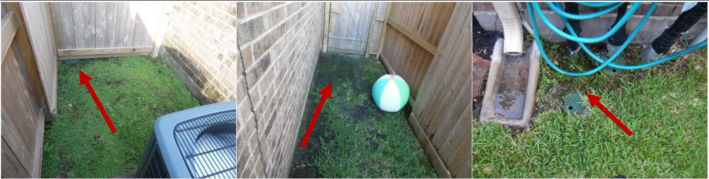
Possible ponding areas
