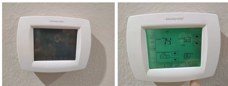
Inspector used new batteries for inspection only
