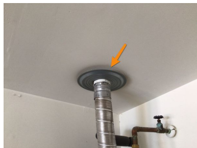
Loose ceiling collar
