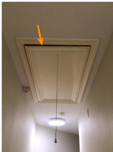
Does not seal
