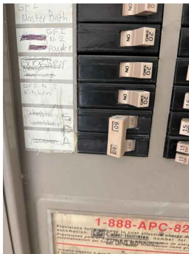
60 amp breaker not functioning
