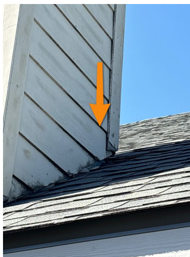
Chimney (damaged siding)
