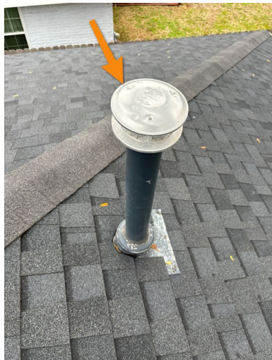
Water heater vent
