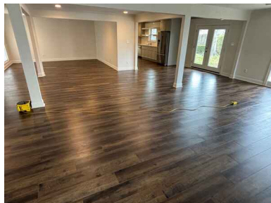
Living room (floor slope)
