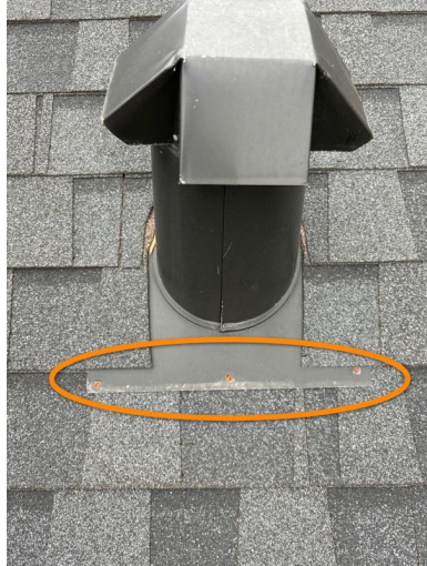
Master bathroom exhaust vent
