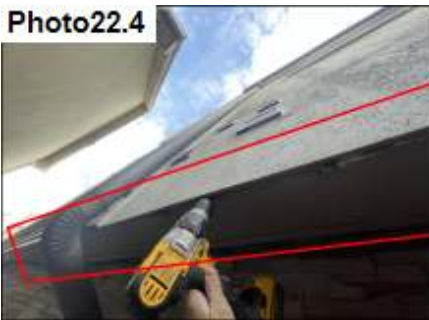
Substrate Damage / Assess, Repair & Modify as Needed
