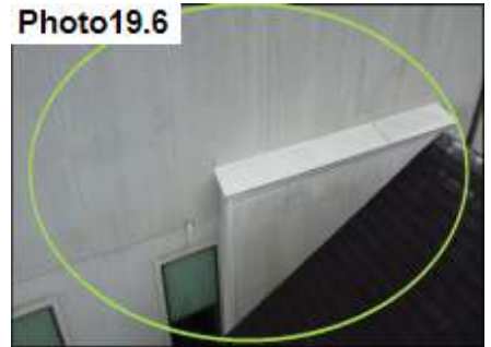
Mildew Stains / Clean (Aesthetic Concern)
