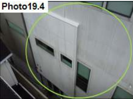
Mildew Stains / Clean (Aesthetic Concern)
