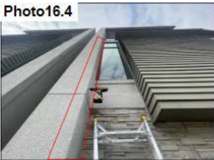
Substrate Damage / Assess, Core Sample & Repair as Needed
