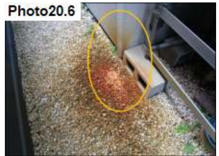
Rust Stains / Clean and Paint as Needed
