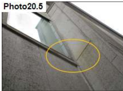
Rust Stains / Clean and Paint as Needed
