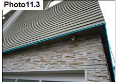
Obstructed Relief / Clean Out
