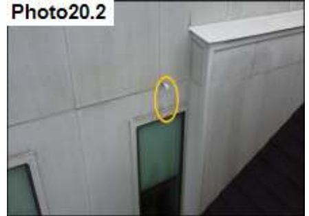
Rust Stains / Clean and Paint as Needed
