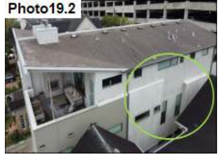
Mildew Stains / Clean (Aesthetic Concern)
