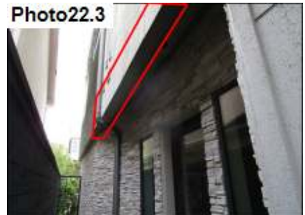
Substrate Damage / Assess, Repair & Modify as Needed
