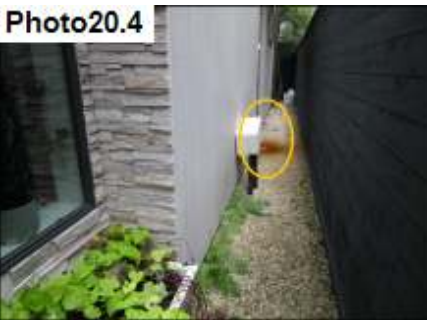
Rust Stains / Clean and Paint as Needed
