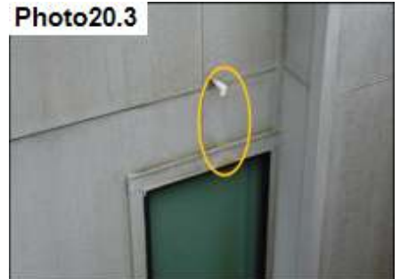
Rust Stains / Clean and Paint as Needed
