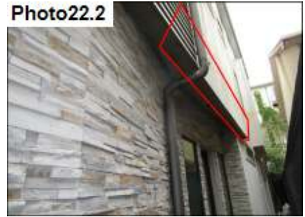
Substrate Damage / Assess, Repair & Modify as Needed
