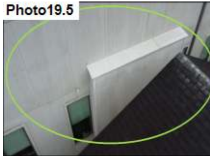
Mildew Stains / Clean (Aesthetic Concern)
