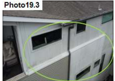
Mildew Stains / Clean (Aesthetic Concern)
