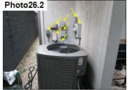
Penetration Sealants / Seal
