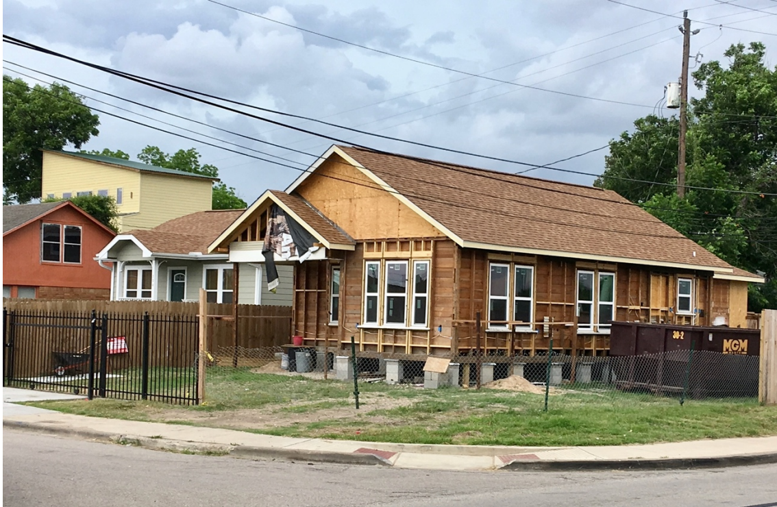
The exterior siding was removed so that new wiring and bat insulation could be installed. Plywood sheathing and cement board siding was installed. Foam insulation was sprayed under the floor and in the back addition (former breezeway ceiling). Central HVAC system installed.
