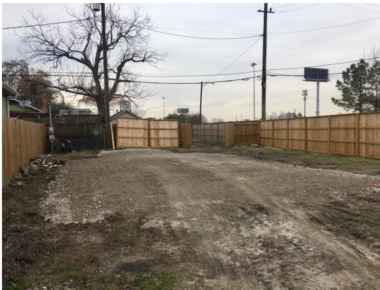
502 Dell Ct foundation site was prepared by replacing topsoil with crushed concrete that was leveled and machine compacted.
