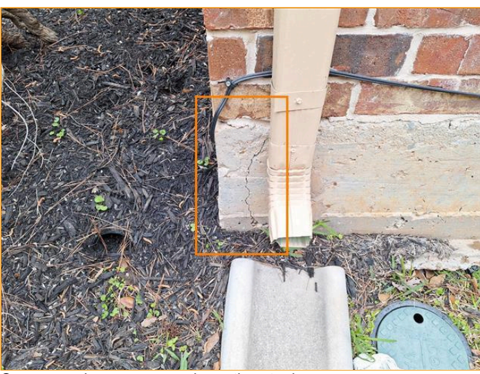
Corner cracks common and non threatening
