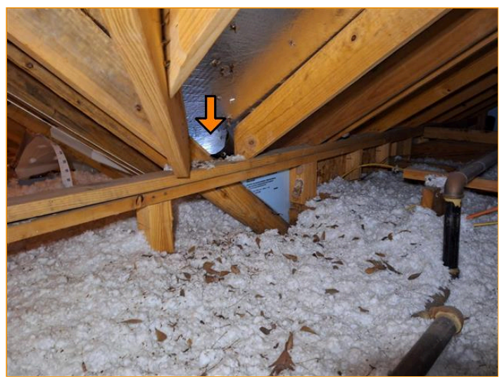
Opening appears to allow debris in
