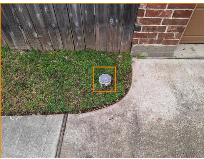
Main clean out
