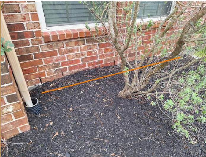
Recommend exposing foundation
