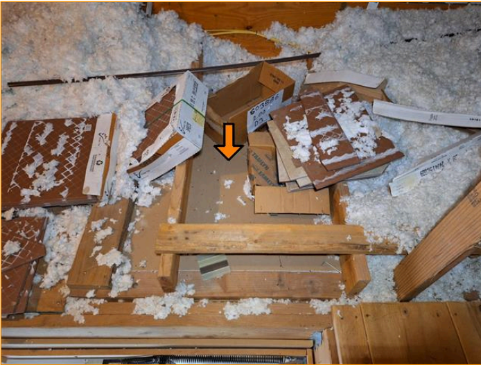
Recommend filling in insulation voids
