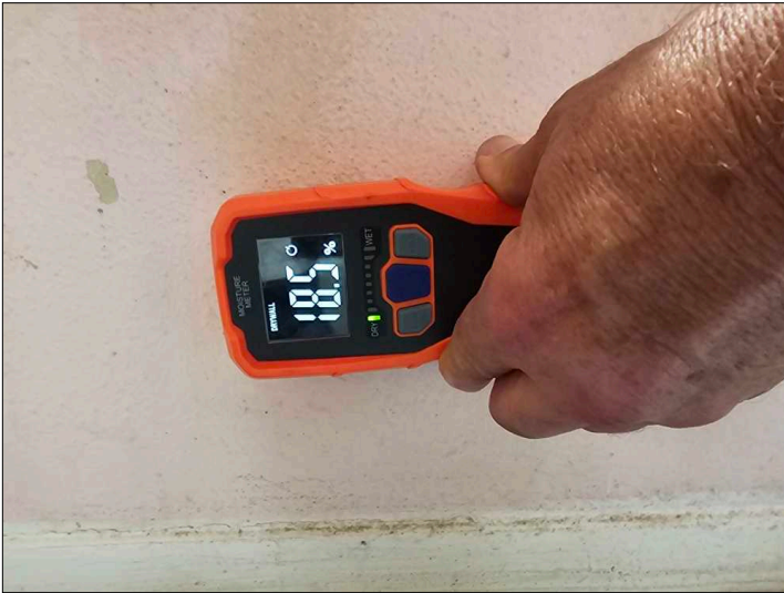
Checked water stain on the walls with a moisture meter and found to be at higher than normal moisture level. Unable to determine condition of the underlying materials. Mainly at - primary bedroom
