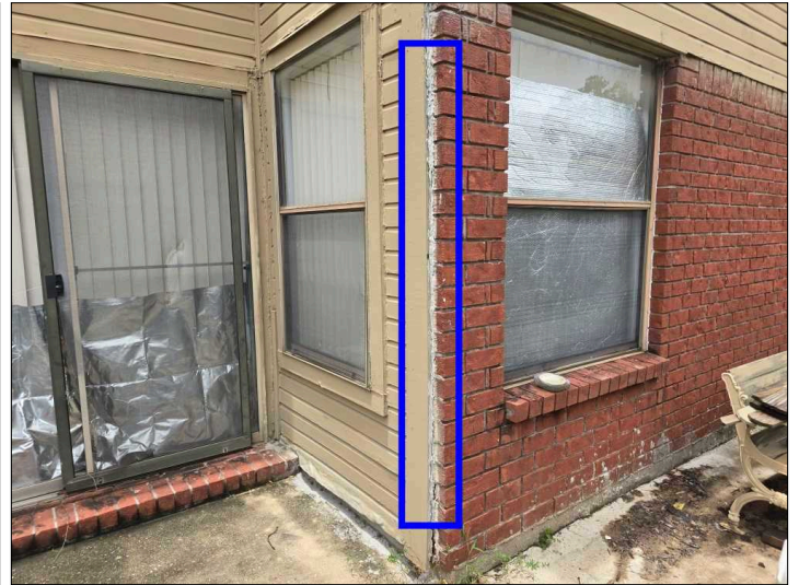
Recommend sealing between the trim and brickwork to help prevent water penetration. Mainly at - right
