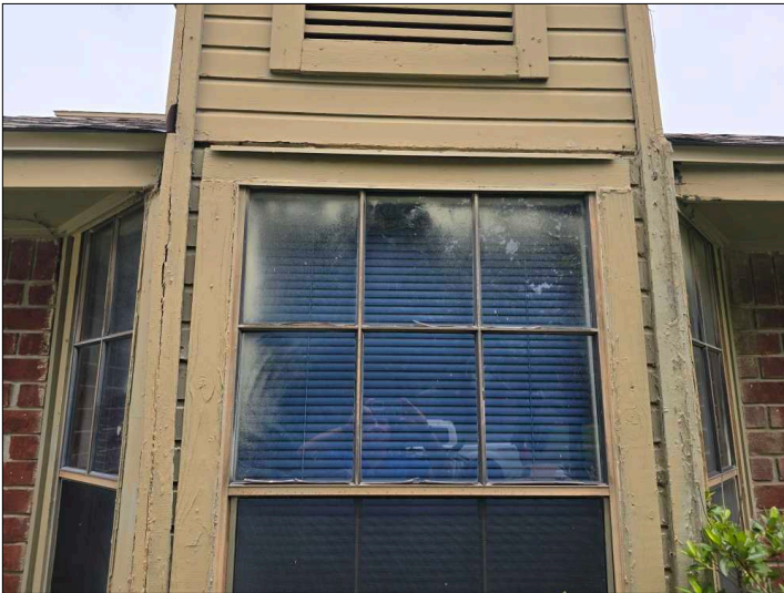
Deterioration was noted at the trim, recommend replacing all deteriorated trim. Unable to determine the condition of the underlying materials. Mainly at - front
