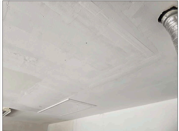
There is evidence of previous patch work and or painting on the interior finishes. This condition may limit the inspector's visual observations and ability to render accurate opinions as to the performance of the structure. Recommend contacting homeowner for more information. Mainly at - garage
