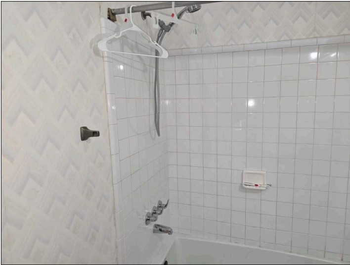
Overview of Plumbing Fixture(s) in Operation.
