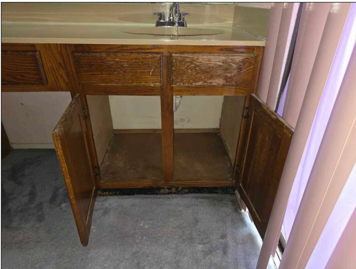
Overview of Plumbing Fixture(s) in Operation.
