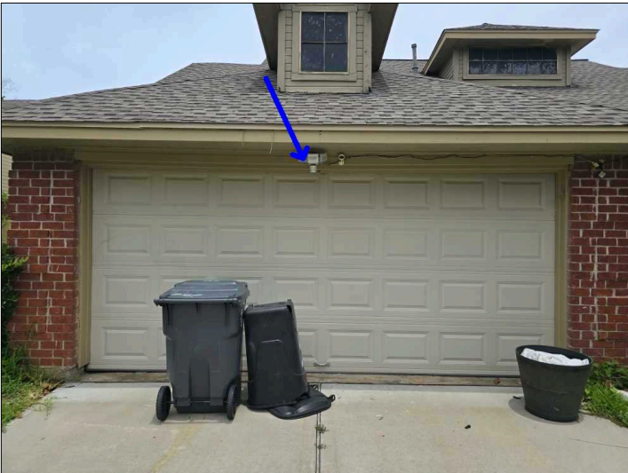
The header is showing signs of sagging over the garage. This is often caused by improper support over the garage door. If this is minor settlement and home is older this may have settled and is likely not to be a major problem in the future, however if there is substantial movement it is recommended that this be looked at by a contractor or structural engineer for further evaluation and repairs as needed.
