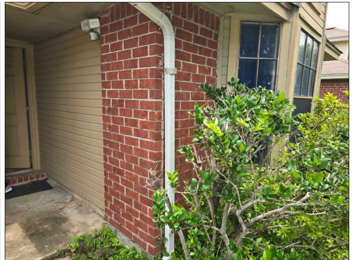
The downspout on the gutter was loose from the wall. Mainly at - front
