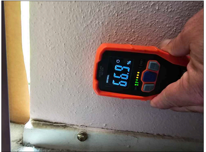
Checked water stain with a moisture meter and found it to be at a high moisture level. Unable to determine condition of the underlying materials. Mainly at - primary bathroom
