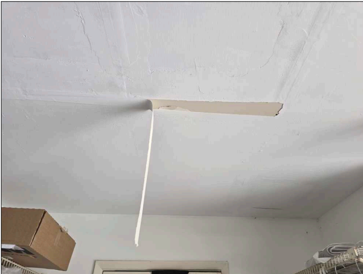
Settlement cracks were noted at the tape joint in the drywall. Mainly at - garage
