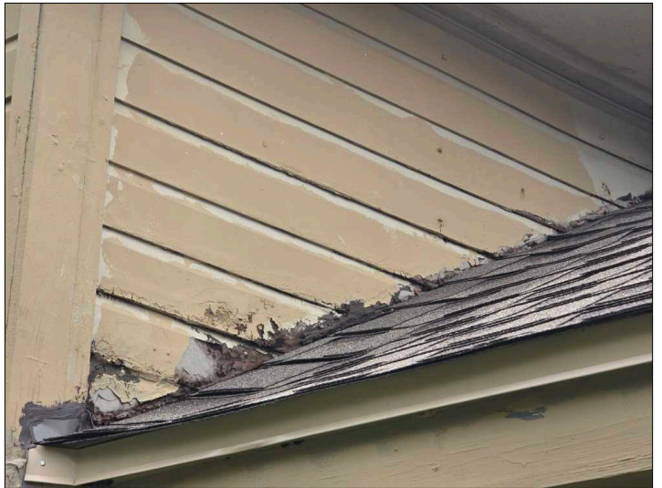
The siding is closer than recommended or in contact with the roof. It is recommended that there be a separation to help prevent water from wicking up into the siding material causing deterioration.
