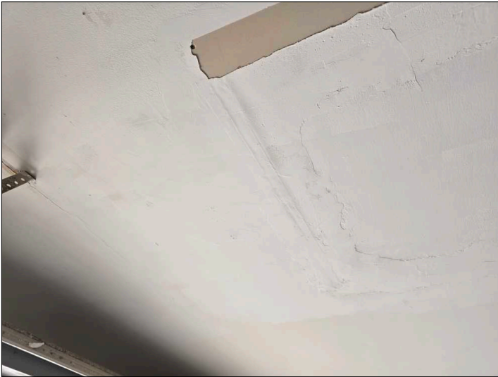
There is evidence of previous patch work and or painting on the interior finishes. This condition may limit the inspector's visual observations and ability to render accurate opinions as to the performance of the structure. Recommend contacting homeowner for more information. Mainly at - garage
