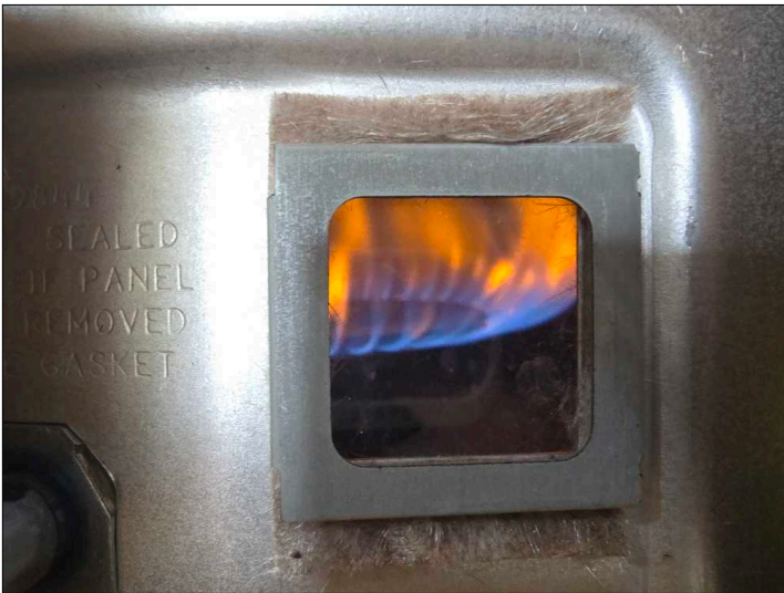
Overview of water heater burner compartment
