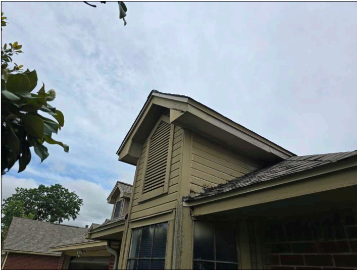
Deterioration was noted at the trim, recommend replacing all deteriorated trim. Unable to determine the condition of the underlying materials. Mainly at - front
