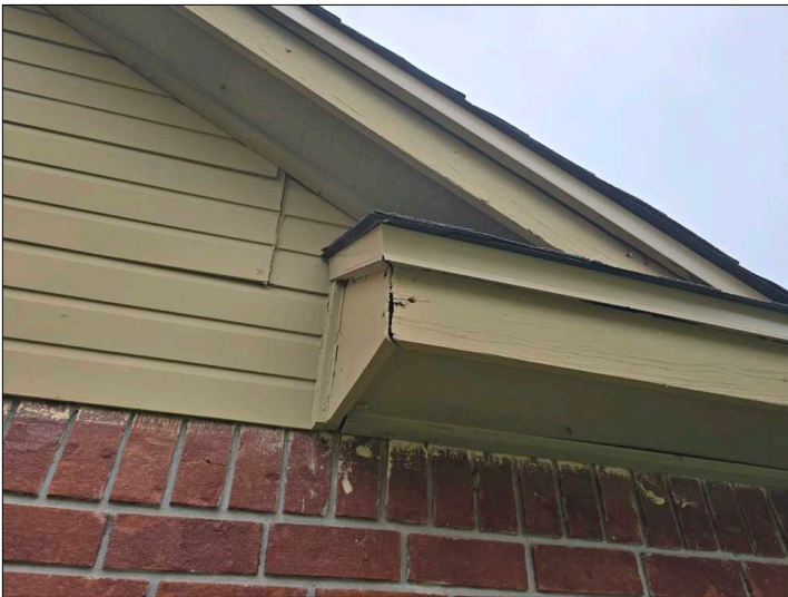
Deterioration was noted at the trim, recommend replacing all deteriorated trim. Unable to determine the condition of the underlying materials. Mainly at - left
