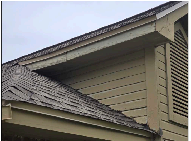
The siding is closer than recommended or in contact with the roof. It is recommended that there be a separation to help prevent water from wicking up into the siding material causing deterioration.
