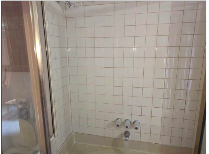
Overview of Plumbing Fixture(s) in Operation.
