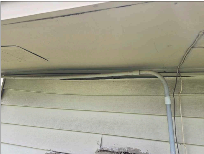
There is loose siding on the home, recommend securing all loose siding to help prevent damaged and water penetration. Mainly at - rear
