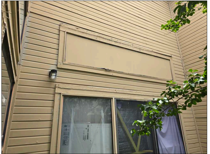
Deterioration was noted at the siding, recommend replacing all deteriorated siding to help prevent further deterioration and water penetration. Unable to determine the condition of the underlying materials. Mainly at - left
