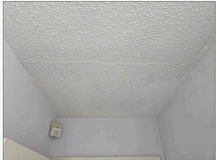
Settlement cracks were noted in the drywall. These are generally considered cosmetic only, unless otherwise noted. Mainly at - right rear bedroom
