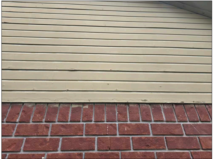
Deterioration was noted at the siding, recommend replacing all deteriorated siding to help prevent further deterioration and water penetration. Unable to determine the condition of the underlying materials. Mainly at - left
