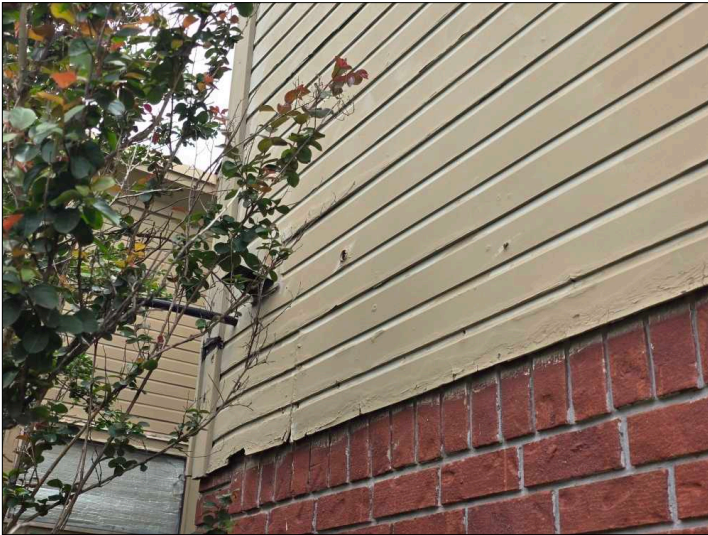
Deterioration was noted at the siding, recommend replacing all deteriorated siding to help prevent further deterioration and water penetration. Unable to determine the condition of the underlying materials. Mainly at - left
