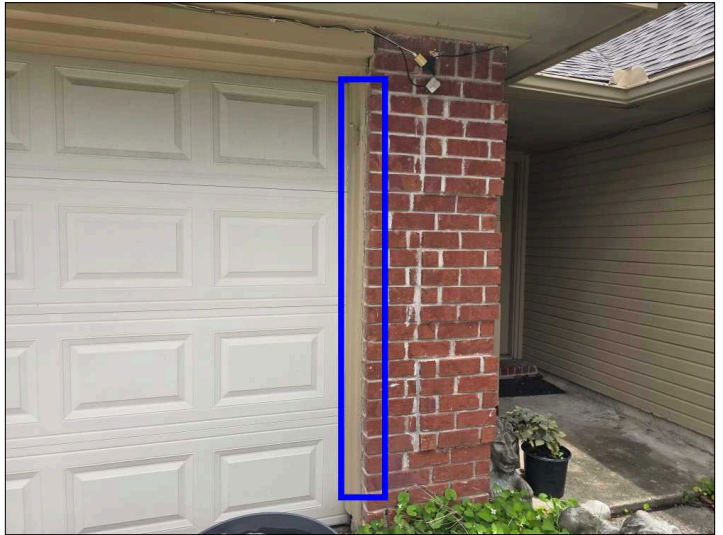
Recommend sealing between the trim and brickwork to help prevent water penetration. Mainly at - front
