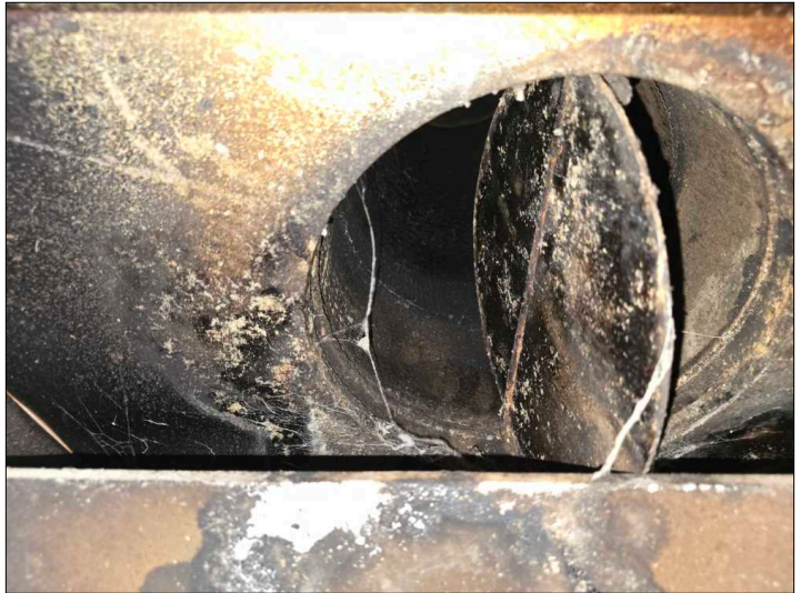
The fireplace damper is missing a damper clamp to ensure proper ventilation for the gas logs, recommend adding damper clamp to help prevent damper from closing.
