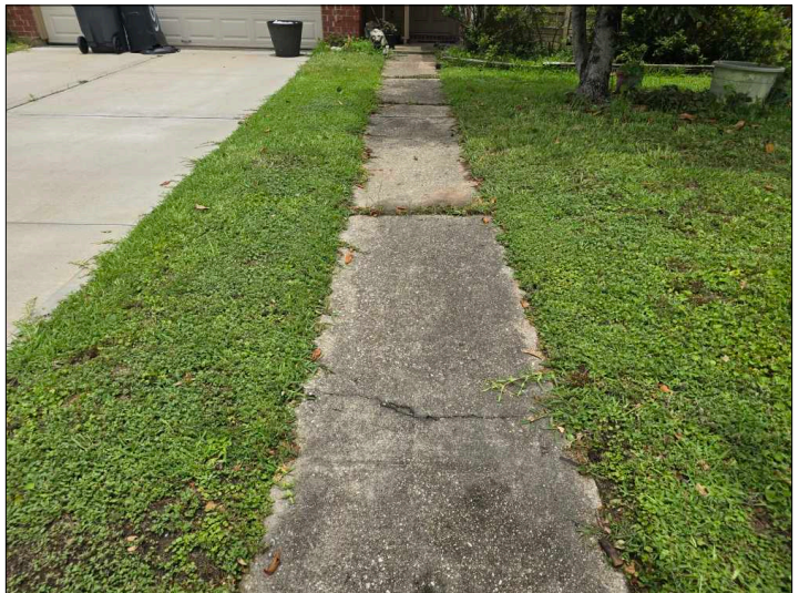
Cracks were noted in the pavement. These are cosmetic in nature at this time. Recommend sealing to help prevent further deterioration. Mainly at - sidewalk
