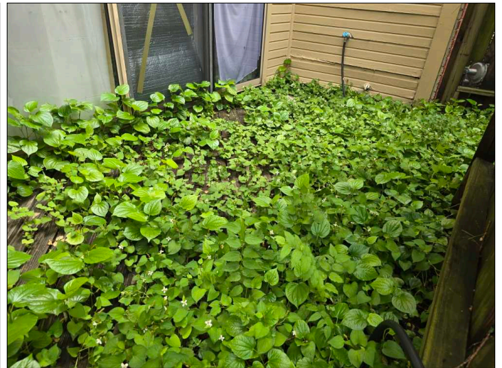
Recommend trimming vegetation so that it is not in contact with the house. Vegetation in contact with the structure can hold moisture against the structure and promote damage to building materials and conducive conditions for wood destroying insects.
