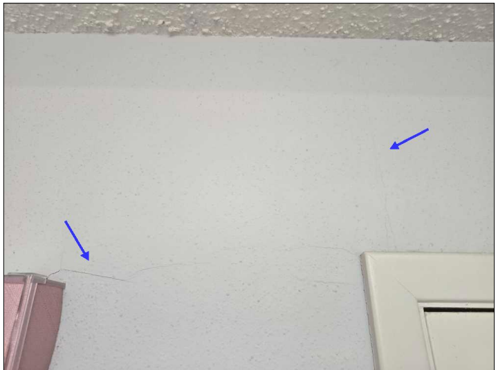
Settlement cracks were noted in the drywall. Mainly at - right rear bedroom
