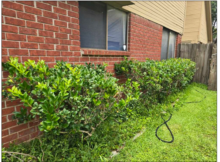
Recommend trimming vegetation so that it is not in contact with the house. Vegetation in contact with the structure can hold moisture against the structure and promote damage to building materials and conducive conditions for wood destroying insects.
