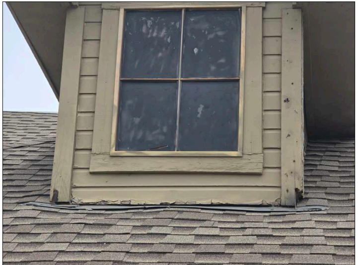
There is some damage to the exterior trim, recommend repairs to help prevent water penetration. Unable to determine the condition of the underlying materials. Mainly at - front
