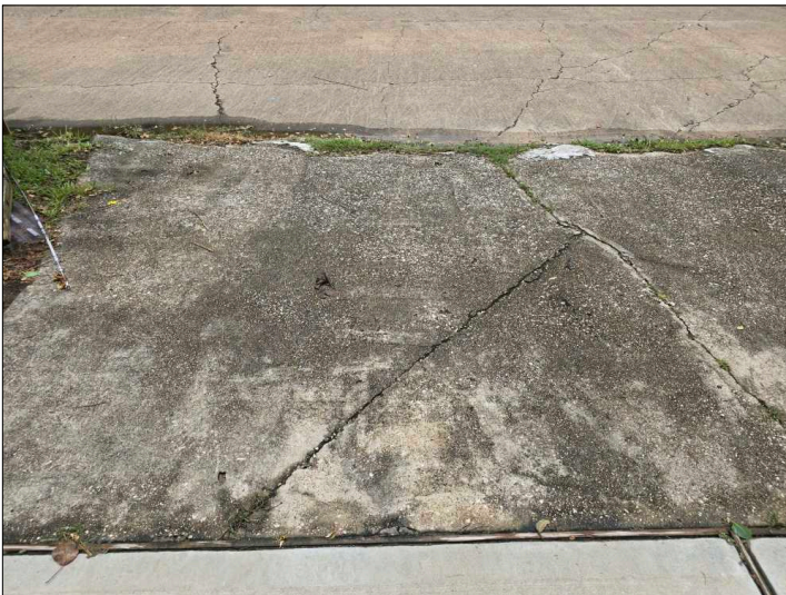
Cracks were noted in the pavement. These are cosmetic in nature at this time. Recommend sealing to help prevent further deterioration. Mainly at - driveway
