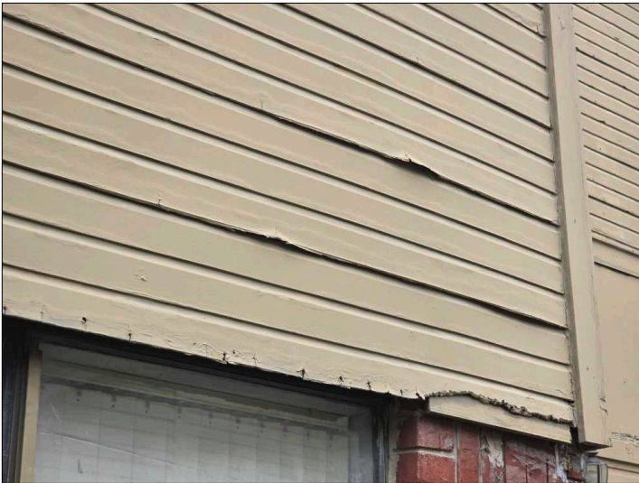
Deterioration was noted at the siding, recommend replacing all deteriorated siding to help prevent further deterioration and water penetration. Unable to determine the condition of the underlying materials. Mainly at - right
