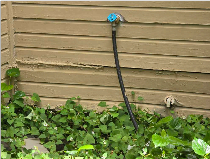
There is some damage to the exterior siding, recommend repair or replacement to help prevent water penetration. Unable to determine the condition of the underlying materials. Mainly at - left
