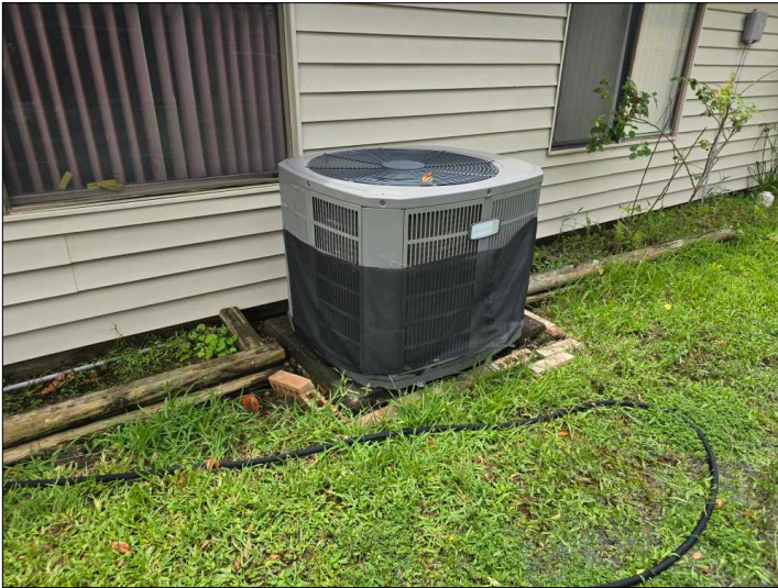
Overview of A/C Condenser
