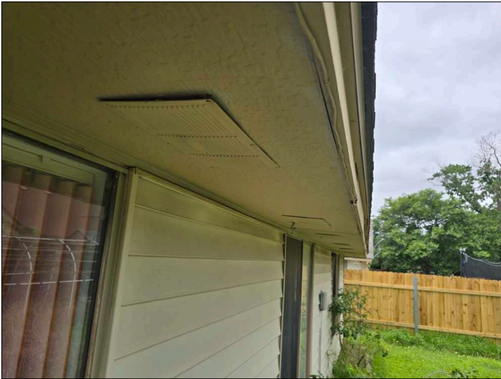
The attic vent screen is loose, damaged or missing, recommend repairs to help prevent unwanted entry.
