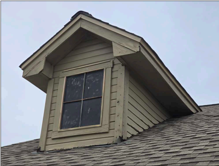
Deterioration was noted at the siding, recommend replacing all deteriorated siding to help prevent further deterioration and water penetration. Unable to determine the condition of the underlying materials. Mainly at - front
