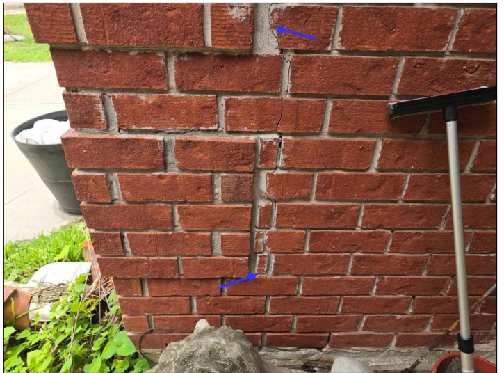
Settlement cracks were noted in the brickwork. Mainly at - front
