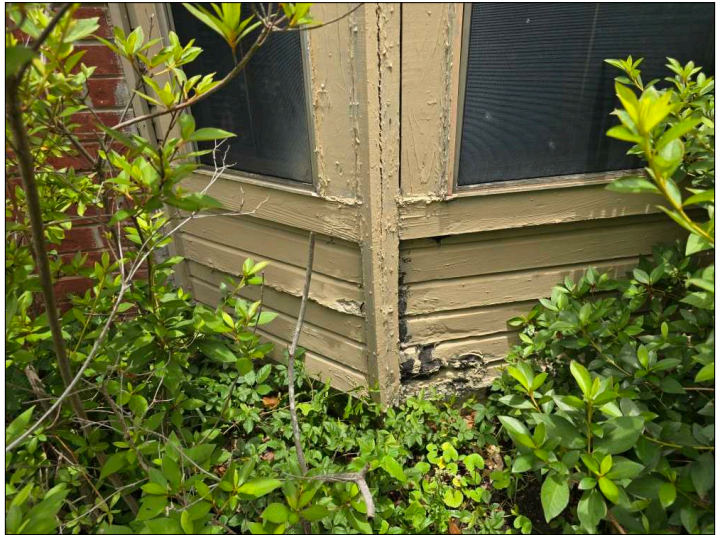
Deterioration was noted at the siding, recommend replacing all deteriorated siding to help prevent further deterioration and water penetration. Unable to determine the condition of the underlying materials. Mainly at - front
