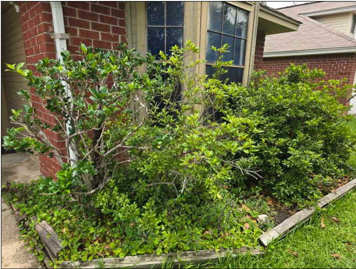
Recommend trimming vegetation so that it is not in contact with the house. Vegetation in contact with the structure can hold moisture against the structure and promote damage to building materials and conducive conditions for wood destroying insects.
