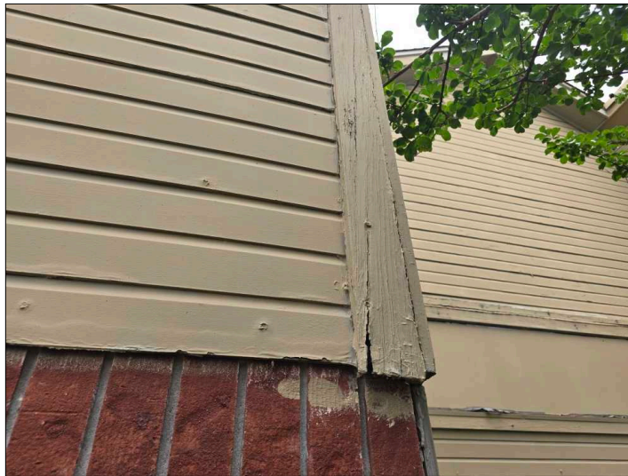
Deterioration was noted at the trim, recommend replacing all deteriorated trim. Unable to determine the condition of the underlying materials. Mainly at - left
