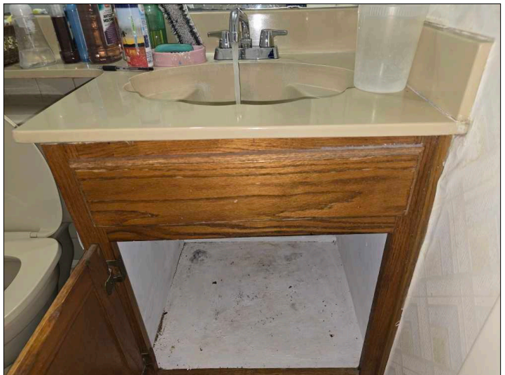
Overview of Plumbing Fixture(s) in Operation.
