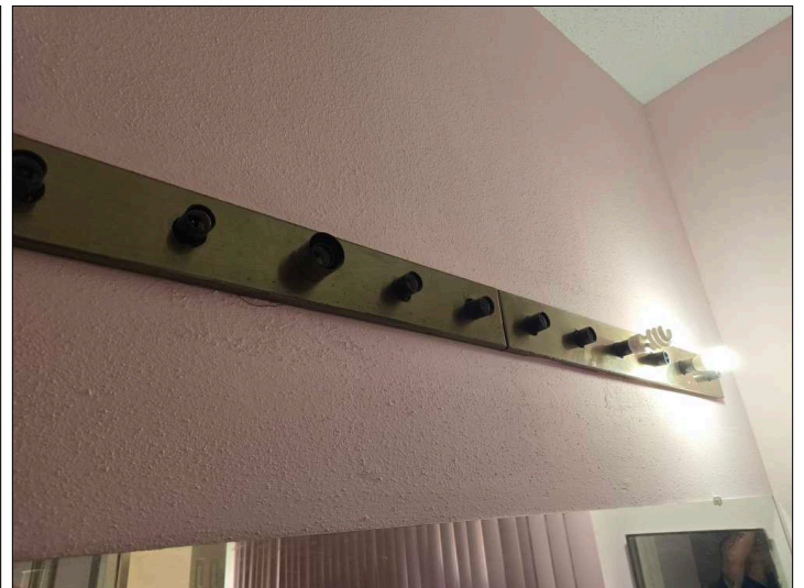
Some bulbs in the light fixture(s) were noted to be missing. Recommend replacing or installing bulb(s) to verify fixture is operating correctly. Some fixture may be on motion or photo cells and are not tested during the inspection. Mainly at - primary bathroom
