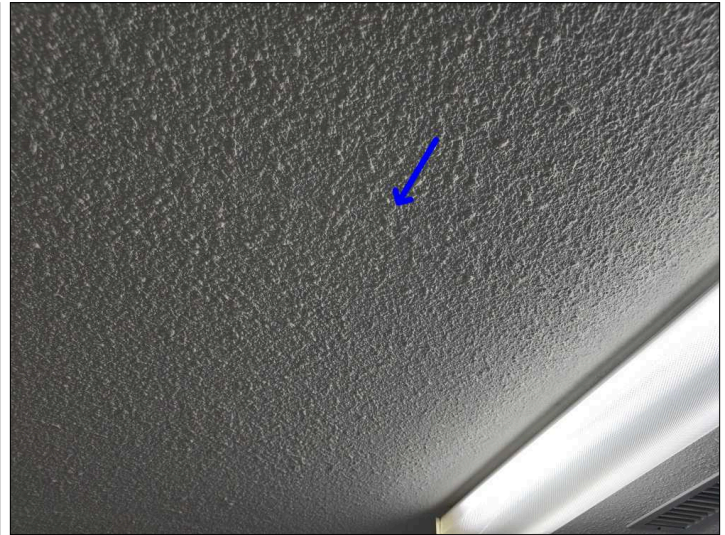
Settlement cracks were noted at the tape joint in the drywall. Mainly at - kitchen
