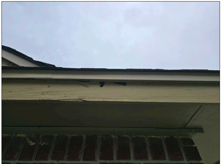
Deterioration was noted at the trim, recommend replacing all deteriorated trim. Unable to determine the condition of the underlying materials. Mainly at - left
