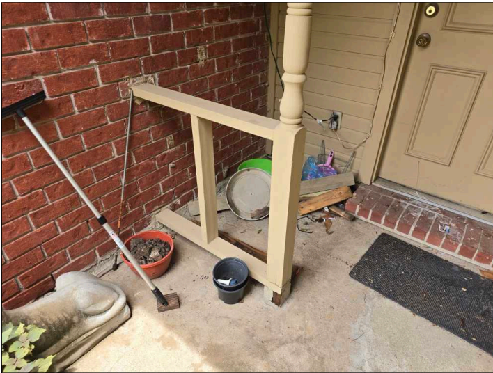
The porch post are showing signs of deterioration, recommend repairs or replacement to prevent further deterioration.
