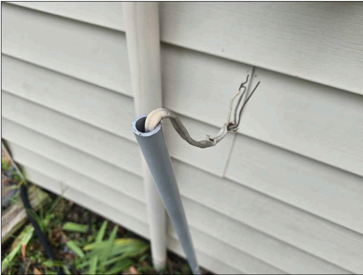
There are visible unprotected wiring splices. Recommend the wiring be properly enclosed. Mainly at - rear
