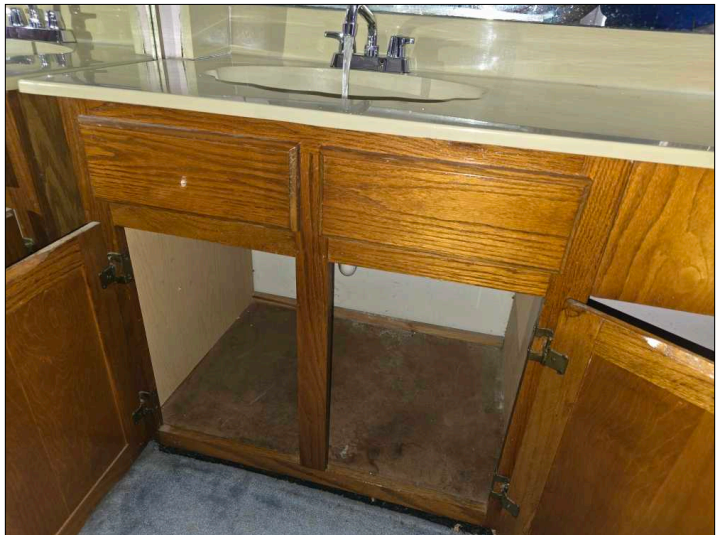
Overview of Plumbing Fixture(s) in Operation.
