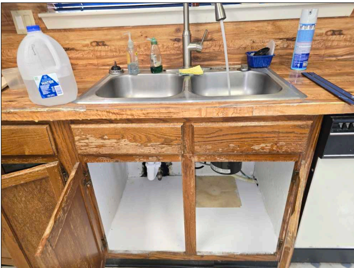
Overview of Plumbing Fixture(s) in Operation.
