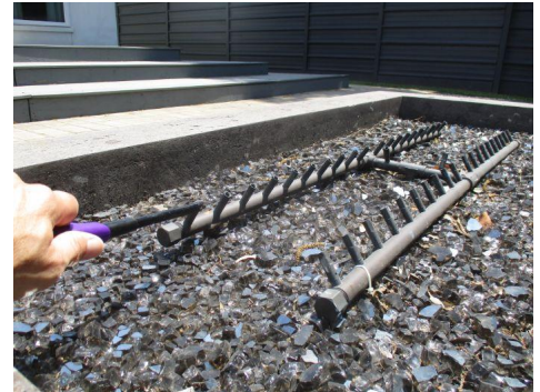
No gas observed
