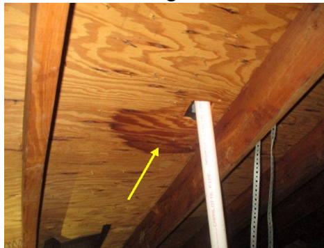
Water stains at South DWV
