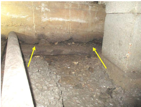
Gaps under grade beam
