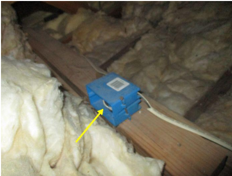
Junction boxes missing covers above living room
