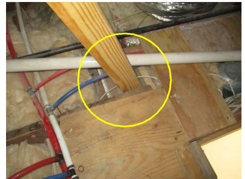
Observed improper installation of bracing from roof rafters down to ceiling joists.
