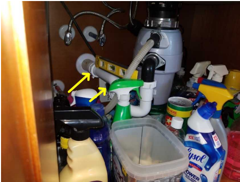
Reverse slope of drain line. kitchen sink.
