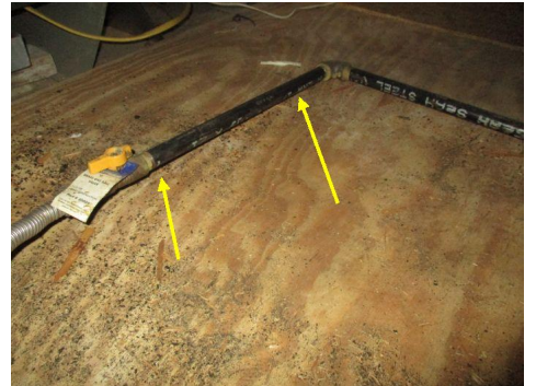
Gas line near furnace is not supported/ or secured to decking
