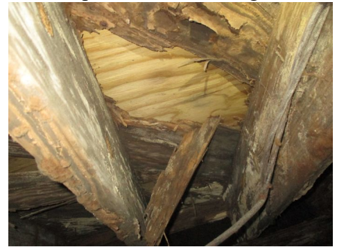
Damaged/ repaired sub floor at multiple locations
