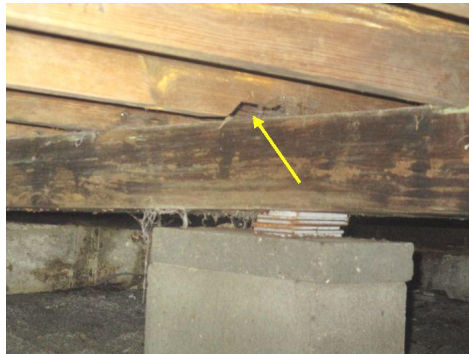
Joist not in contact with beam under living area
