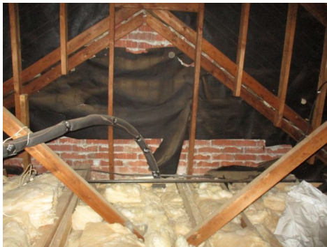
Observed damaged paper vapor barrier in attic.
