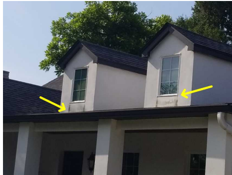
Stains on stucco surfaces
