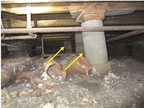
Piers leaning under center of home
