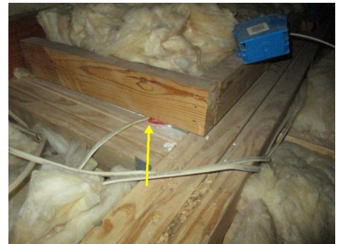
Framing in attic improperly installed on top of electrical wiring above living room/ hallway in attic.
