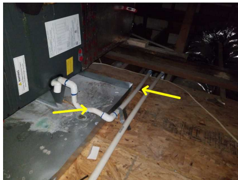
Primary drain line is missing insulation; West unit
