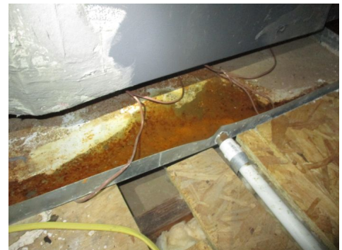
The secondary drain pan contains water, correct existing conditions; East unit.
