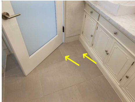
Cracked tiles at master bath
