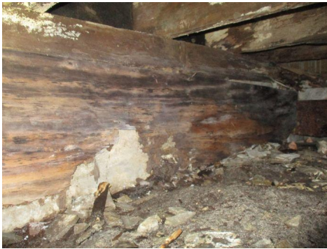
Form board/ wood to ground contact at multiple locations
