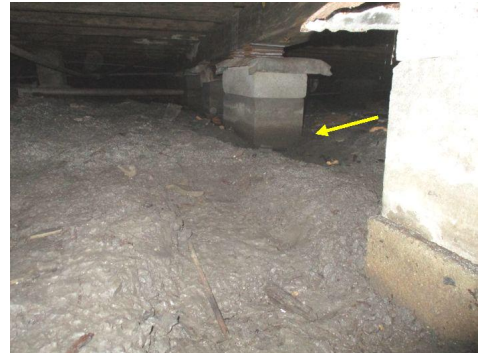
Ground is very soft in areas, water stains at piers
