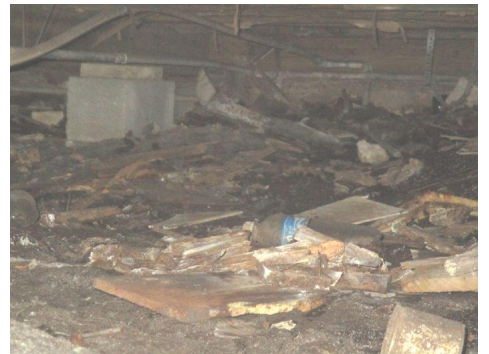
Scrap wood/ debris/ junk below home should be removed
