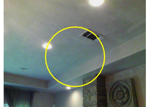
Missing insulation at living room
