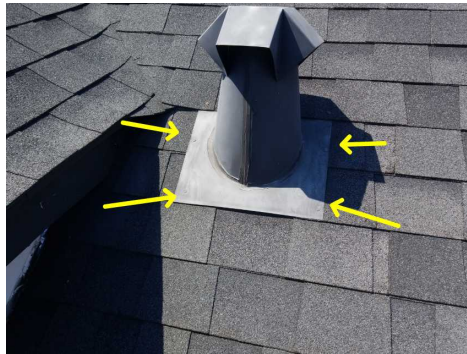
Exposed nail heads and not shingle fashion
