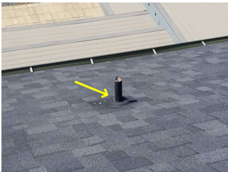
Rubber boot flashing inverted at South exterior
