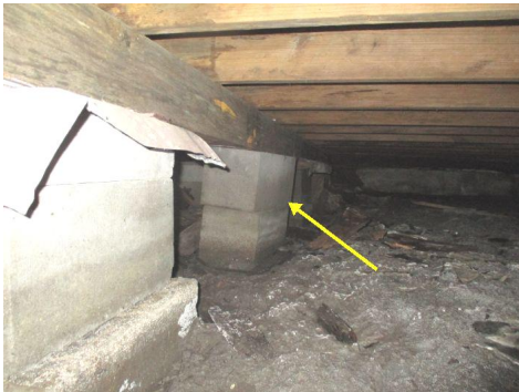
Pier leaning Northwest
