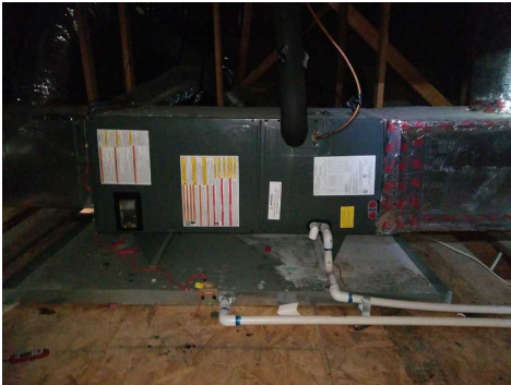
West Electric Unit
