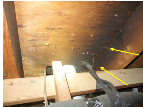
Discolored wood in attic indicates improper venting of the gas-fired furnace and recognized fire hazard,
