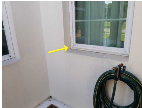
Window frame is cracked/ damaged; North exterior.
