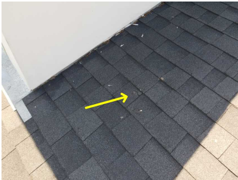
Scuffed/ damaged shingles at front dormer
