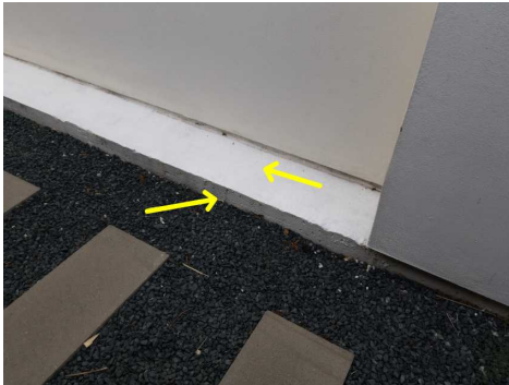
Small crack at West exterior
