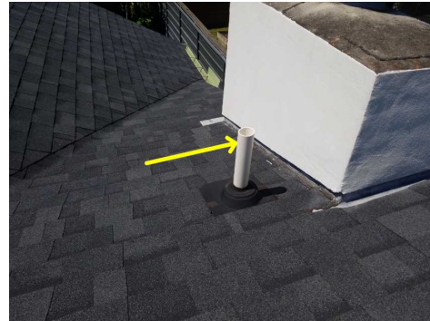
Painting of exterior plastic PVC vents above the roof line required to prevent UV damage.
