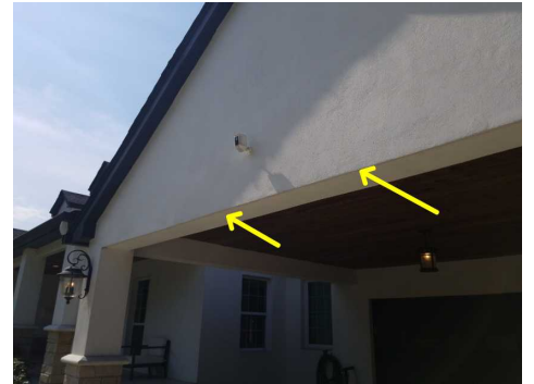
Weep screed holes are blocked/ sealed over.
