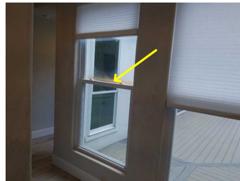
West hallway window lost seal
