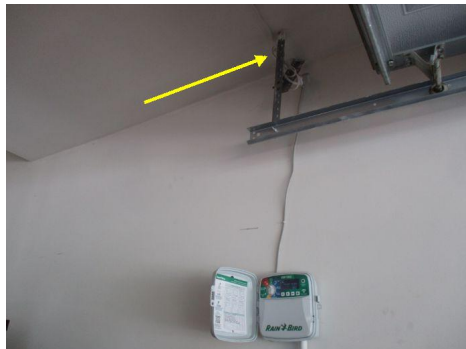
Extension cord wiring for irrigation controller
