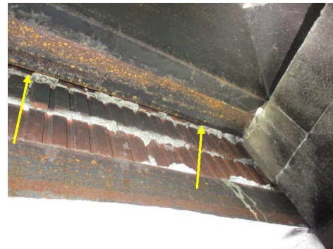
Hearth not sealed properly around the perimeter of damper and/or on the interior backside of the lintel
