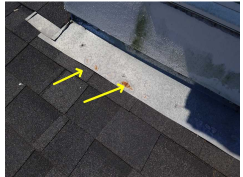
Rusted flashing at front dormers
