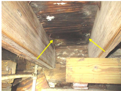
Sub floor appears wet under front exterior/ porch
