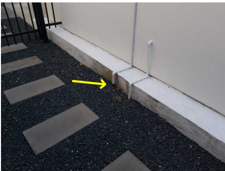
Primary drains near foundation
