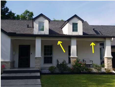
Header sagging or leaning, at front porch
