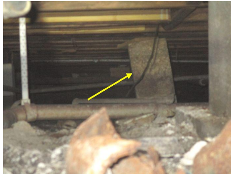
Pier leaning West
