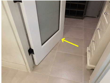
Master closet door will not open/ close, in contact with floor
