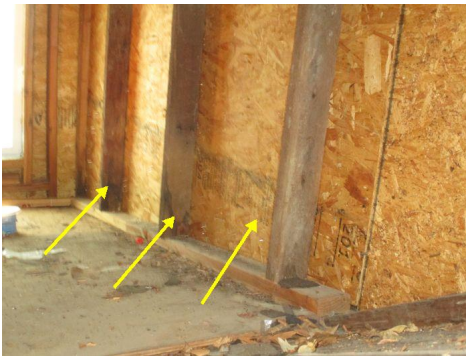
Water stains at front dormers
