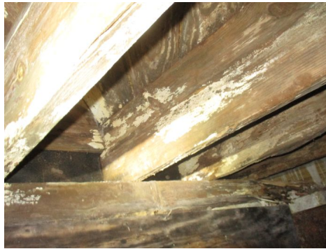
Wood rot/fungus on various wood members in crawlspace observed below the house.
