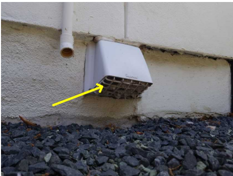
Dryer vent is clogged and has a screen
