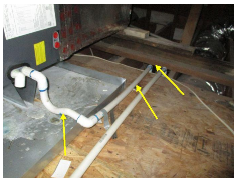
Primary drain line missing insulation; West unit
