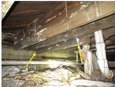
Joists under guest bath need repair
