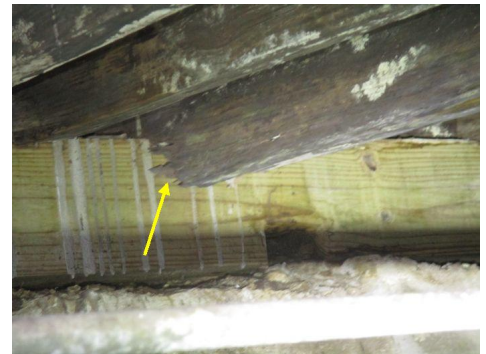
Damaged joists below guest bathroom
