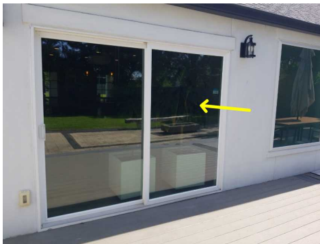
Sliding door system lost its seal
