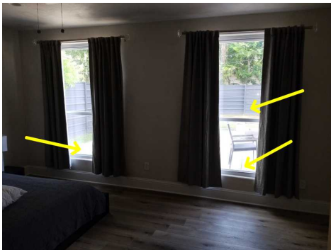
East bedroom windows lost their seals
