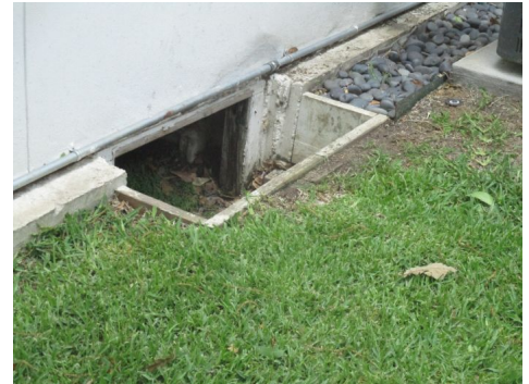
Crawlspace access missing a door
