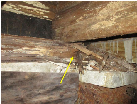
Southeast corner needs further evaluation/ repair
