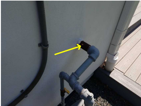
Exposed exterior gas piping not protected from corrosion
