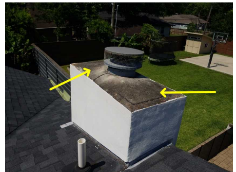
Missing cap flashing at chimney
