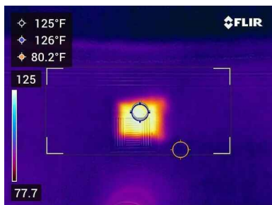
Area #1 Temperature at Register
