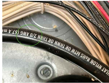
2/0 AWG Copper Service Entrance Conductors
