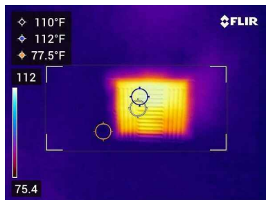
Area #1 Temperature at Register
