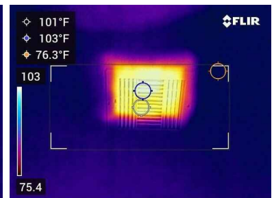
Area #1 Temperature at Register
