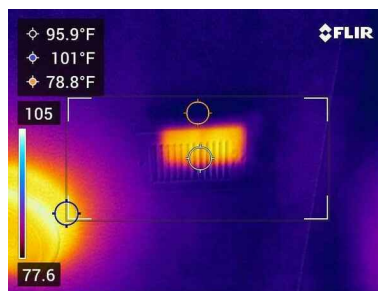
Area #1 Temperature at Register
