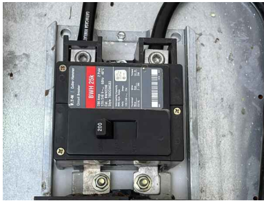
200 amp main breaker
