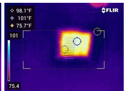
Area #1 Temperature at Register
