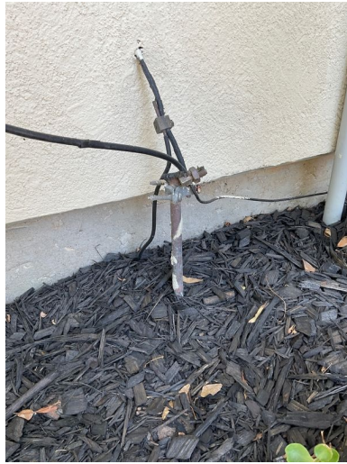
Electric Subpanel Location: Garage
