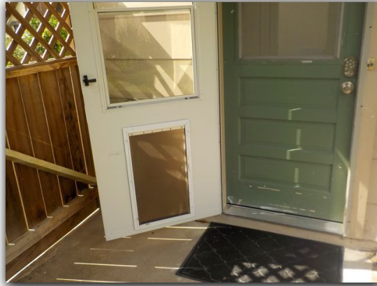
The upstairs right front room closet doors need maintenance.
