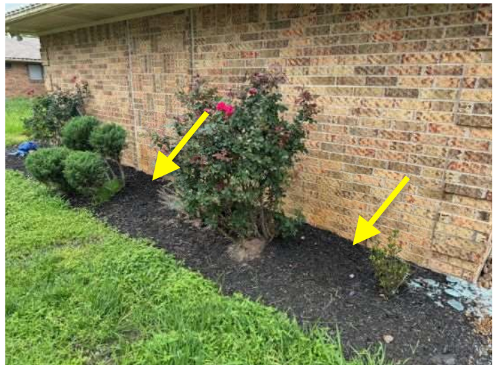
High soil level observed - Front- Foundation not visible
