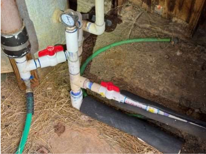
Water main shutoff for the house
