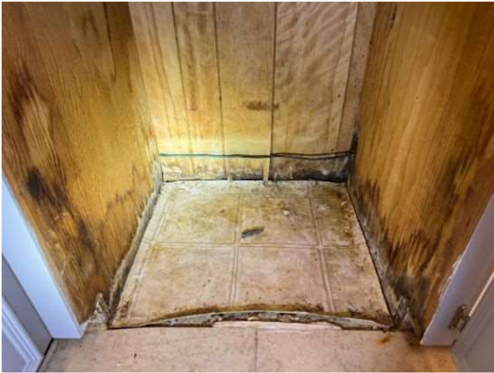
Kitchen cabinet deteriorating under sink
