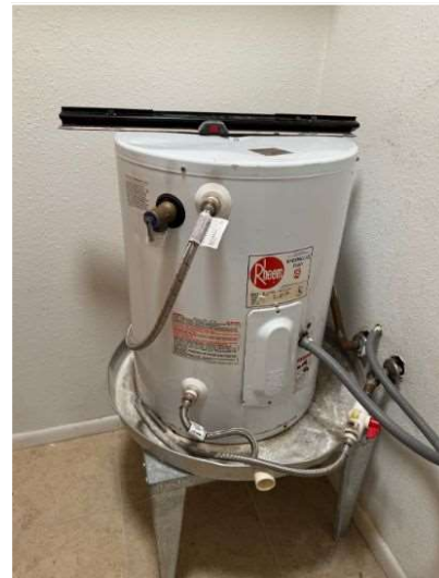
Water heater not installed as per standards
