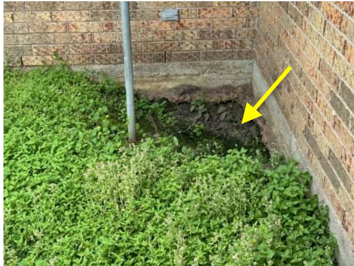
Water ponding observed - Rear
