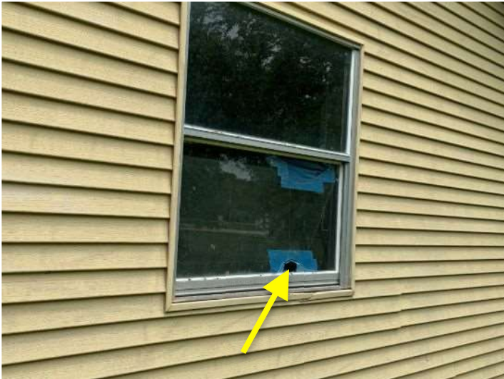
Glass insert cracked - replace it
