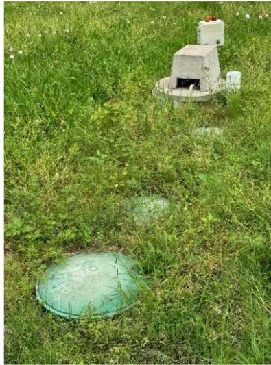
Plumbing main cleanout - septic system
