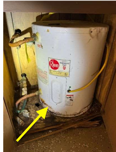
Water heater rusted / damaged / Leak - Not operational - Patio area
