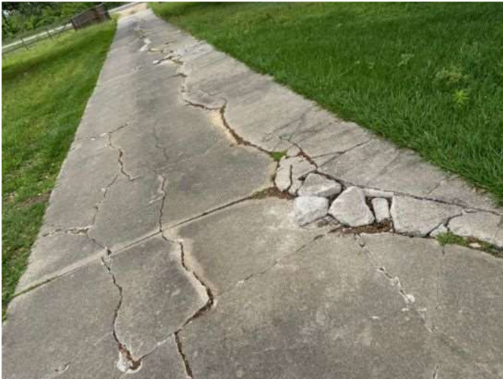
Cracks on driveway - Uneven
