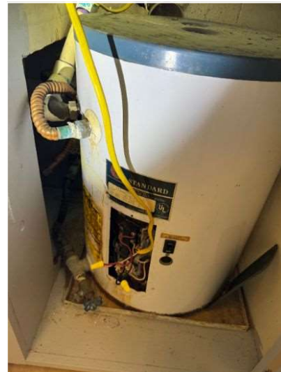
Water heater not installed as per standards - Laundry room
