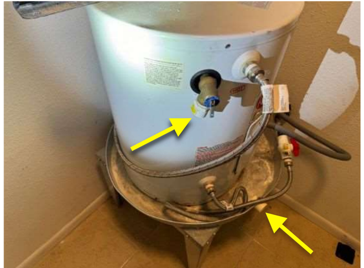
Safety valve not extended outside
