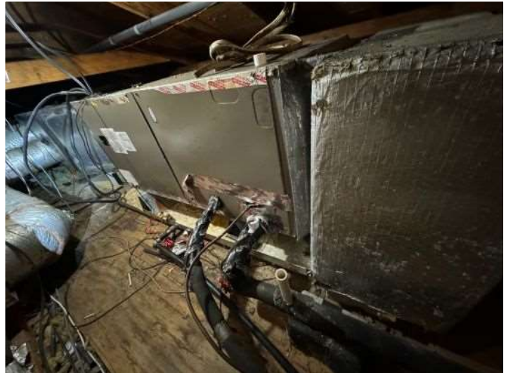
Furnace installed as per standards
