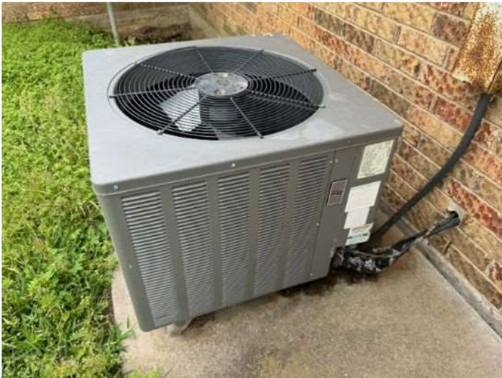
AC compressor installed as per standards
