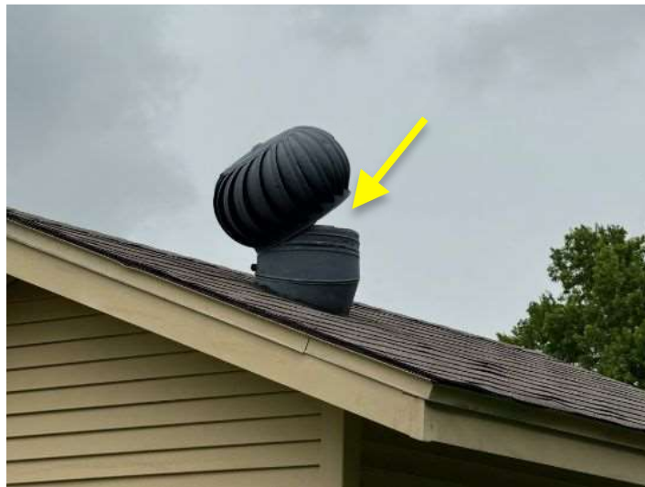
Roof vent separated - opened - Water well area
