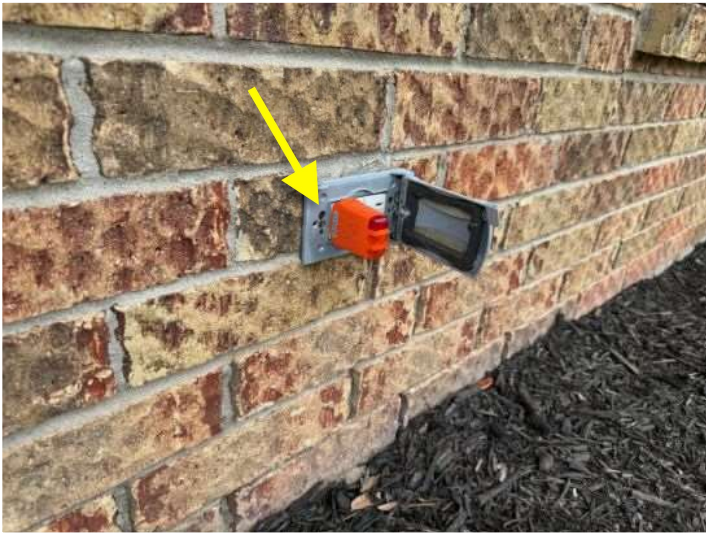
No power to receptacle - front
