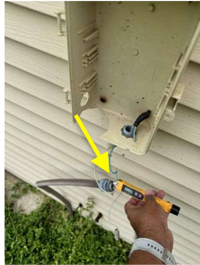
Open splices - Exposed hot wires - rear of the house
