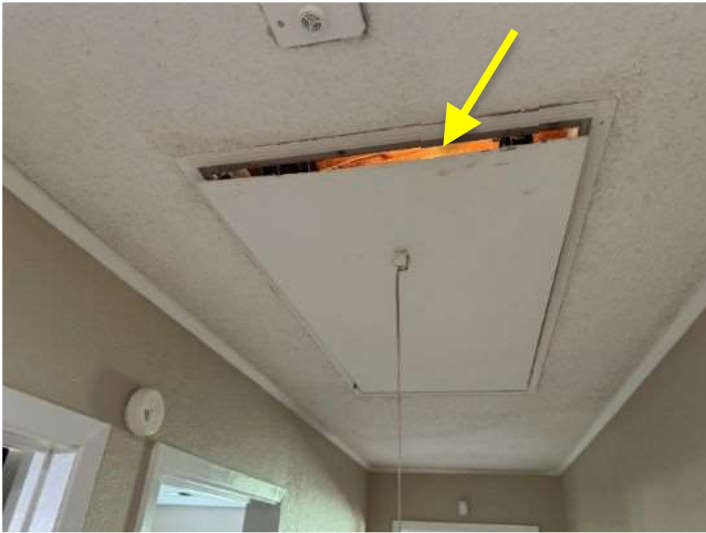
Attic door does not close securely - gapp observed
