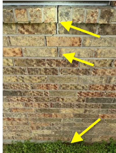
Crack on foundation slab and bricks above - Rear - further evaluation recommended
