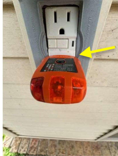
No GFCI (Ground fault circuit interpreter) installed - Rear
