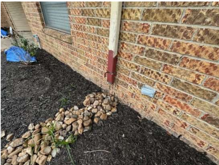
Splash guard not installed -Front - rain water will splash close to foundation slab
