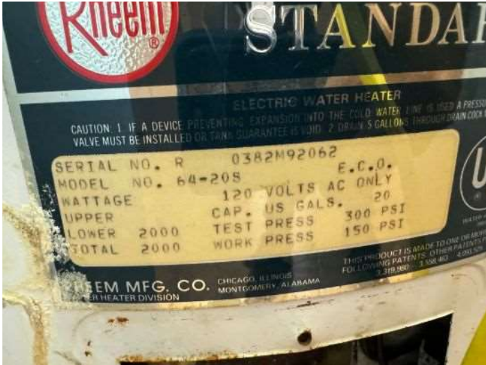
Data info - water heater 20gallons.
