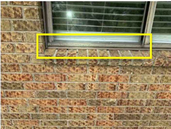
Window frame needs caulking and sealing
