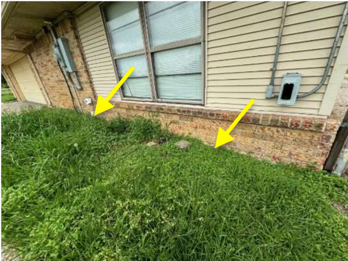
High soil level observed - Right side of the house- Foundation not visible
