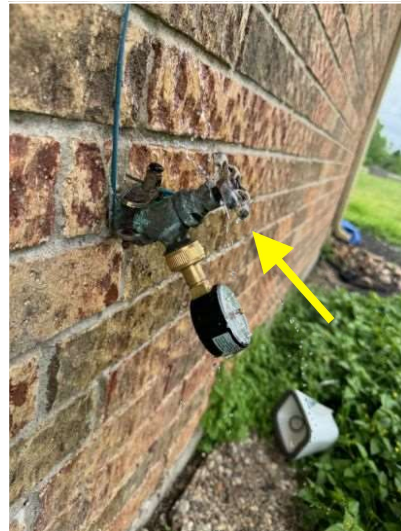
Faucet leaks Left side of the house
