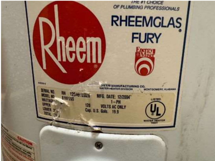
Data info - water heater 19.9 gallons.
