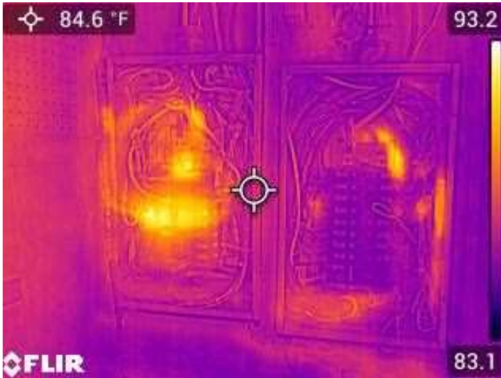
Branch circuit - Copper wiring observed
