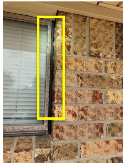
Window frame needs caulking and sealing Rear
