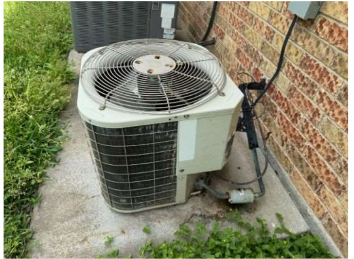
AC compressor installed as per standards
