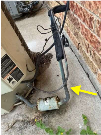
Insulation needs to be replaced
