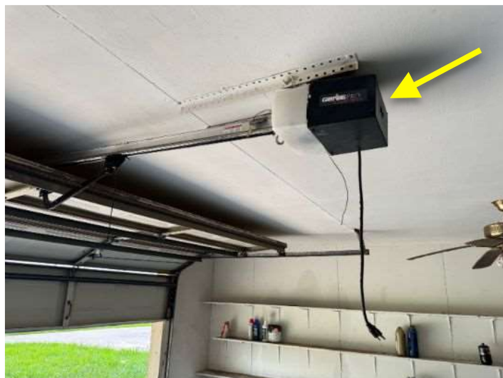
Garage door operator not operational - Unplugged
