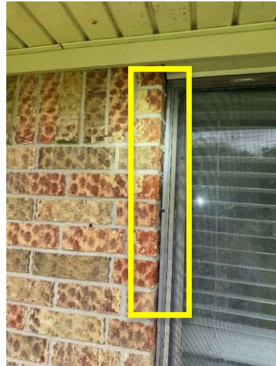
Window frame needs caulking and sealing Left side of the house
