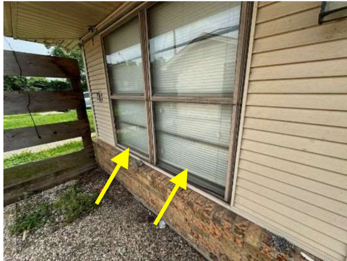
Window screen not installed first level bedroom
