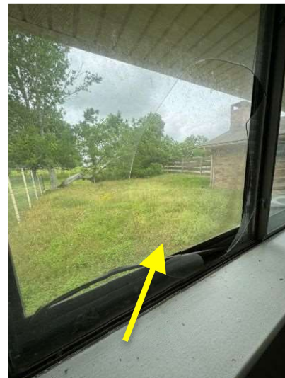
Glass insert cracked - first level bedroomreplace it
