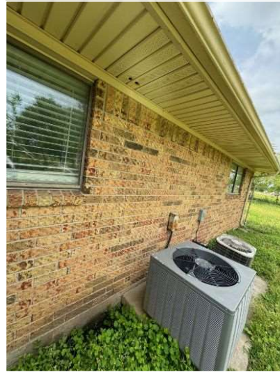
Condensation water dripping line not extended out from soffit area
