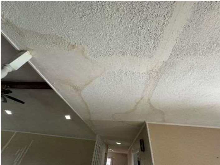
Water stains/ marks observed - Living
