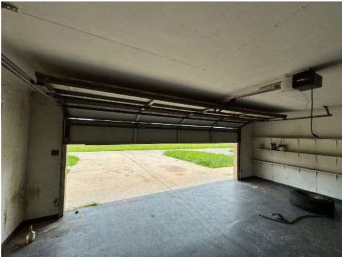
Garage door manually operational.
