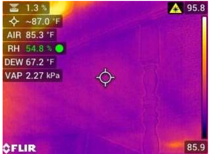
Thermal imaging - Active moisture from attic to ceiling sheet-rock in Living area
