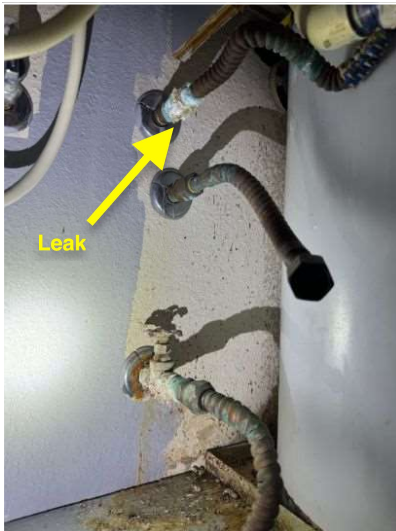
Corrosion and leak found around the hot line valve from water heater
