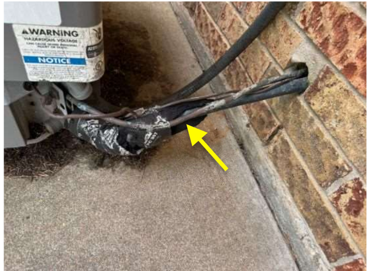
Insulation needs to be replaced
