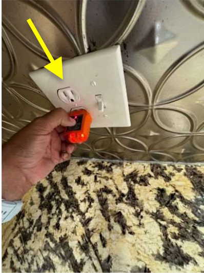
No GFCI (Ground fault circuit interpreter) installed - Kitchen
