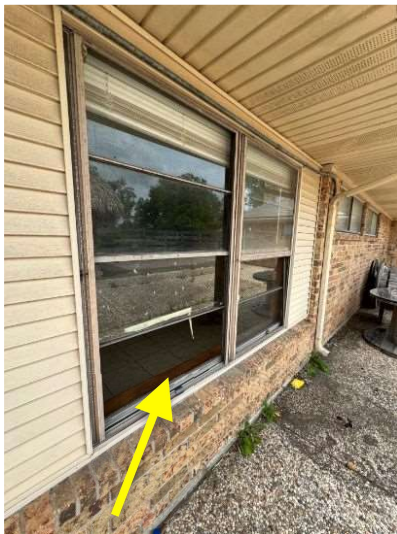
Glass insert cracked - replace it
