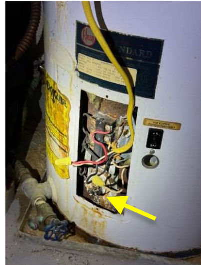
Water heater rusted - water dripping from tank - Laundry area water heater
