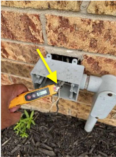
Open splices - Exposed hot wires - front of the house
