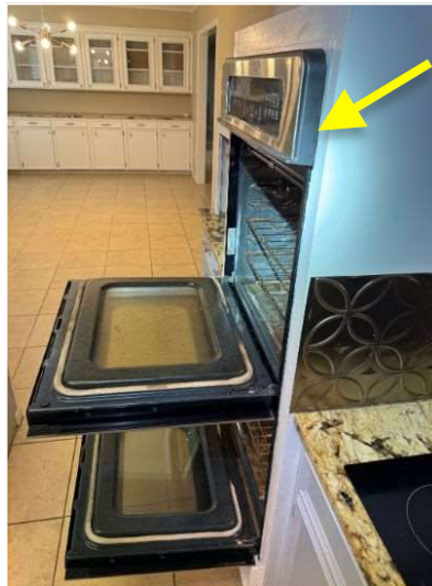
Oven not screwed with cabinet - Loose
