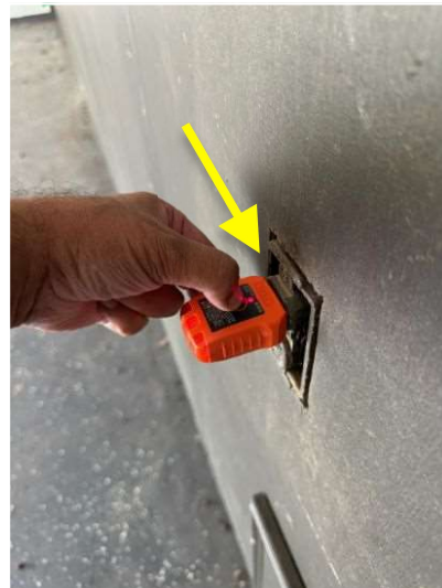
No GFCI (Ground fault circuit interpreter) installed - garage
