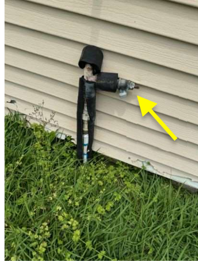
Faucet damage - Right of the house
