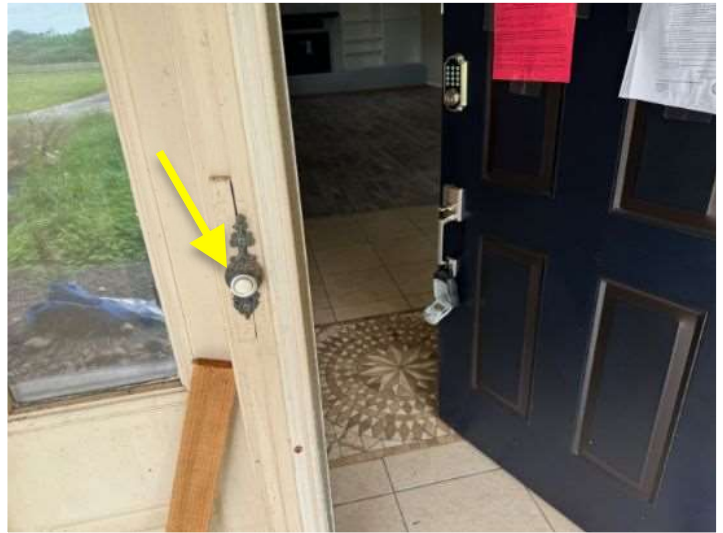
Door bell does not work
