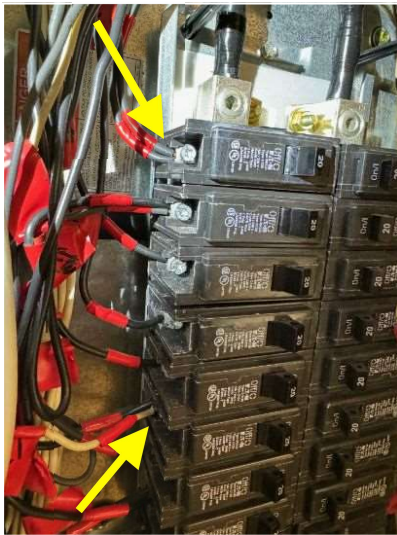
Double tapping on breakers
