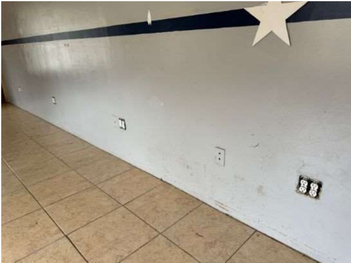
Missing / damaged outlet cover multiple
