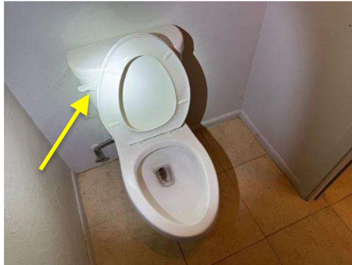
Toilet seat water tank not operational
