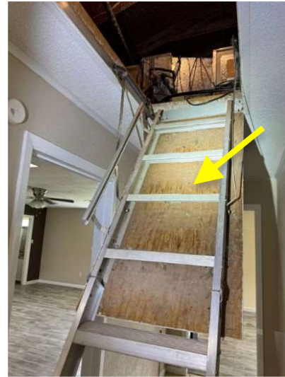
No fire resistant insulation installed on attic opening door
