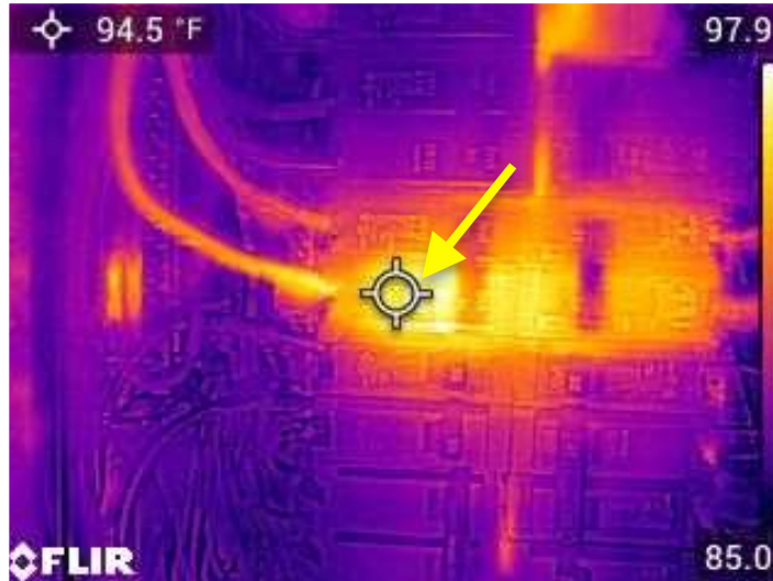
Ac breaker loose and sparking - Recommended licensed electrician
