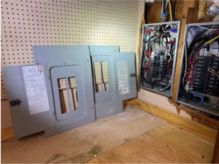
Electrical panel cover not installed and breakers not labeled.
