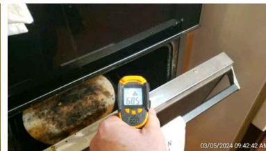
Lower Oven Inoperative
