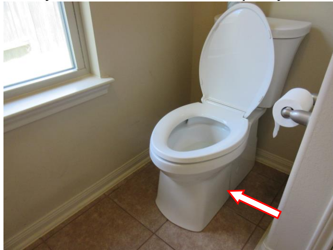
Hallway full bathroom: toilet isn't adequately secured
