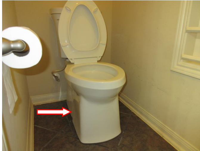
Master bathroom: toilet isn't adequately secured
